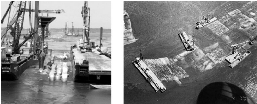
Figure 4.16 Typical moments of construction at Airbus site Hamburg, overview (Alexiew and Raithel, 2015)
