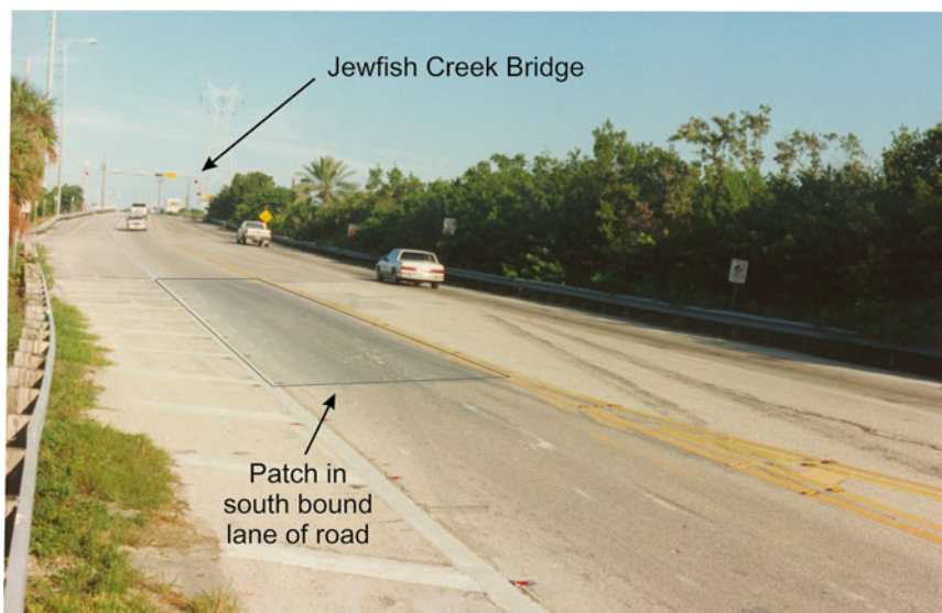
Fig. 26.2 A patch about 15 m long was noted in the southbound lane of US-1. The Jewfish Creek lift bridge is seen in the top of the photograph. The view is towards the northwest
