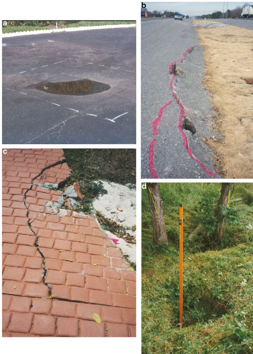
Fig. 15.10 Early subsidence is commonly indicated by the presence of circular depressions that retain water (a), cracks, fractures or local settlement in the soil (b), cracks in asphalt or concrete driveways (c) and localized depressions or drop-outs (d)
