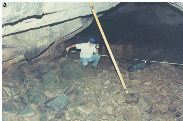
Cave discovered during site walkover in Virginia
