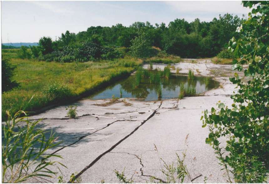
Fig. 25.23 Evidence of surface subsidence up to 2 m is seen in the paved parking lots of the two medical office buildings that were built over the easternmost extent of the Tobin Mine
