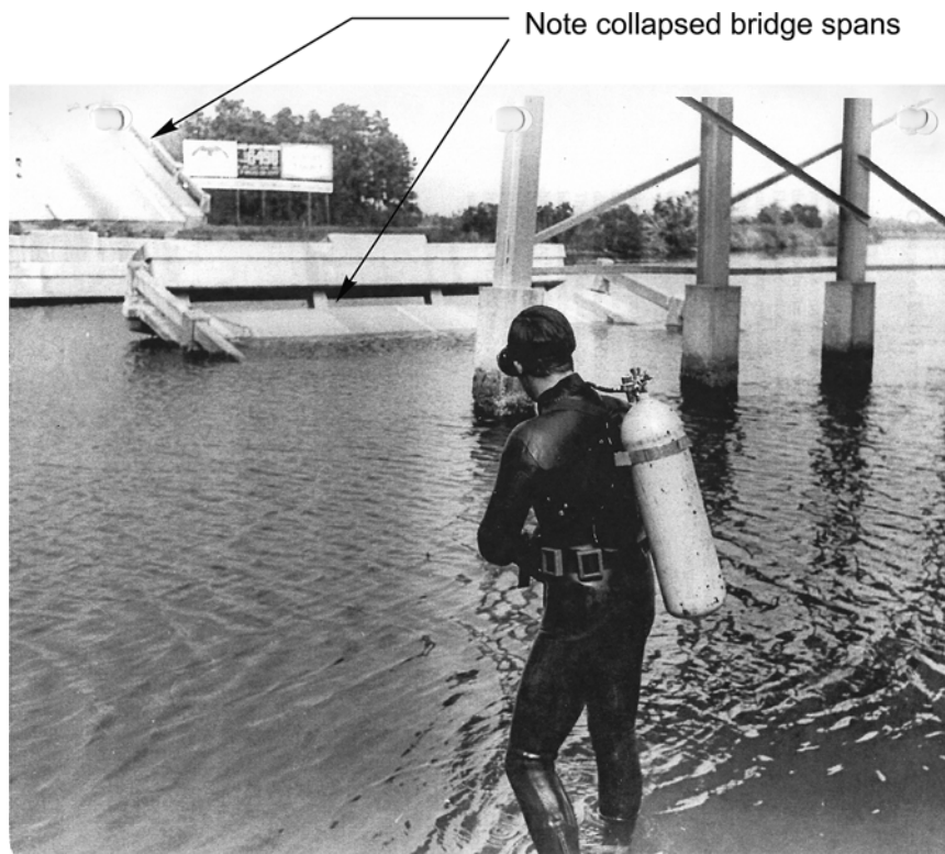
Fig. 19.2 A geologist prepares to make a dive to inspect conditions of a bridge collapse (Photo courtesy of Paul Beam)
