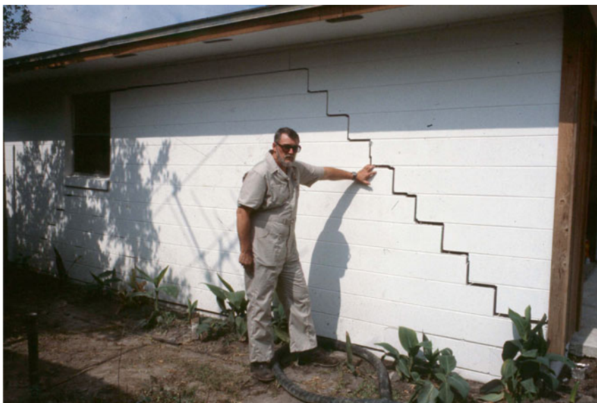
Fig. 7.1 In some cases the structure may be impacted by settlement resulting in cracks
