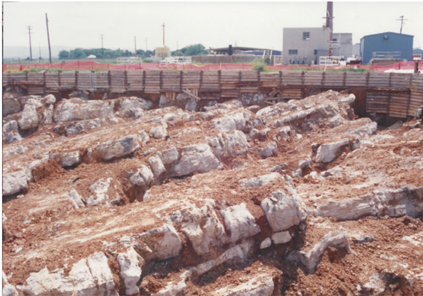
Fig. 17.23 An excavation clearly shows the complex nature of the top of limestone
