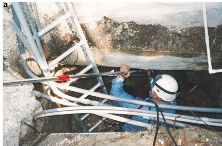
a Downhole video camera mounted on pole being extended into collapse beneath home
