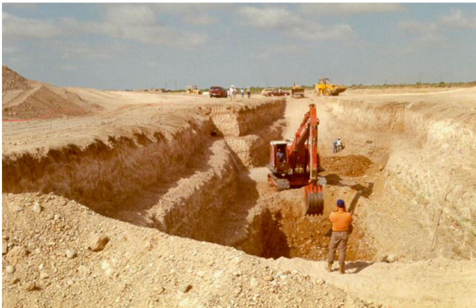
Fig. 17.24 A large trench is being excavated to expose the top of rock and assess possible buried channel or paleokarst conditions
