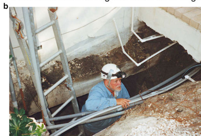
Inspection of collapse reveals cave under house along east coast of Florida
