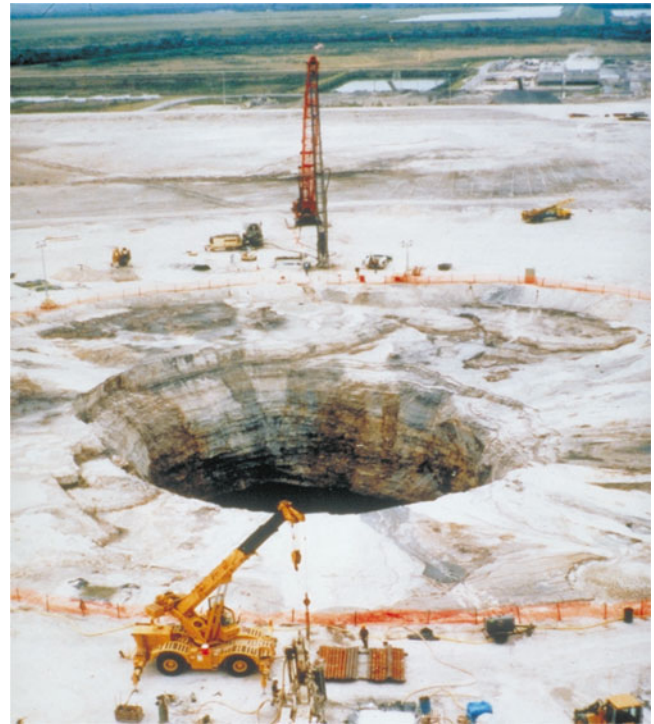
Fig. 7.8 A large sinkhole developed in a gypstack, a waste material from the phosphate industry in Florida (Tihansky 1999)
