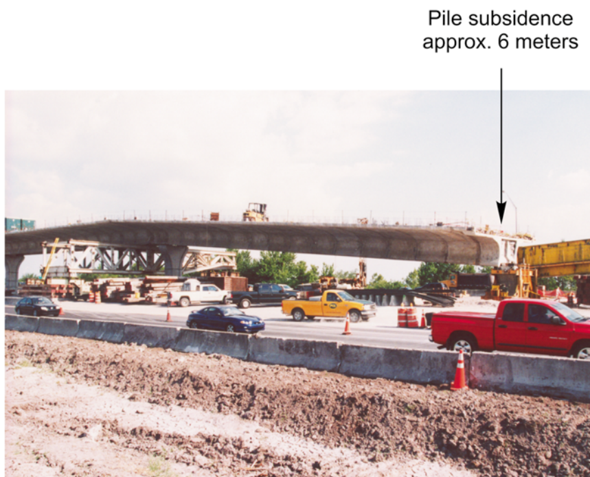
Fig. 7.6 Damage occurred during construction of the Crosstown Expressway in Tampa, Florida when one pile slowly sunk about 6 m
