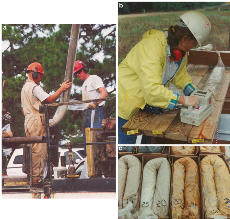
Fig. 17.12 A sediment sample from a roto sonic drill rig is being placed into a plastic sleeve (a), which is then monitored for radioactivity (b). The core is then labeled and stored (c)
