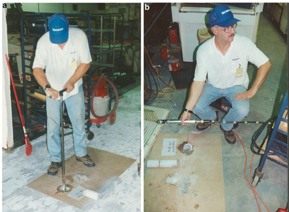
Fig. 17.19 A cored borehole was cut through the concrete floor of an electroplating plant to assess suspected voids under the floor and acquire samples (a). A borehole video camera was used to assess the extent of the void under the floor (b)
