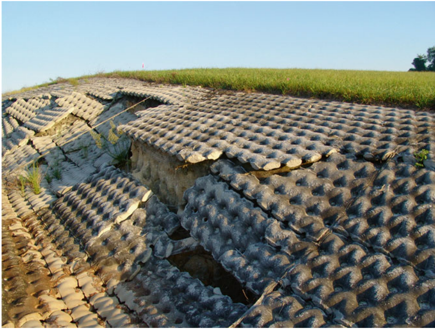
Fig. 7.2 Seepage of water through a concrete lining used to transfer surface water away from a landfill resulted in washing away of sediment and ultimately the collapse of the lining
