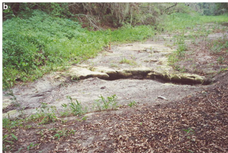
open fracture found in dry creekbed
