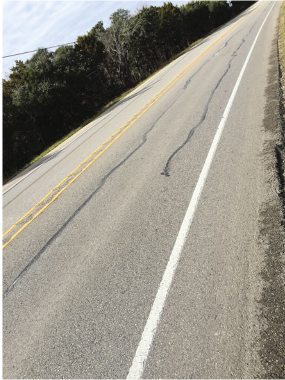
Fig. 8.4 Typical fatigue cracks on a pavement section along the wheel path (Photograph by A Bhasin)
