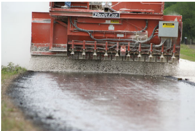
Fig. 3.8 Single-sized aggregates being sprayed on a pavement surface coated with asphalt emulsion (Photograph by A Bhasin)
