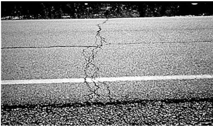
Fig. 1.21 Photograph of thermal cracking. (Source Road Science, a Division of ArrMaz)
