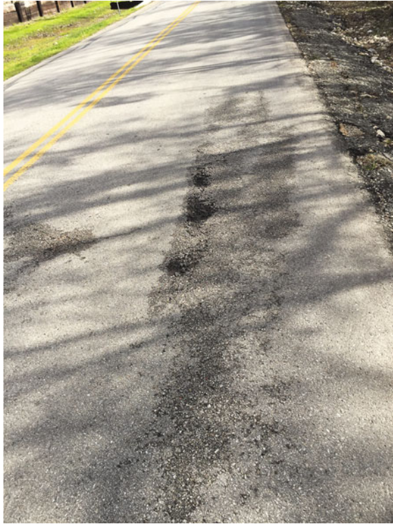
Fig. 8.8 Typical example of a pavement section with severe moisture induced damage (Photograph by A Bhasin)
