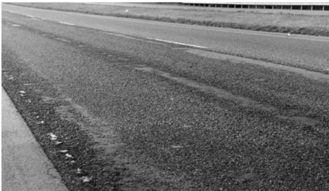
Fig. 1.22 Photograph of raveling. (Source Road Science, a Division of ArrMaz)
