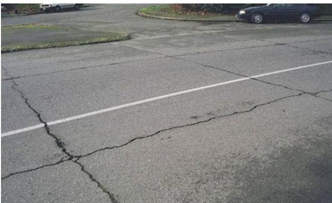
Fig. 1.20 Photograph of reflective cracking. (Source Road Science, a Division of ArrMaz)
