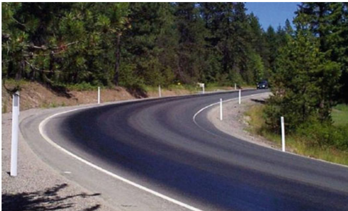
Fig. 1.17 Photograph of bleeding. (Source Road Science, a Division of ArrMaz)
