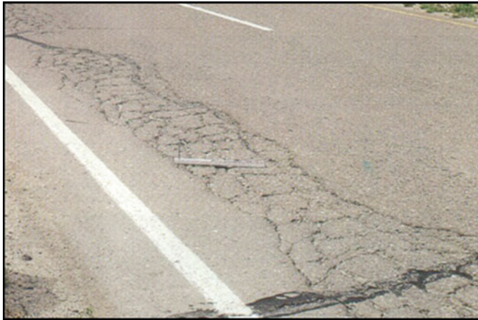
Fig. 15.45 Photograph showing typical alligator cracking along wheel path within the roadway (Source Road Science, a Division of ArrMaz)
