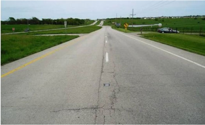
Fig. 1.18 Longitudinal cracking. (Source Road Science, a Division of ArrMaz)
