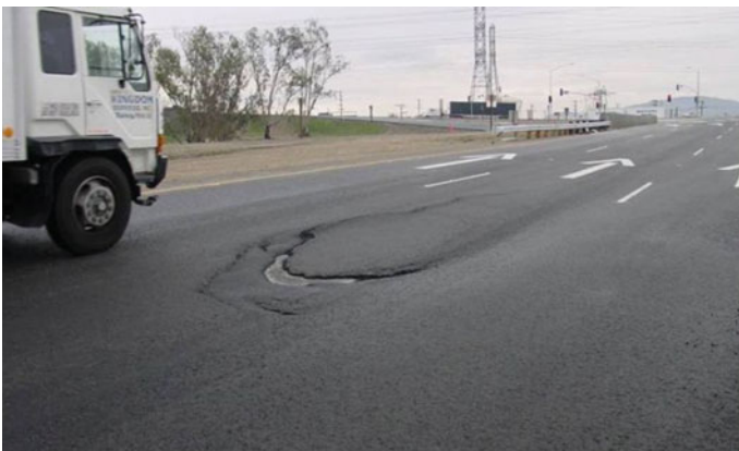
Fig. 1.19 Photograph of pushing accompanied by delamination. (Source Road Science, a Division of ArrMaz)
