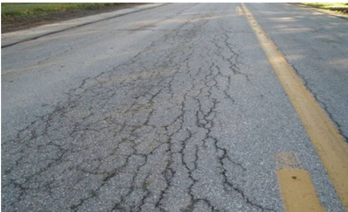
Fig. 1.15 Photograph of fatigue cracking. (Source Road Science, a Division of ArrMaz)
