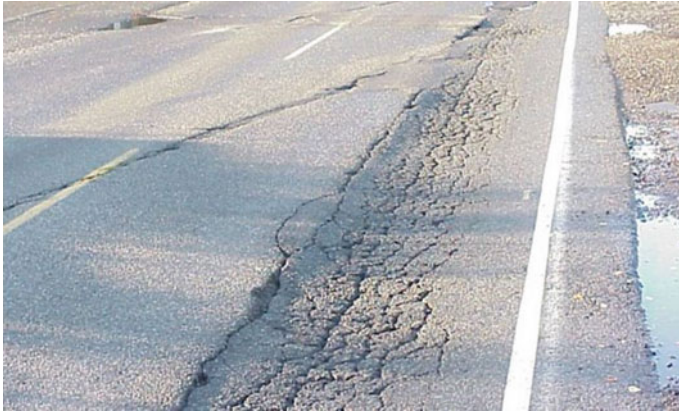
Fig. 1.25 Photograph of rutting accompanied by alligator cracking. (Source Road Science, a Division of ArrMaz)
