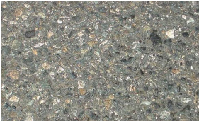
Fig. 1.26 Photograph of surface wear resulting in aggregate polishing. (Source Road Science, a Division of ArrMaz)
