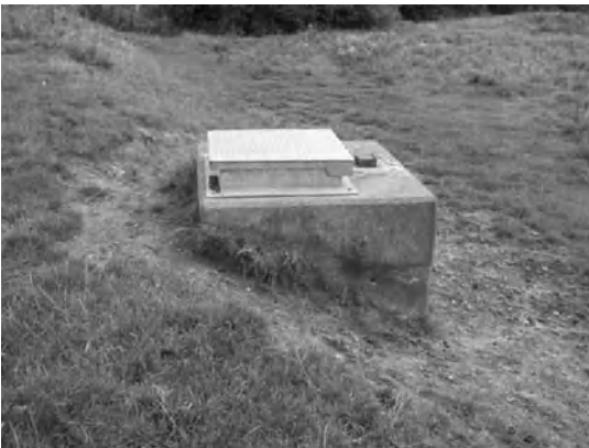
Fig. 6.11 Foreign object presence causing erosion in slope.
