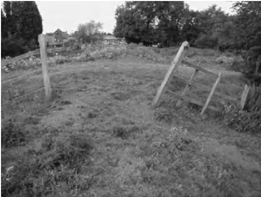
Fig. 6.10 Rutting of slope and crest caused by livestock.
