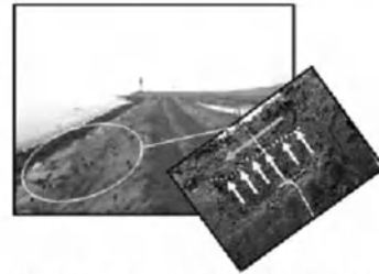
Fine fissuring - FRMRC WP 4.1 Mark Dyer
