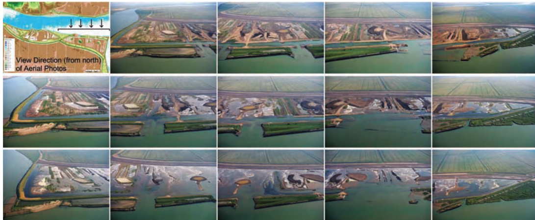
Fig. 4.3 Initial flooding of the first scheme on the Wallasea site, where the design made use of the existing field drains.
