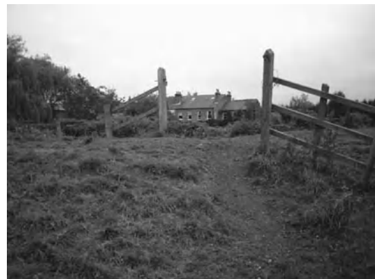
Fig. 6.9 Rutting of embankment crest and slope caused by third party (livestock).
