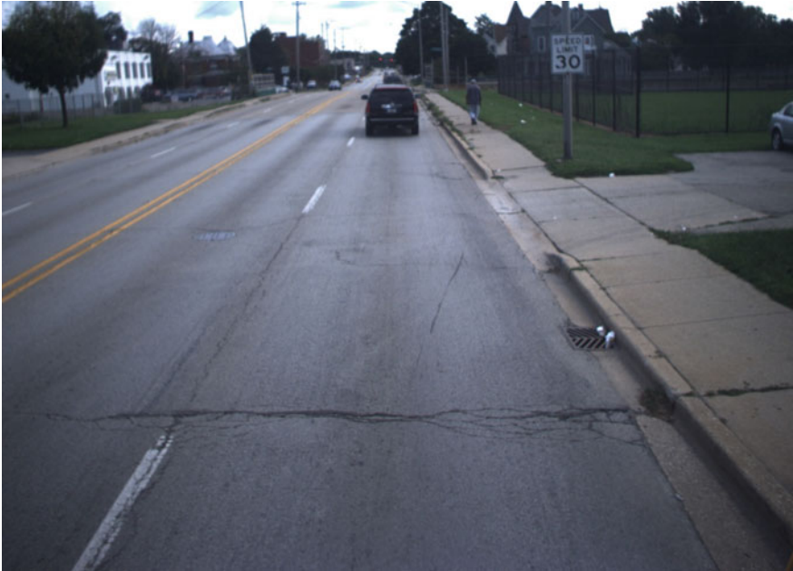
Fig. 1.4 Reflective cracking in asphalt pavement in Chicago, Illinois. Photo W. Buttlar
