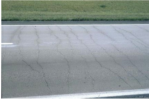
Fig. 4.46 Thermal cracking in asphalt pavement
