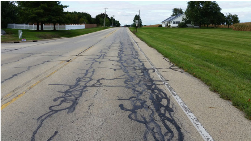
Fig. 1.3 Fatigue cracking in asphalt pavement in Savoy, Illinois. Photo W. Buttlar
