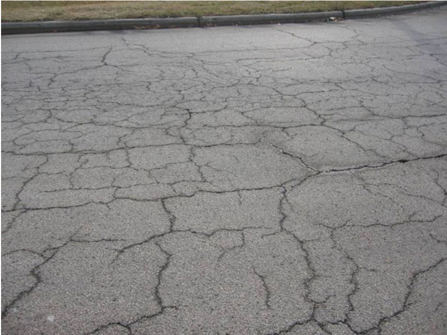
Fig. 1.6 Block cracking in asphalt pavement in Urbana, Illinois. Photo W. Buttlar
