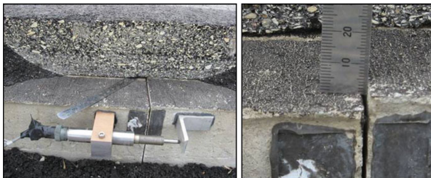
Fig. 1.23 Section-3 slab faulting and intact overlay system
