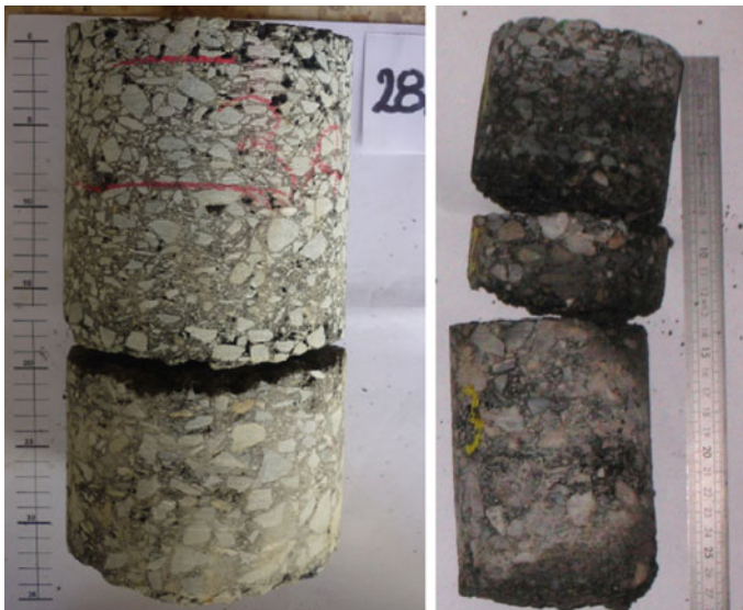
Fig. 1.1 Examples of cores from thick bituminous pavements, showing debonding of surface or internal layers
