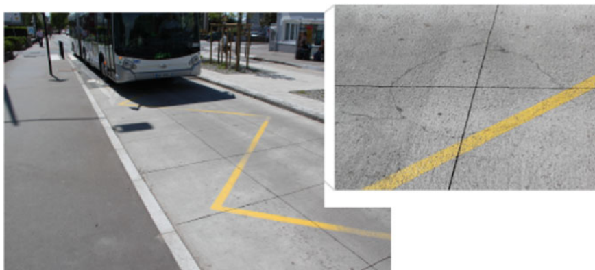
Fig. 1.8 Corner crack of UTW in Nantes, France. Photo A. Chabot
