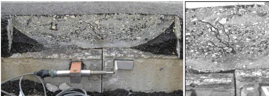
Fig. 1.22 Section-2 crack jumping and slab faulting
