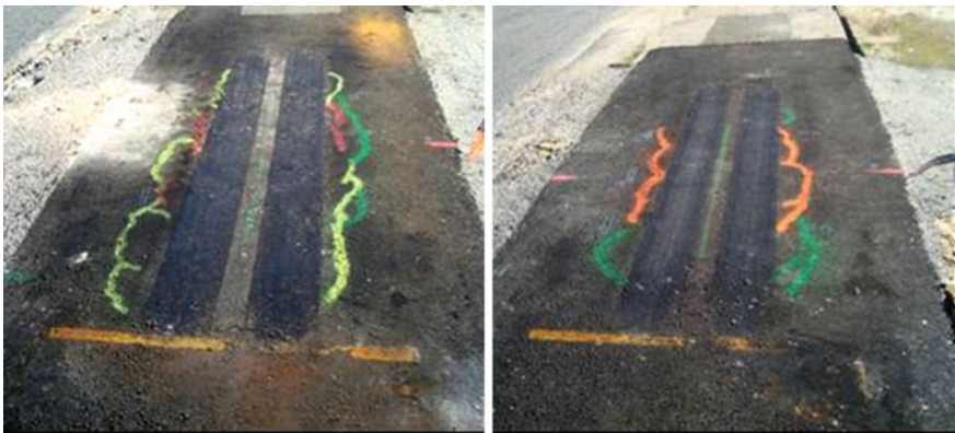
Fig. 1.19 Final condition of structure P2 with Tri-Ax grid (left) and section P4 with AR-G grid (right) [39]
