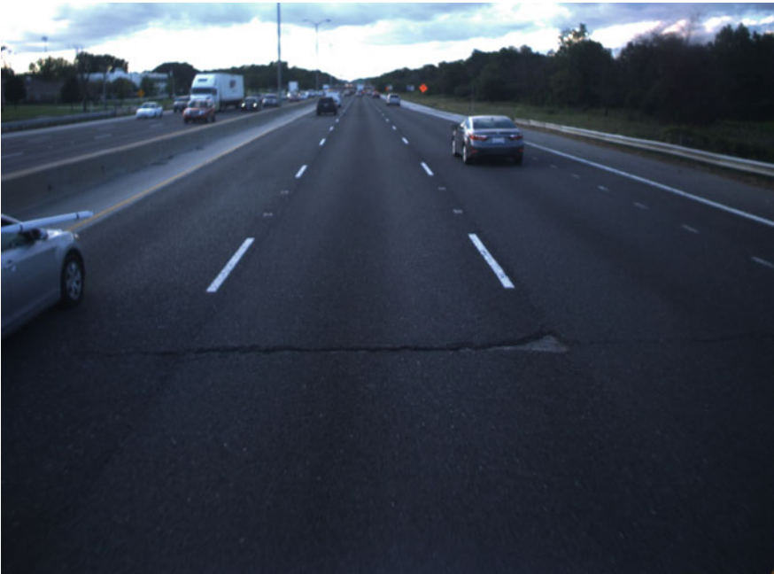
Fig. 1.5 Debonding in asphalt pavement in Chicago, Illinois. Photo W. Buttlar
