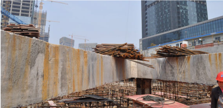
Fig. 10.2 Inappropriate storage of rebar at Project B
