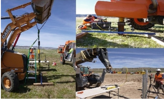
Fig. 2. Photos of pile load testing (left: uplift, upper right: compression, lower right: lateral. Courtesy of RRC power & energy, LLC)
