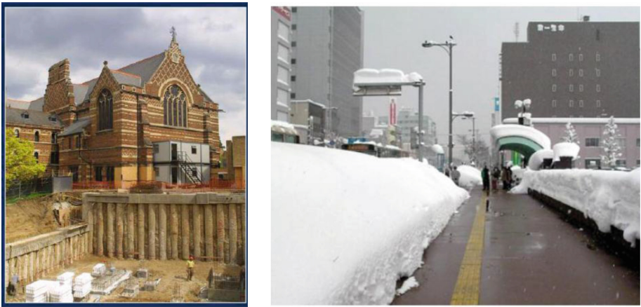
Fig. 1. Implementation of Energy Piles in: Left) Keble College, UK. and, Right) a Walk Road in Japan
