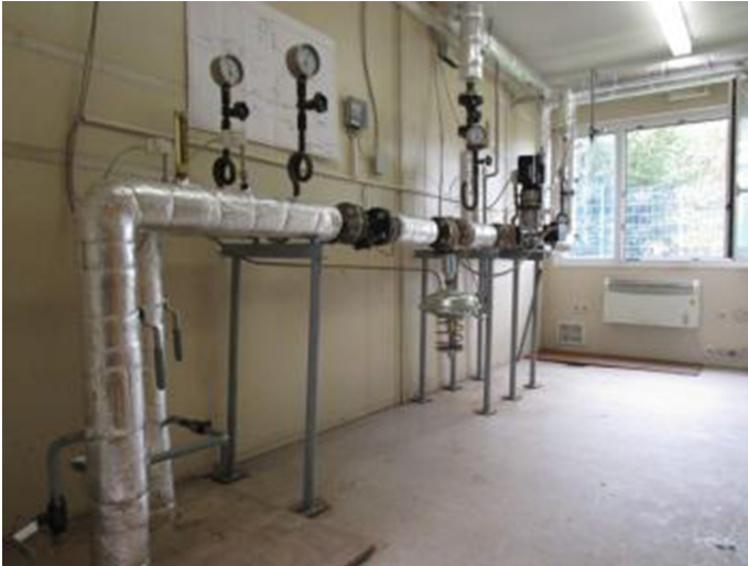
Fig. 1. Control unit showing devices and instruments, arrows indicate flow direction
