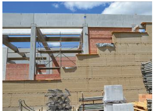
Figures 1 & 2. Ricola Herb Centre, Laufen by Basel, Switzerland, Herzog & de Meuron Architects, construction phase, July 2012. Production of prefabricated rammed earth elements and application on building site. Development, production and construction of rammed earth structures were made by Martin Rauch, LEHM TON ERDE.
