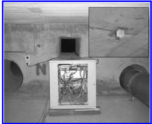
Figure 2. ‘ADVANCED’ monitoring system ROBO®CONTROL installed at Weyermannshaus Viaduct in Bern – Switzerland.
