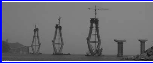
Figure 4. View of the 3-pylon cable-stayed bridge construction site of Busan-Geoje Fixed Link.
