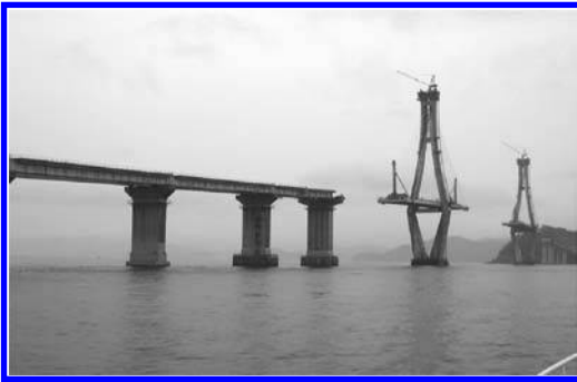
Figure 2. View of one of the two cable-stayed bridges (Geoga Bridge) of the Busan-Geoje fixed link under construction (total length: 8.2 km, central span: 470 m, design service life: 100 years).
