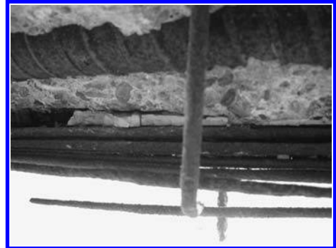
Photo 1. PC Tendon fractured by chloride attack 1) .
