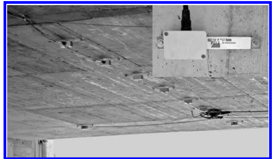
Figure 1. Typical B-WIM installation.
