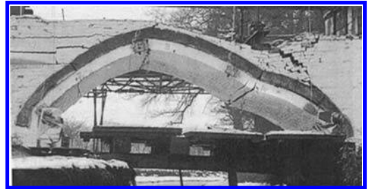
Figure 2. Prestwood bridge at the end of testing (Page 1987).
