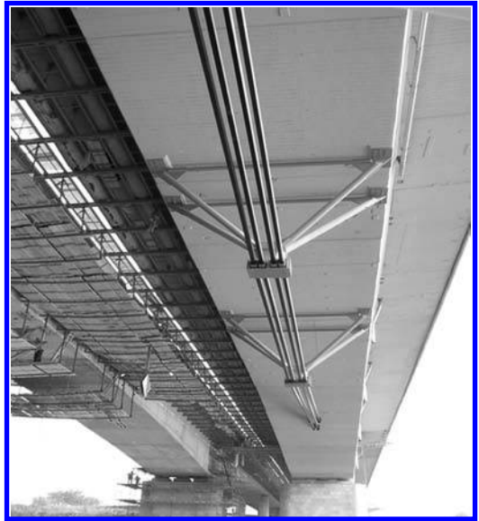
Figure 1. Bridge with excessive deflections after reparation process.
