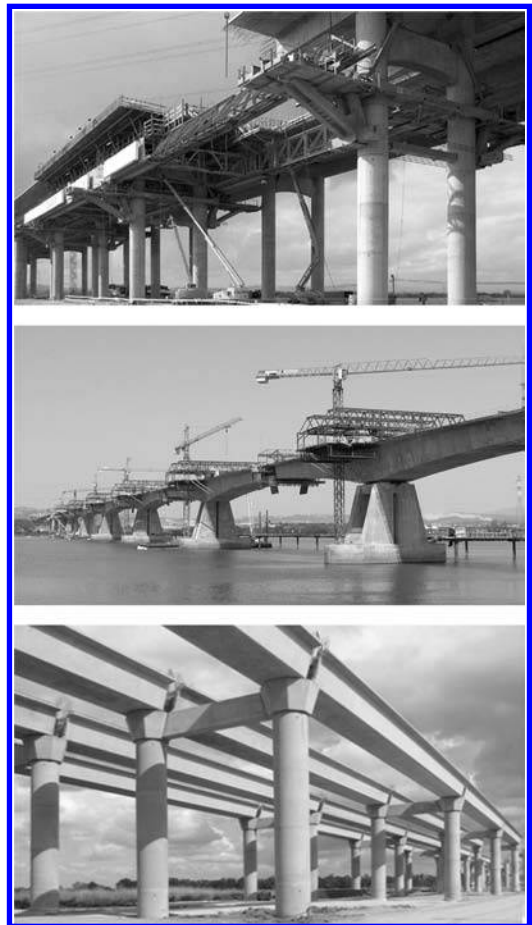
Figure 1. Lezíria Bridge – north viaduct (top), main bridge (middle) and south viaduct (bottom).
