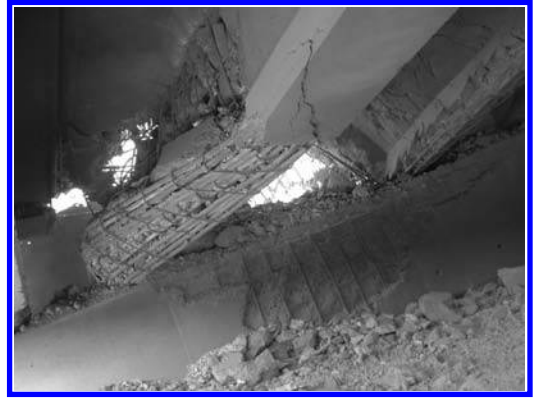
Figure 3. Explosively damaged girders.
