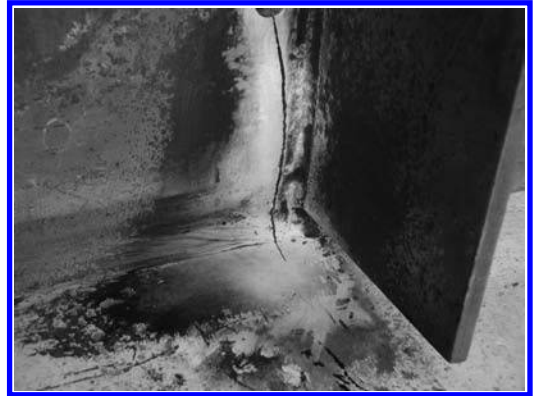
Figure 5. Crack into bottom flange.
