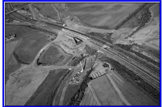
Figure 3. Aerial view of the A-231 motorway and the viaduct in Pergola in construction.
