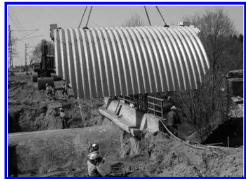
Figure 2. The construction of the steel culvert bridge. This new bridge was placed on top of an existing masonry arch bridge with a gap in between, which leaves the old bridge structurally functionless.
