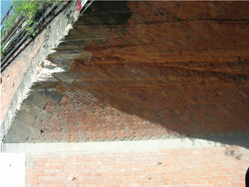
Fig. 6.18 Arch bridge after a car impact ( Picture D. Proske )
