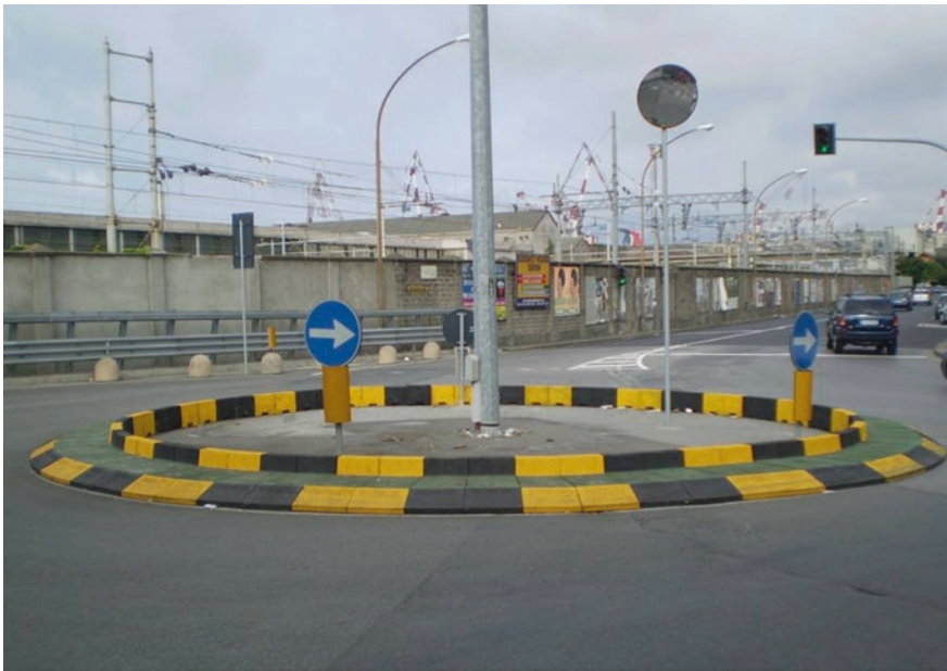
Fig. 4.3 Central island of an assembly roundabout, constructed from concrete prefabricated segment-shaped elements, Genova, Italy
