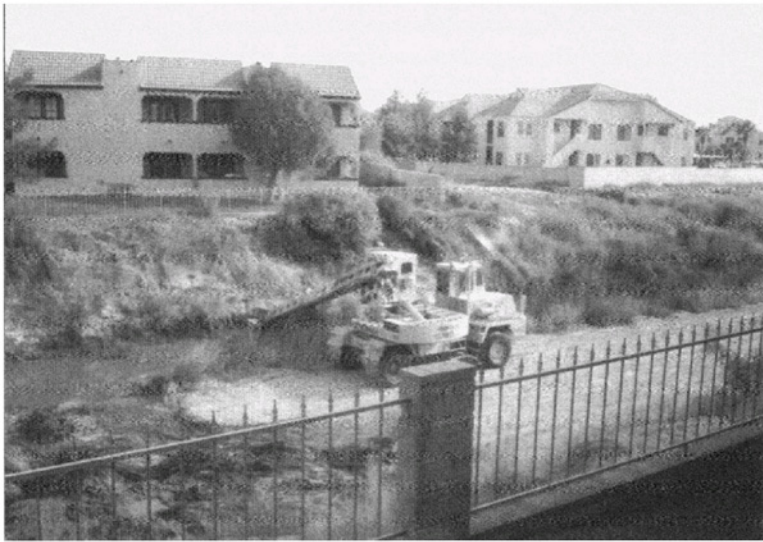
Figure 4.8. Drainage of storm runoff is vital to communities and maintenance is necessary. These conveyances are often high quality habitat in urban areas such as Henderson, Nevada.
