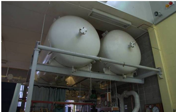
Figure 5. Air Storage Vessels
