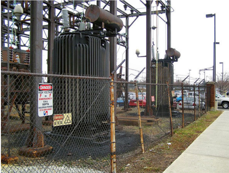
Fig. 3 Substation transformer (Sturmovik, GNU Free Documentation license, Wikimedia Commons)
