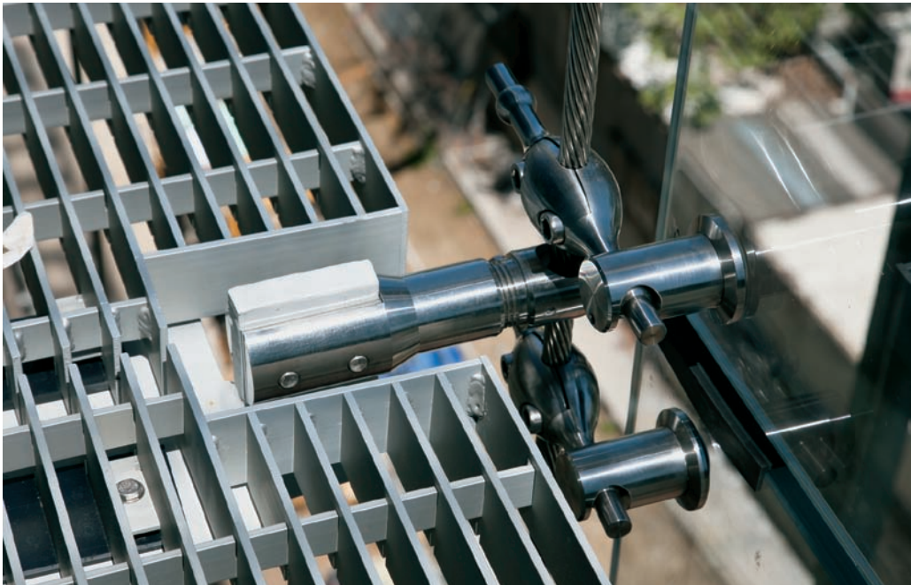
FIGURE 13.6 Outboard glass connection detail. The cable is attached to the end of a kicker extending from the floor slab that also supports the grating at each floor level. Note the up-down, in-out, and side-to-side adjustment mechanisms to accommodate installation tolerances.
