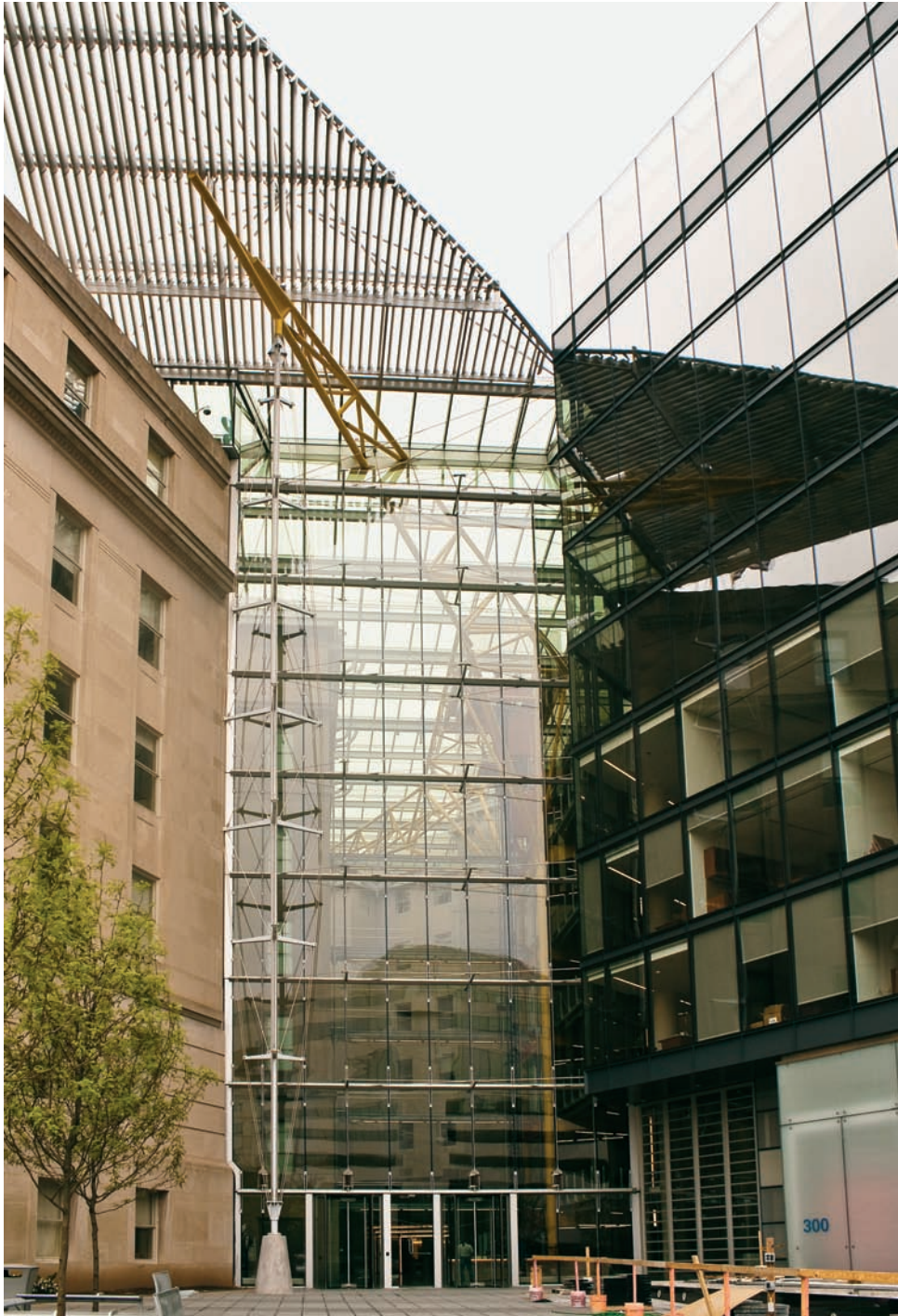
FIGURE 10.16 The atrium entry wall as the new building (to right) nears completion.
