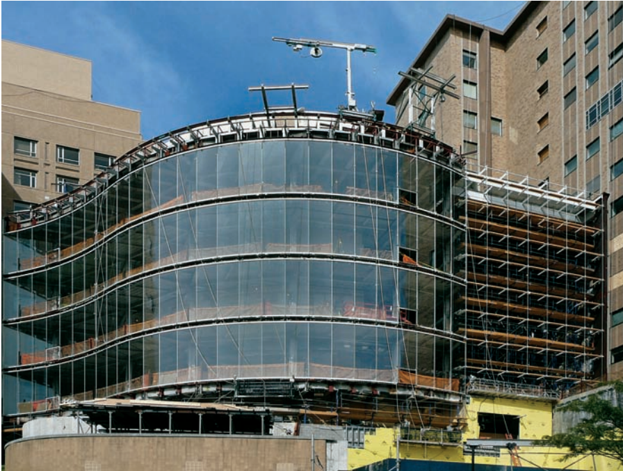
FIGURE 11.17 Construction photo of the climate wall facade on the left (the rod truss system was not yet installed) and the atrium on right.
