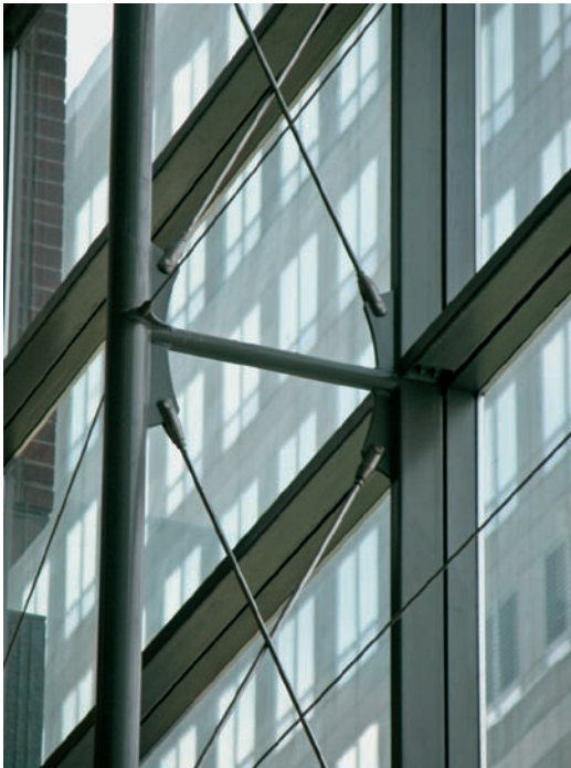
FIGURE 3.4 Detail of a simple truss system with cable bracing and an emphasis on craftsmanship.
