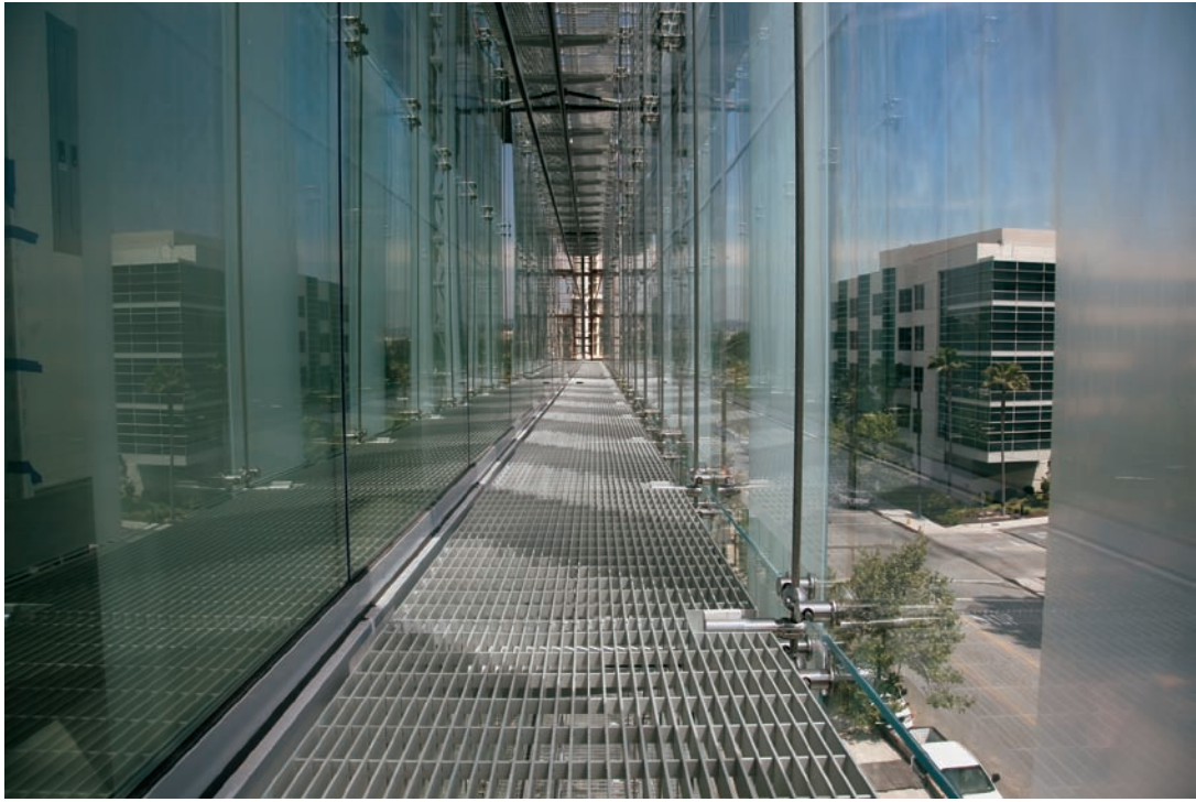
FIGURE 13.11 The cavity of the double-skin wall provides a thermal buffer for the building's interior.
