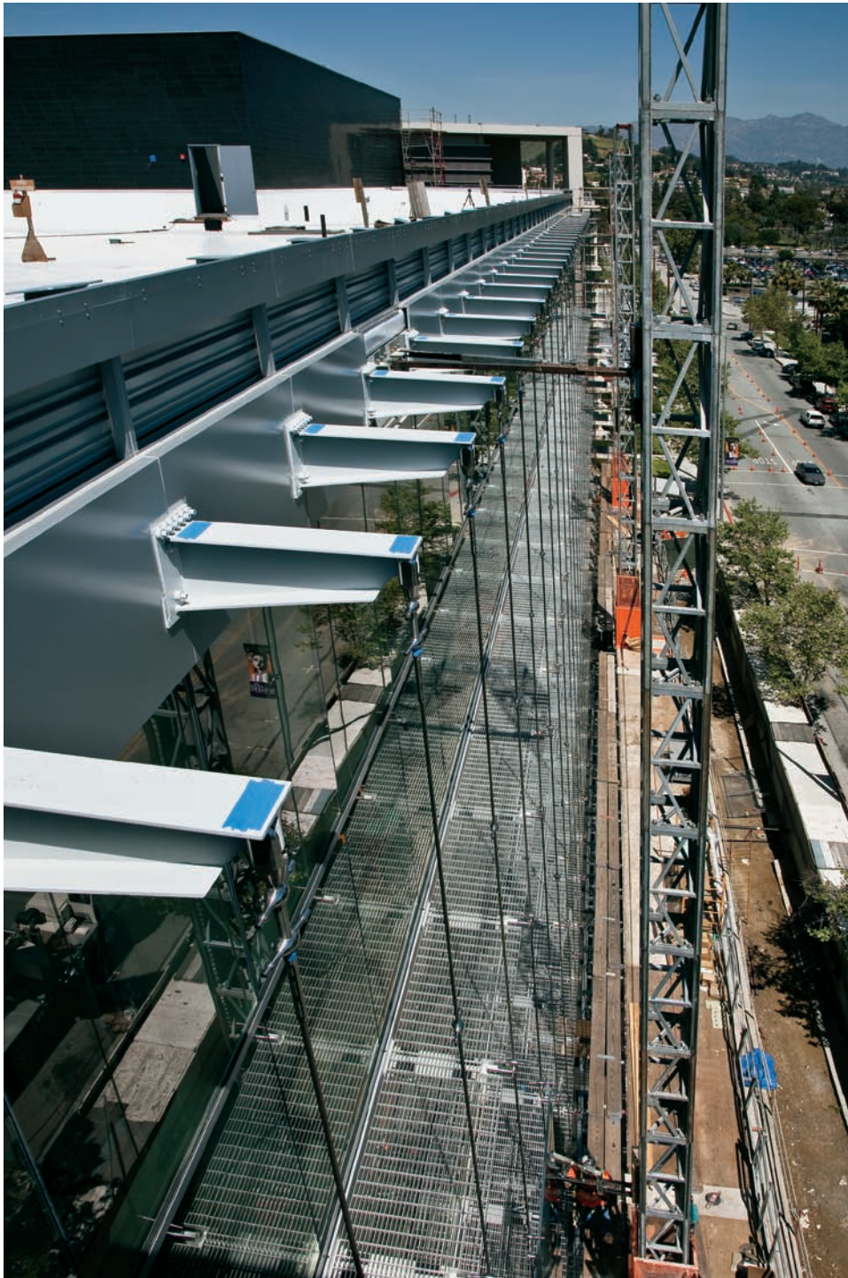
FIGURE 13.4 East facade under construction before the setting of the outboard skin. The cables are hung from the outriggers, and the grating is in place.
