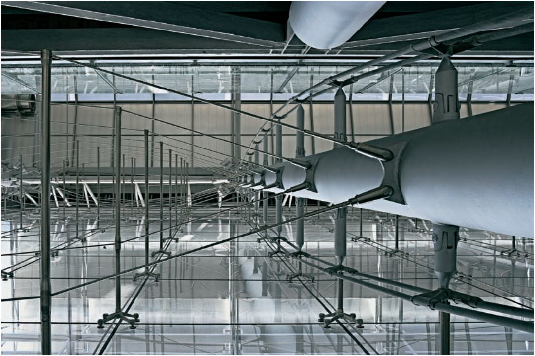
FIGURE 8.5 The view up a primary mast truss reveals bracing elements perpendicular to the glass plane and connections to horizontal cable trusses, which support the glass.
