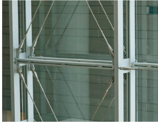
FIGURE 7.7 Each south wall facade includes a braced end bay to provide in-plane stability.
