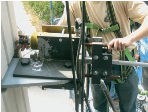
FIGURE 14.13 A horizontal cable is fixed to the shark fin and prepared for pretensioning.
