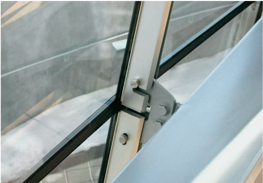
FIGURE 2.8 The panel system shown here consists of aluminum rails structurally glazed to two sides of an IGU. The system is butt-glazed.
