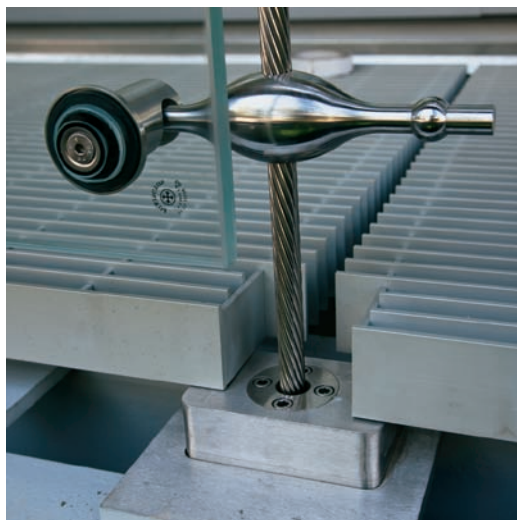
FIGURE 13.8 The cable base connection detail. The cable passes through a protective bushing to the bottom of a support girder that runs the length of the cable wall.
