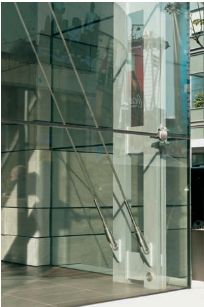
FIGURE 7.10 In-plane bracing at an end module of the south facade. Note the different foot design of the end truss.
