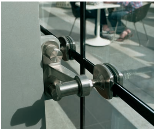
FIGURE 7.12 Typical glass system connection detail using a clamp-type component, requiring no perforation in the glass.
