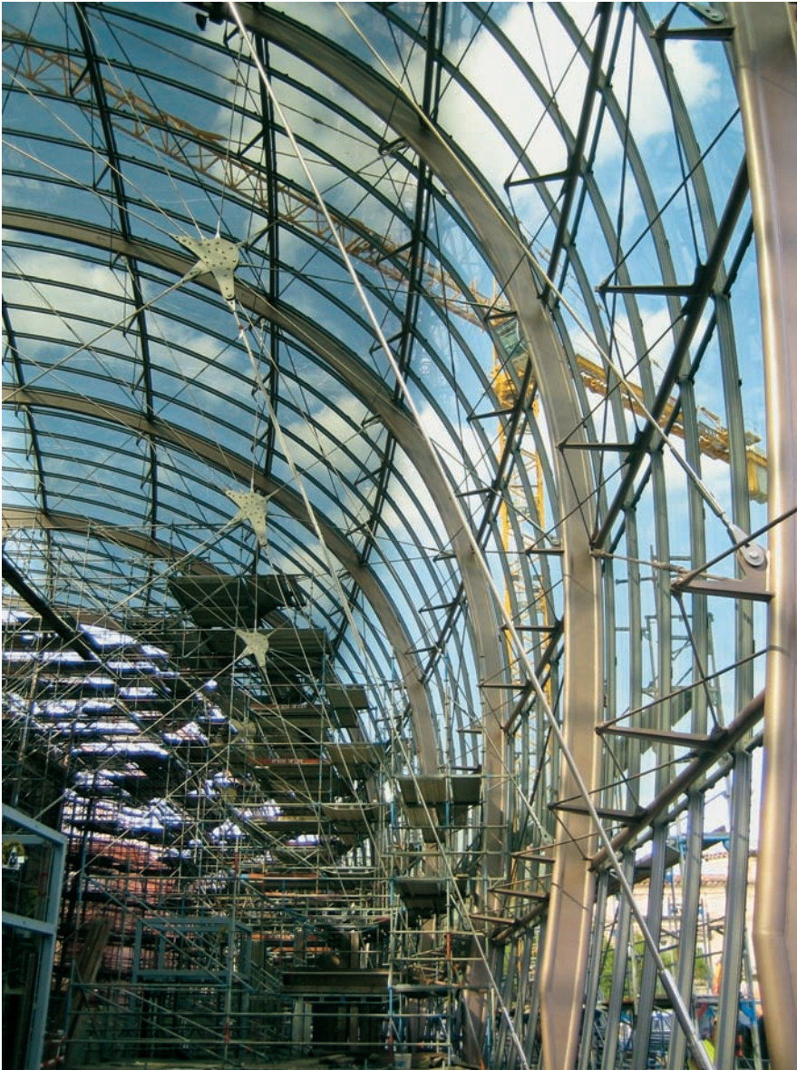
FIGURE 12.9 The steel arch and horizontal cable truss detailing is visible in this image during construction.
