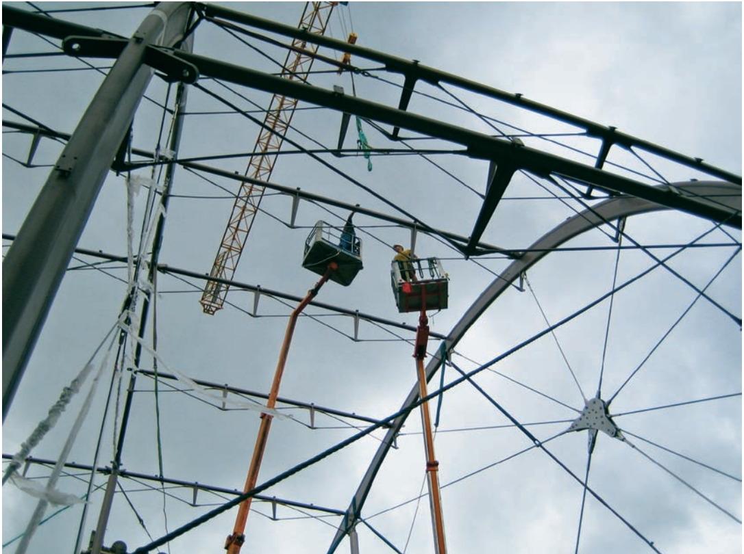
FIGURE 12.4 Horizontal cable trusses space the 30 ft (9 m) bays, and cables brace the arches.
