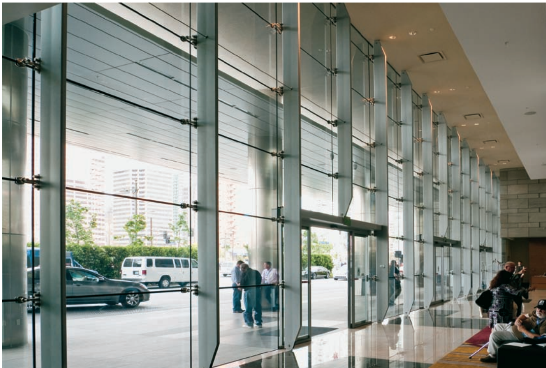
FIGURE 7.3 The north facade structure is a mullion system with a 25 ft (7.6 m) steel mullion tapering to a pin connection at the head and foot.
