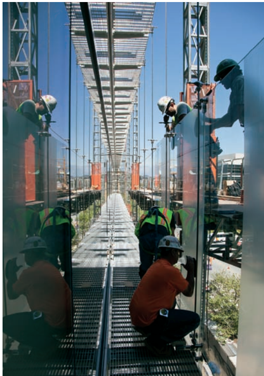
FIGURE 13.9 Construction workers install the outboard glass of the double-skin wall. Note the mast climber supporting the workers outside the wall, which provides access along the entire length of the facade.
