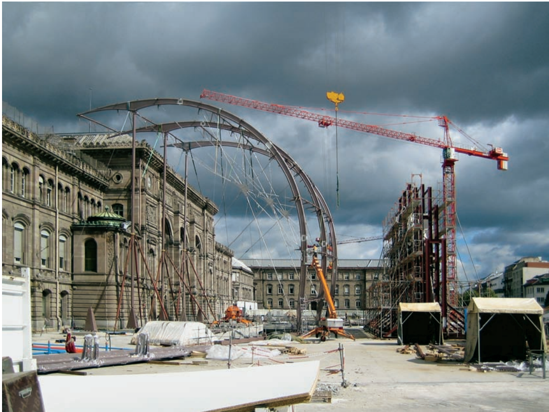
FIGURE 12.3 Steel arches frame the first two bays of the addition. Note that the new structure cantilevers out over the old building but does not touch it.
