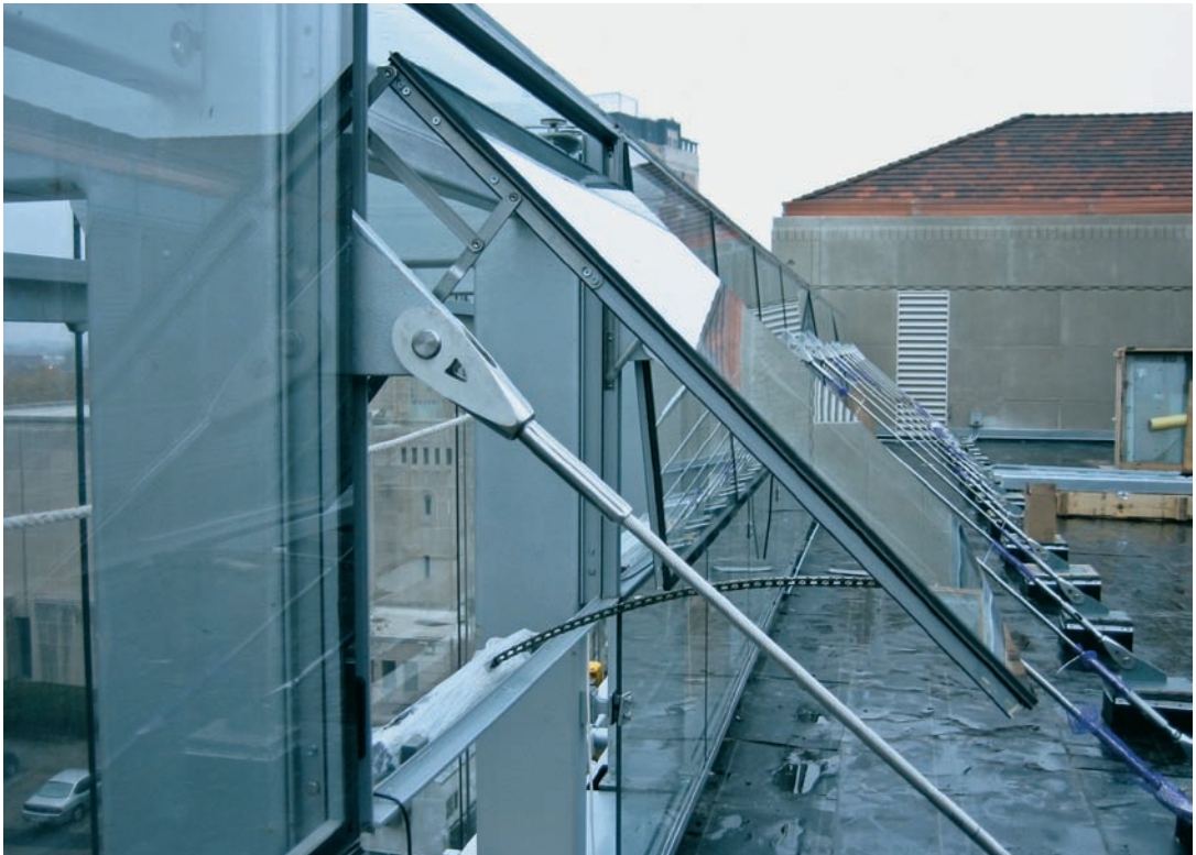
FIGURE 14.10 The hangman tieback at the top backside of the double-skin wall. The automated windows open to vent the cavity as part of the whole-building ventilation system.
