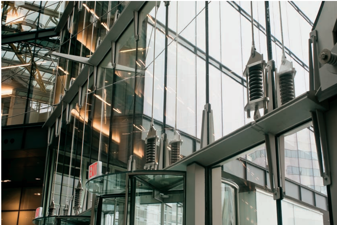
FIGURE 10.5 The wall is hung from tension rods that terminate in a spring connection at the door header, allowing the wall to deflect under lateral loads but returning it to its original position as the loads decrease and accommodating any vertical deflections while keeping the rods always in tension.
