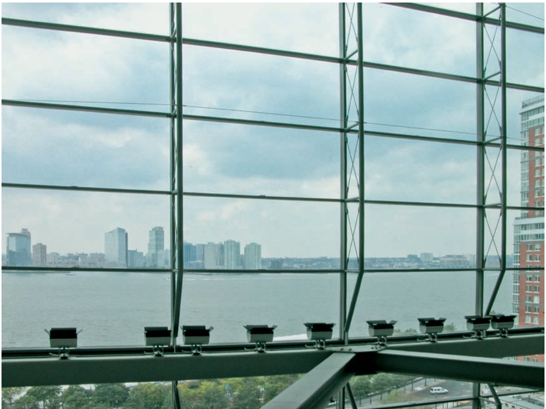
FIGURE 2.6 The exposed steel structure includes vertical trusses and bolt-up horizontal mullions, providing a grid to which a minimal veneer-type glazing system is fixed.
