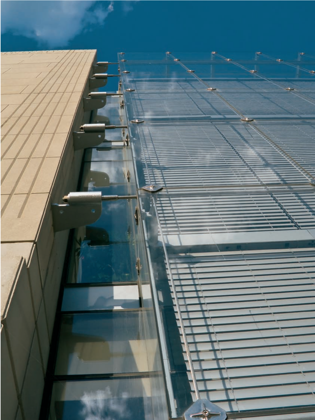
FIGURE 14.18 The horizontal cable terminations are expressed by a setback in the glazing plane.
