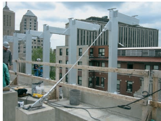
FIGURE 14.12 Hangmen being installed at the top of the double-skin wall. The tiebacks are pretensioned to 8 kips (36 kN).
