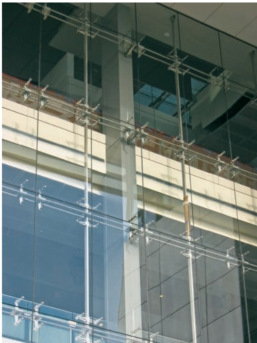
FIGURE 15.3 The horizontal cables are braced at two building columns to limit the overall span to 40 ft (12.2 m).
