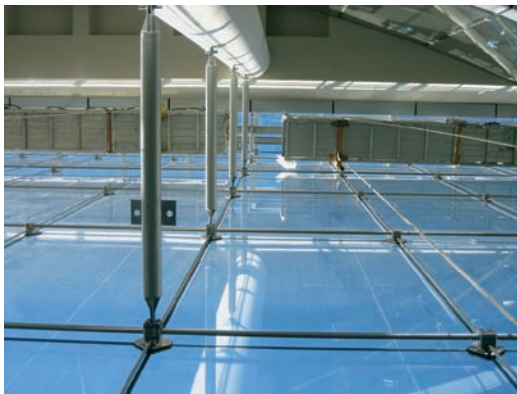
FIGURE 14.7 A view up the facade from inside the cavity reveals the kickers that tie the cable net to the building structure every 30 ft (9.1 m).
