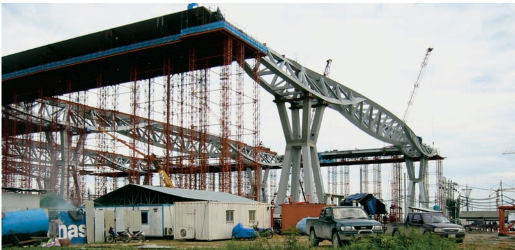
FIGURE 8.2 Eight supertrusses and column pairs provide the primary structure for the MTB, one of the largest single-building enclosures in the world.
