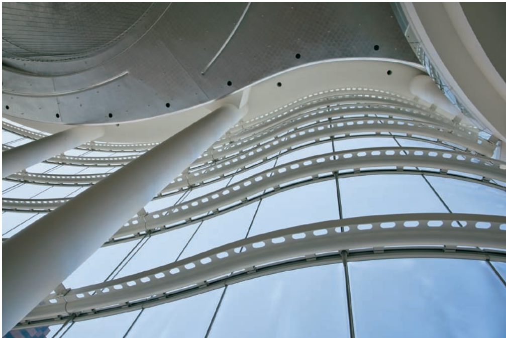
FIGURE 3.2 Curved horizontal mullions are suspended from stainless steel rods located on the vertical glass gridlines.
