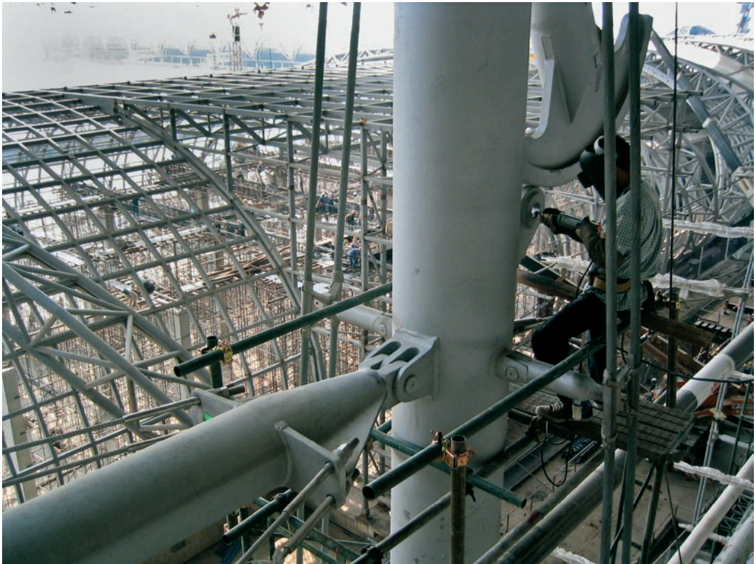
FIGURE 8.14 A worker prepares to connect a cable high up on one of the mast trusses.
