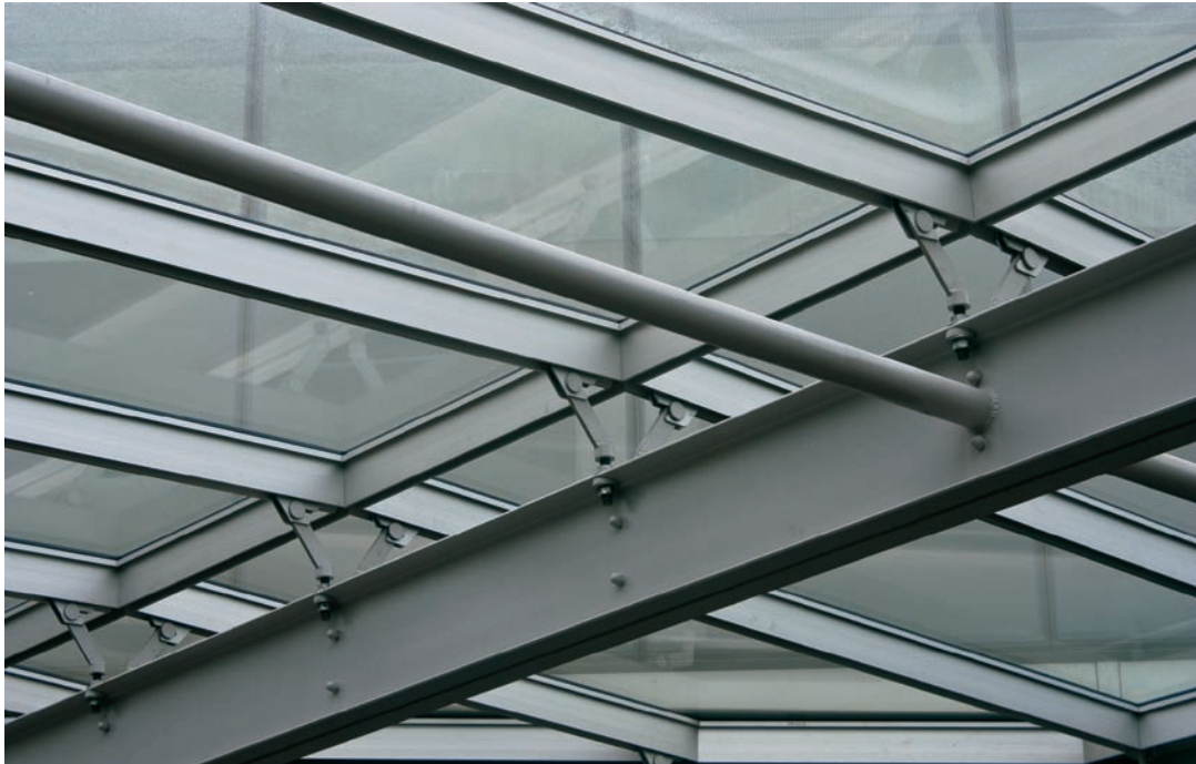
FIGURE 10.11 Glass roof detail showing the paddle arm and pin connection of the glass system to the ladder trusses. The primary structural member is actually split into two channels that are part of separate ladder trusses.
