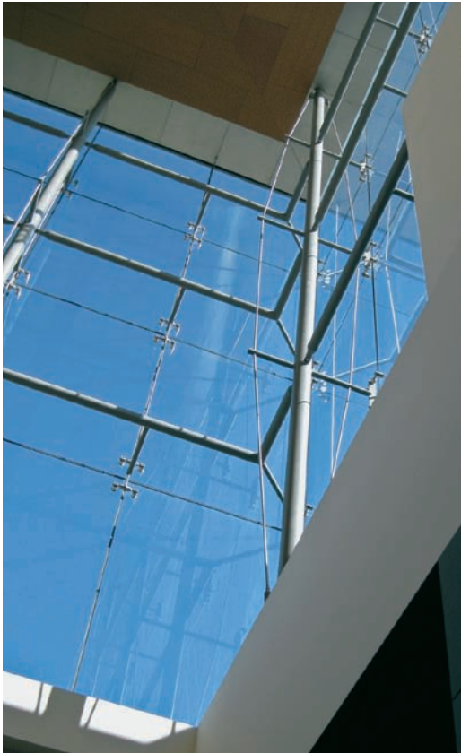
FIGURE 9.5 The corner condition is treated as an extended outrigger, simplifying the structure and heightening the facade's transparency.
