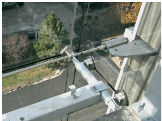
FIGURE 14.9 Construction shot showing the shark-fin cable anchor at the right and the glass-fixing strut at the glass return. Note the penetration of the cable through the glass at the joint.
