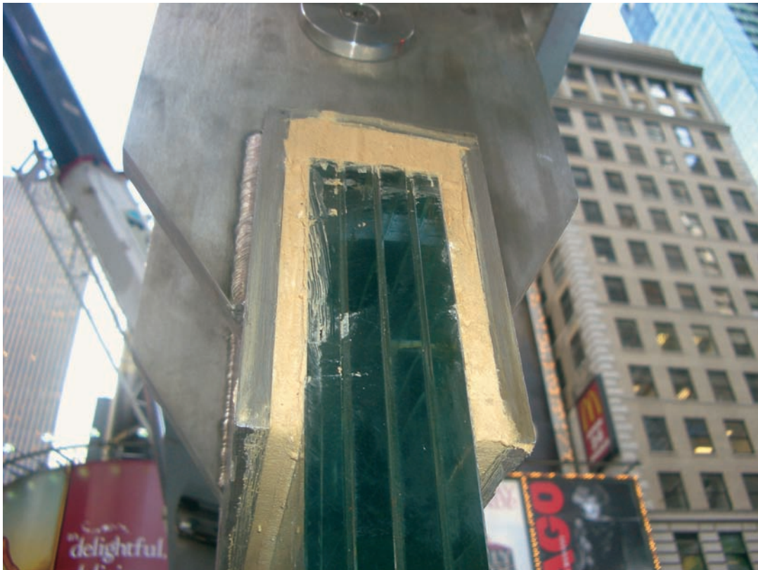
FIGURE 6.11 A construction detail at the midwall connection shortly after the application of grout, which ensures uniform bearing of the beams on the four-ply glass wall.
