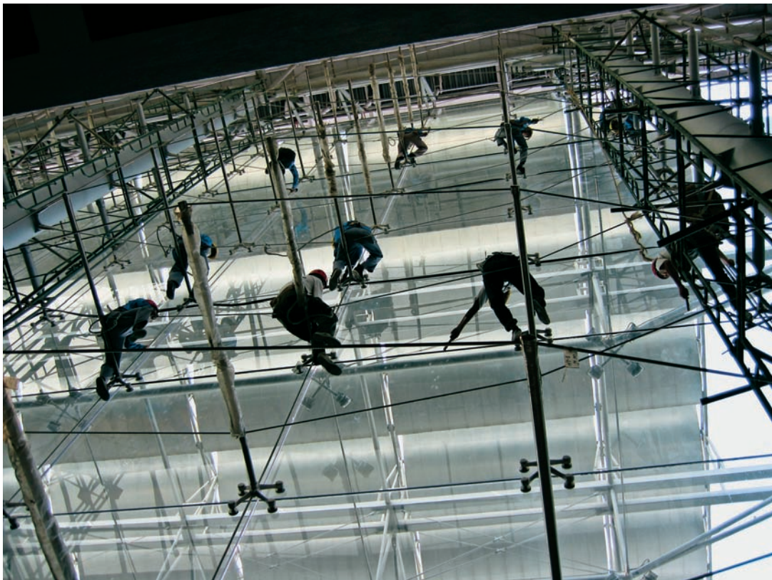
FIGURE 8.15 A caulking crew applies the silicone material that provides the weather seal.
