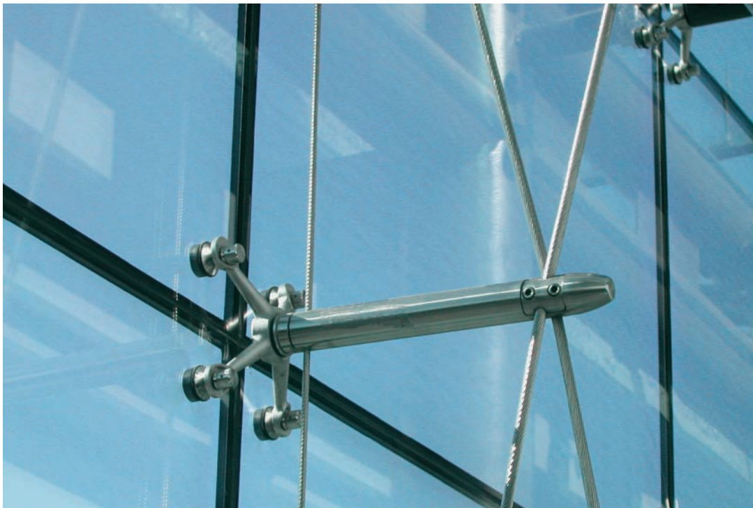
FIGURE 2.9 A point-fixed bolted glass system using a spider fitting and perforated glass. A specially designed bolt penetrates through the perforation to fix the glass. The glass dead load is usually carried at the connections at the top of the panel.
