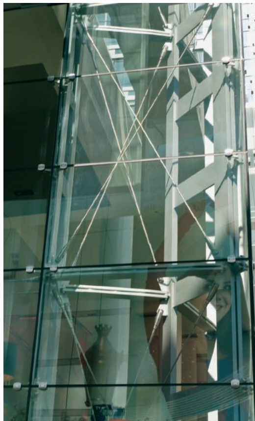
FIGURE 7.8 This corner truss is a unique condition at the interface of two perpendicular wall segments that comprise part of the south facade enclosure.
