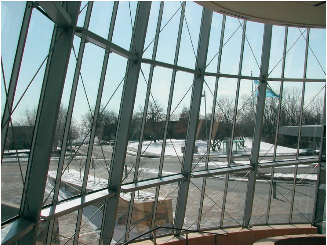
FIGURE 4.5 This system was used to enclose the lobby of a corporate office building.
