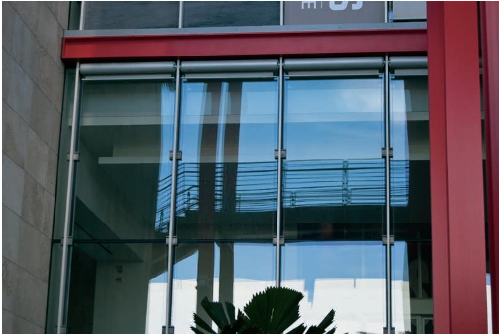
FIGURE 3.1 A vertical mullion system using a thin steel plate mullion with a minimal sight line. The clips at the side clamp the glass in place.
