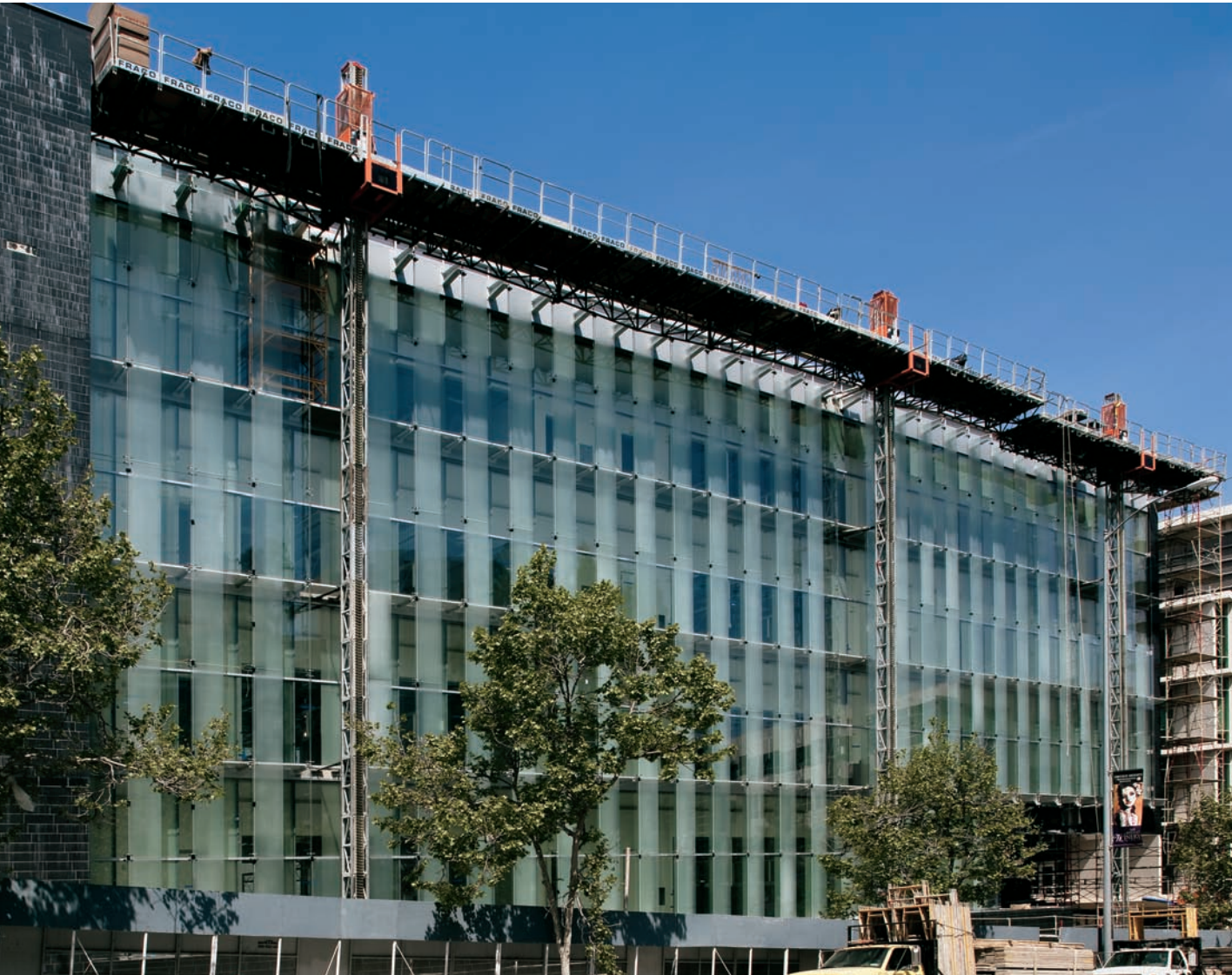
FIGURE 13.1 The east elevation, here under construction, is dominated by a full-building-height double-skin facade. Note mast-climber rig used to set glass.
