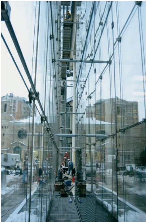
FIGURE 14.3 Technicians work within the double-skin cavity. The cable net is the outboard skin to the left, and the inboard skin is the VS-1 system.
