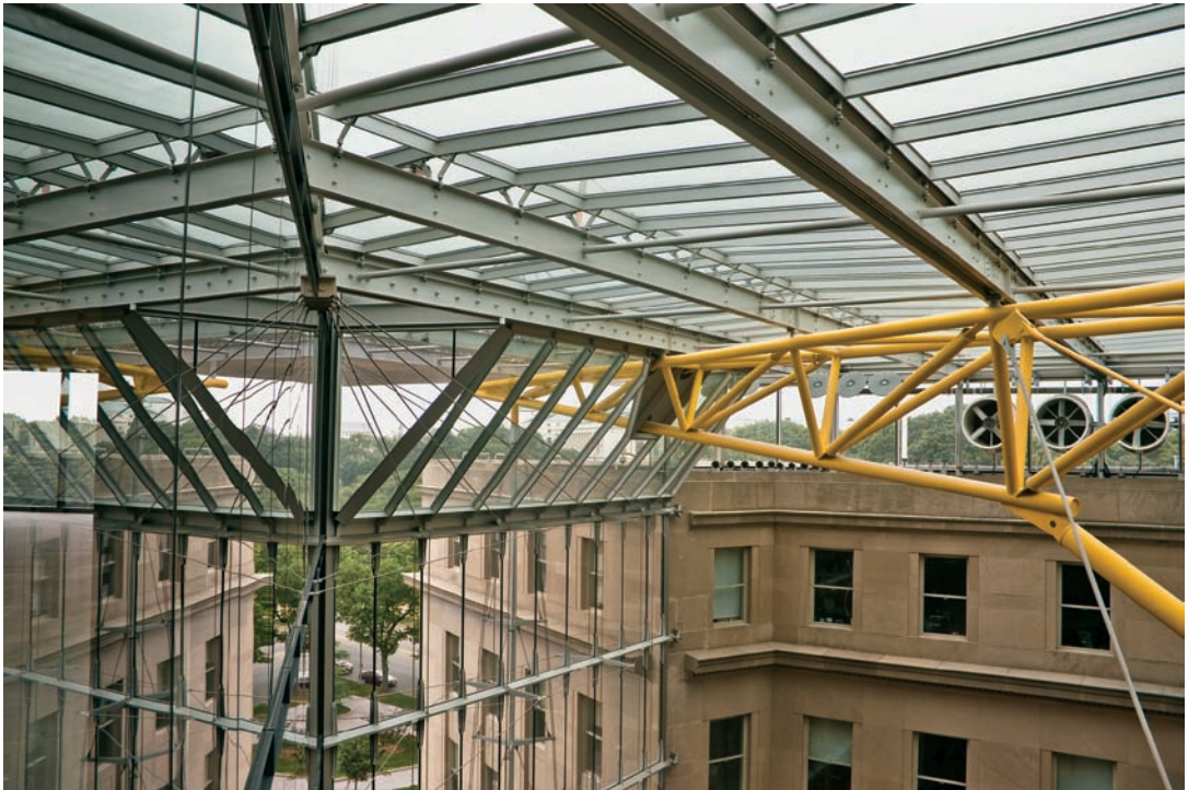
FIGURE 10.12 The yellow roof support truss penetrates the sloped skylight transition through a metal panel.
