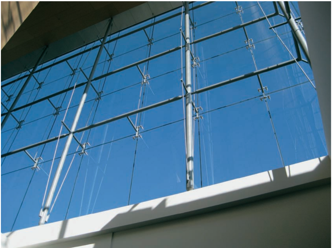
FIGURE 9.2 The basic facade structural system consists of alternating cable trusses and suspended horizontal outriggers.
