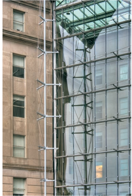
FIGURE 10.9 A mast truss supports skylight framing that extends over the entry area and contains shading louvers.
