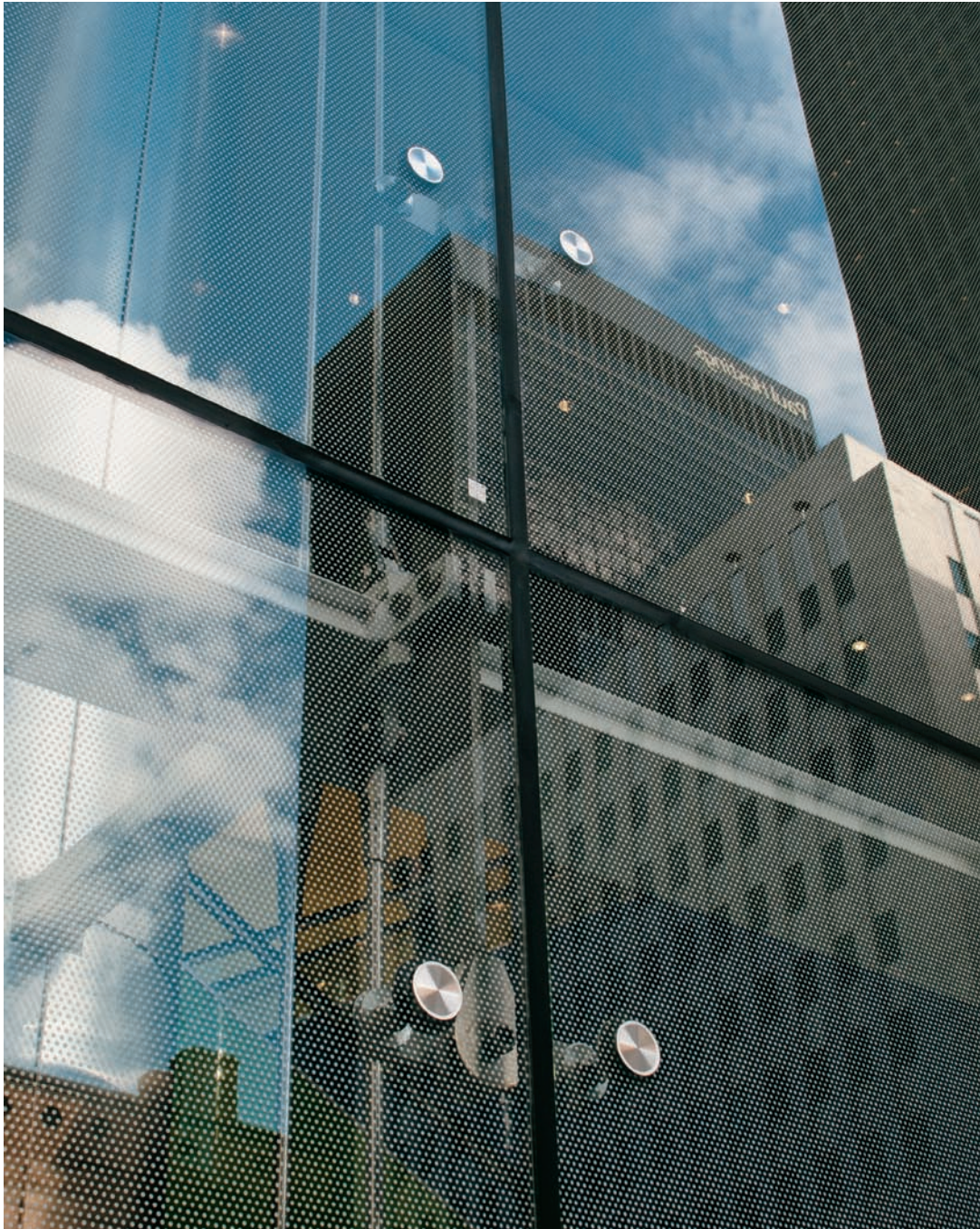
FIGURE 2.5 A butt-glazed joint is produced by the field application of wet silicone material to the gap between adjacent glass lites. The material gradually cures to a tough rubbery consistency. The technique produces a reliable and durable weather seal. Detail from a glass wall provided by Novum Structures, 2010, at the lobby of a downtown Los Angeles high-rise.
