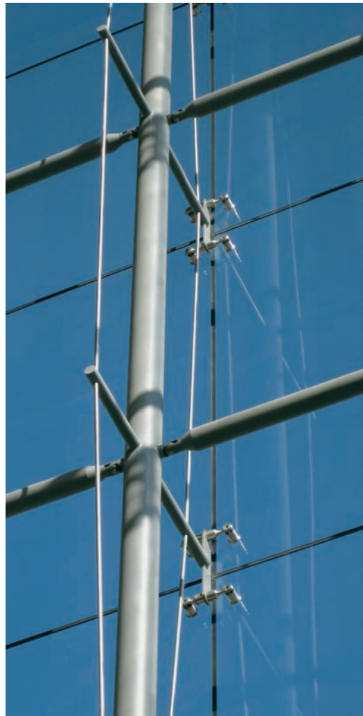
FIGURE 9.4 Bracing struts welded to the mast extend to the glass plane. A vertical plate welded to the strut end provides for the attachment of the glass fixings.
