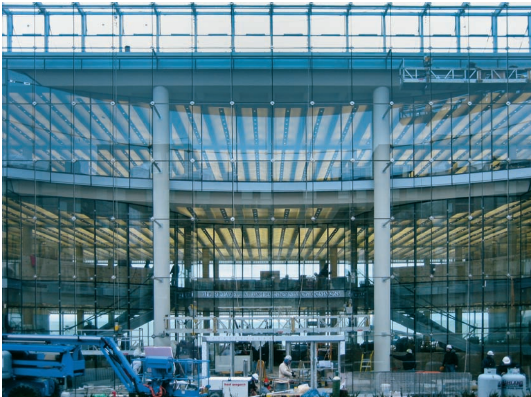
FIGURE 14.2 The entry of the west facade during construction. Note the view to Lake Michigan beyond.
