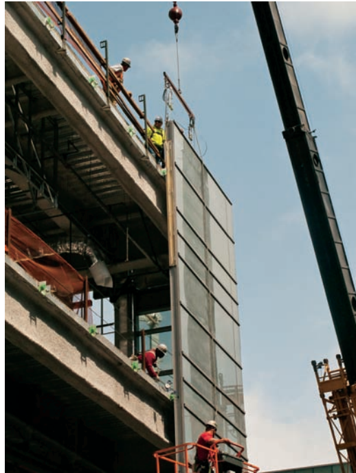
FIGURE 2.7 A large curtain wall unit containing over 30 glass panels being positioned for attachment to building anchors.
