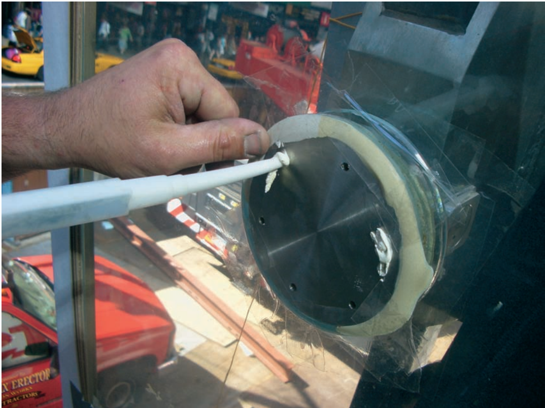
FIGURE 6.12 The rotule fitting is suspended in the glass hole as grout is applied through injection holes in the rotule cap plate. The design allowed for visual confirmation that the material was applied free of voids.
