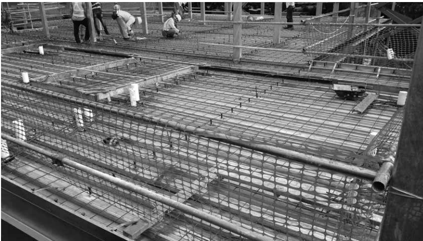
Figure 6.6 Profiled metal deck composite slab under construction (shear studs indicate beam positions).
