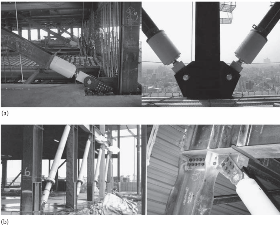
FIGURE 7.3 (a, b) Damper connection details. ((a) Courtesy of Taylor Devices, Inc. North Tonawanda, NY. and (b) Courtesy of ITT Enidine, Inc. Orchard Park, NY.)
