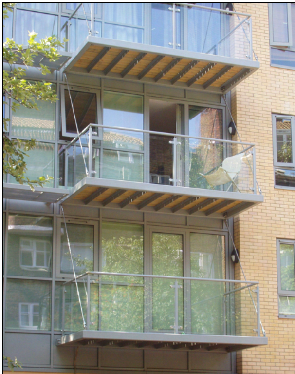
Figure 6.6 Tied balconies St Edmunds Terrace, Primrose Hill, London (Courtesy of HTA Architects)
