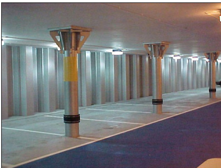
Figure 7.2 Millennium Car Park, Bristol showing sheet piling and the column head detail supporting the floor slab
