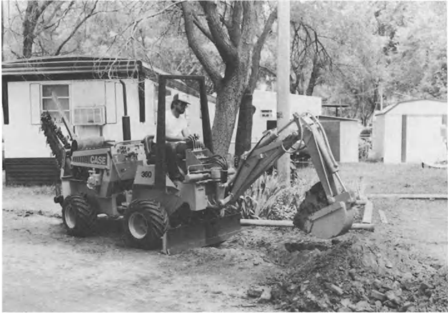
FIGURE 3-2. A backhoe in the process of cutting a trench for visual examination of a soil profile. [Ref. 7]
