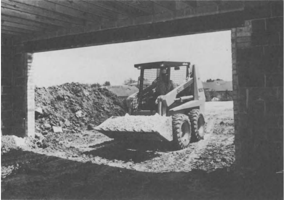
FIGURE D-3. Access as required for the delivery of stone base for use under slab on ground. [Ref. 7]
