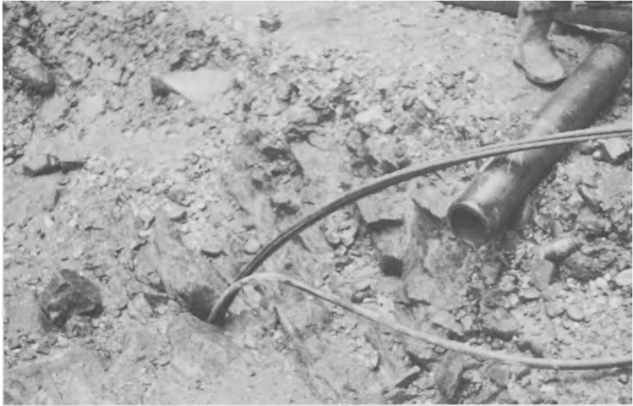
FIGURE 8-20. Rock anchor cable and grout tube positioned in hole prior to grouting the dead end anchorage. [Refs. 9 and 12]
