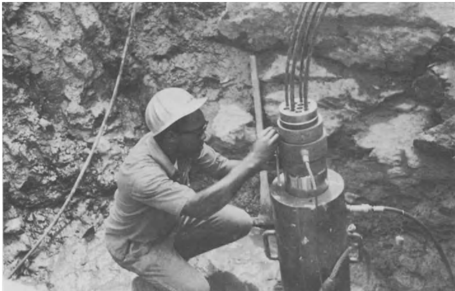
FIGURE 8-21. Measuring the rock anchor elongation after the cable has been pre-stressed. [Refs. 9 and 12]
