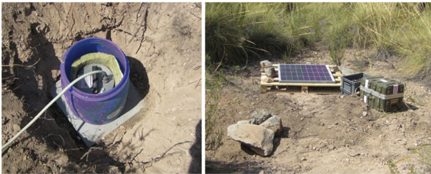
Fig. 7.12 A simple temporary field installation. Left: A hole is prepared with a leveled ceramic base at its bottom, cemented with concrete. The BB sensor (Güralp CMG3T) is on the base protected with a plastic barrel with its bottom lid cut off and positioned on a thick glass fiber foam thermal isolator in close contact with the sensor. Once the top lid is closed, the barrel is buried with soil. Right: A view of the complete station. The stones mark the sensor location. The recorder, including GPS antenna, is inside the fiber box. The battery and charge regulator are in an open plastic box and a solar panel is fixed to a wooden base almost horizontal (this would not be practical at high latitudes). Once finished, the recorder and battery boxes are covered with a plastic fabric and soil. If there are cattle or wild animals in the area, the station should be protected with a fence
