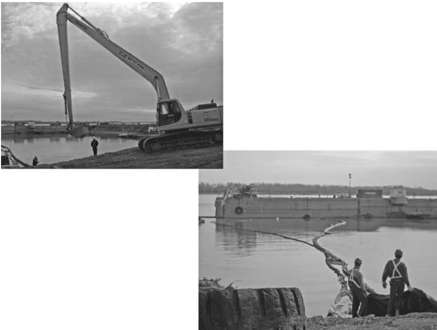
FIGURE 9.3 Photographs of sediment removal and silt curtain during restoration of Sector 103 in Montreal, Canada.
