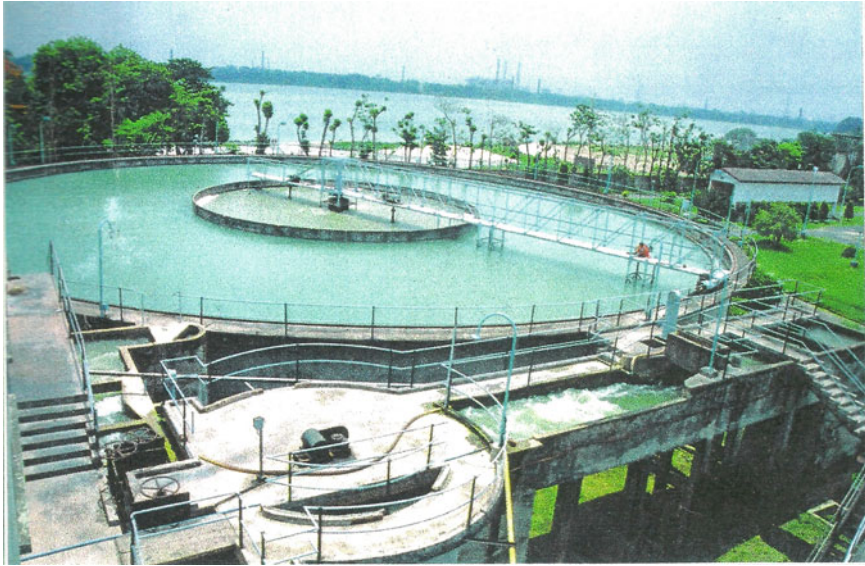
Exhibit 12.1 Serampore Water Treatment Plant showing Parshall Flume, flash mixer and clariflocculator
