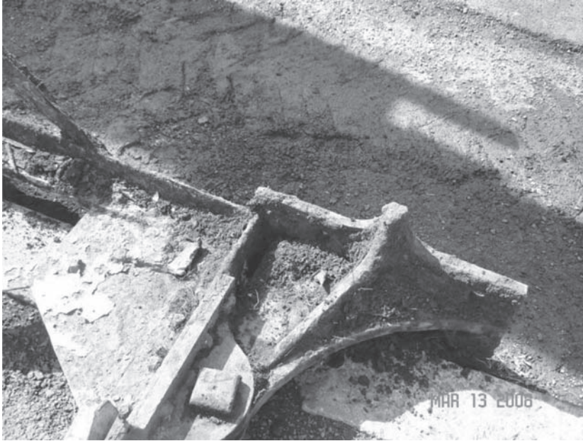
Figure 17. Existing movable bridge bearing uncovered during the removal of the existing draw span.
