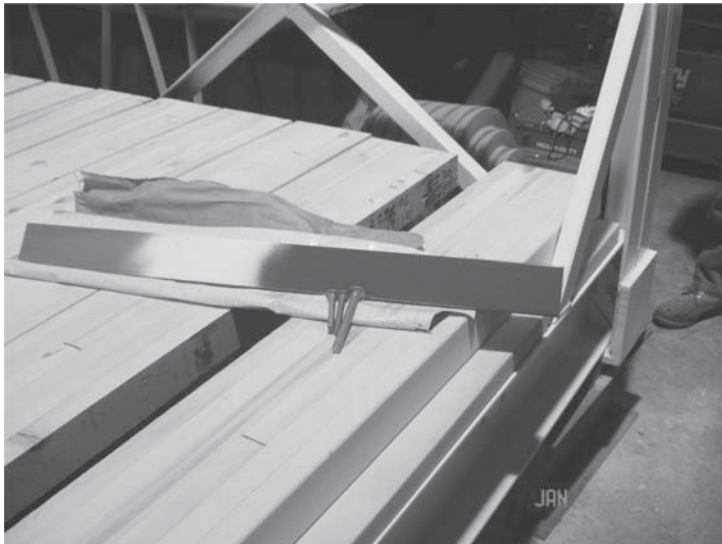
Figure 18. Paint sample for approved three coat system. Note rehabilitated sheave assembly in the background.
