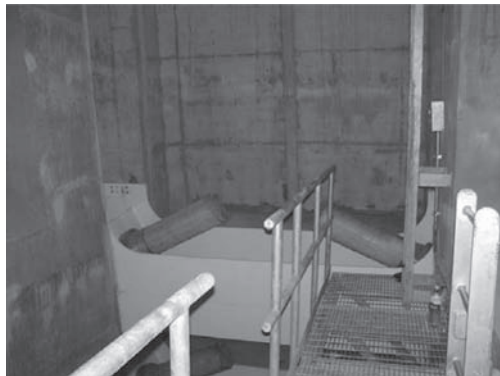
Figure 13. Large chamber on tower top allows cable anchors to be readily accessed by ladder and platform.
