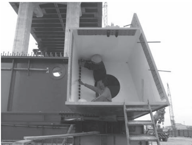
Figure 6. The edge girder box was designed for people to work comfortably inside.
