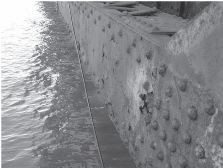
Figure 8. Dumbarton bridge—typical failed paint on truss member.
