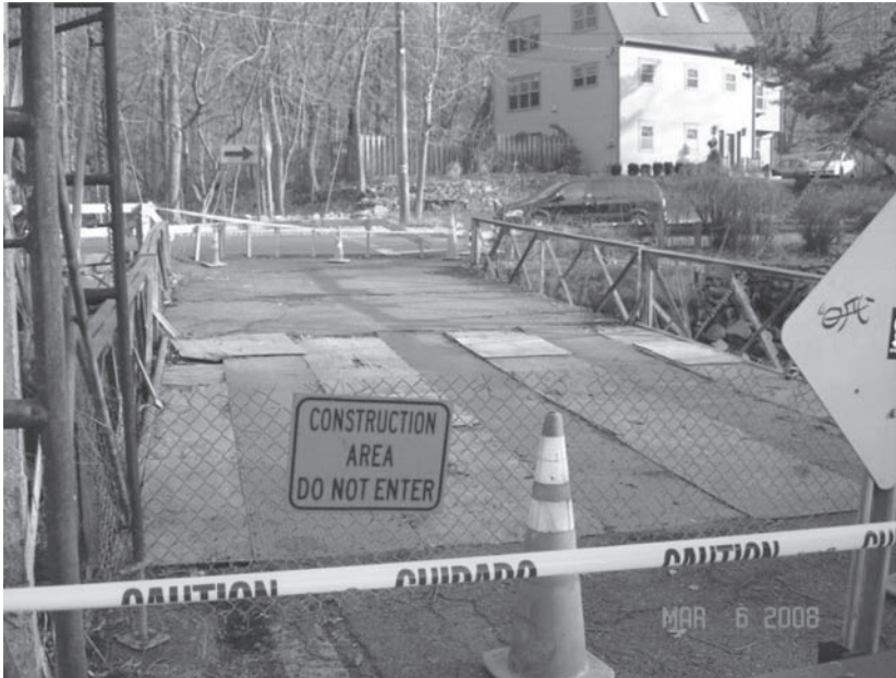
Figure 5. View looking south across the deteriorated timber deck on the bascule span at the start of construction. Also note the asphalt overlaid concrete approach deck and lateral deformation of the approach truss.
