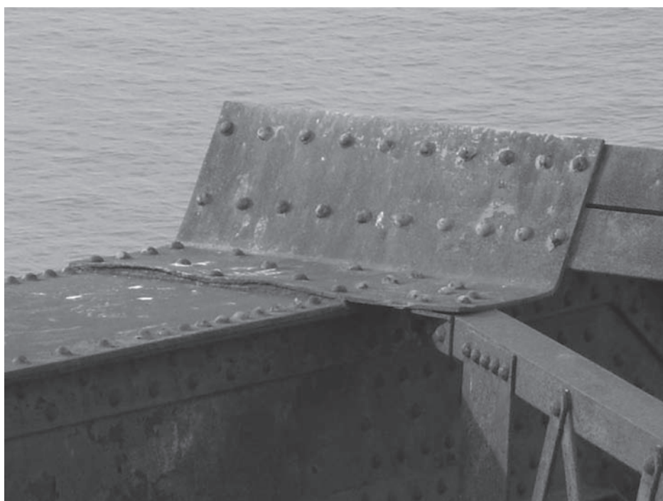
Figure 9. Dumbarton bridge—typical corrosion and pack rust of steel truss member.
