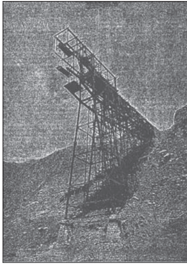
Figure 11. View showing newly built west pier and use of traveler to build out cantilever span.
