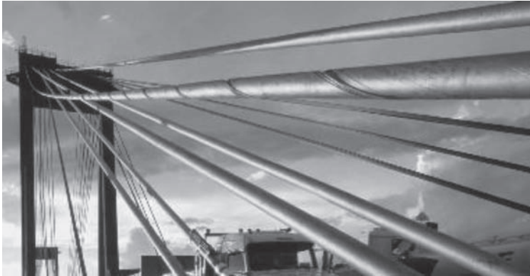
Figure 1. Obvious damage on a locked coil cable, Gal Belgrano Bridge, Argentina.
