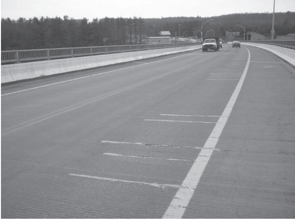
Figure 5. Cracks, sealed and unsealed, forming above the main steel in grid panels.
