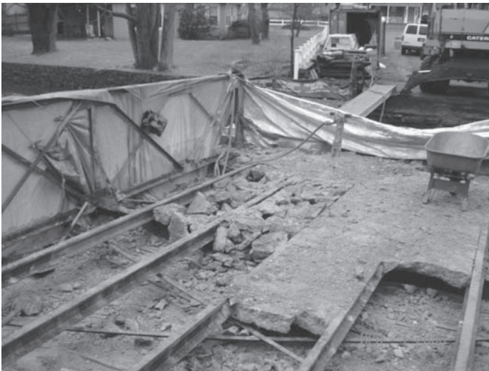
Figure 9. Demolition of the concrete approach deck uncovered used rails in the deck.
