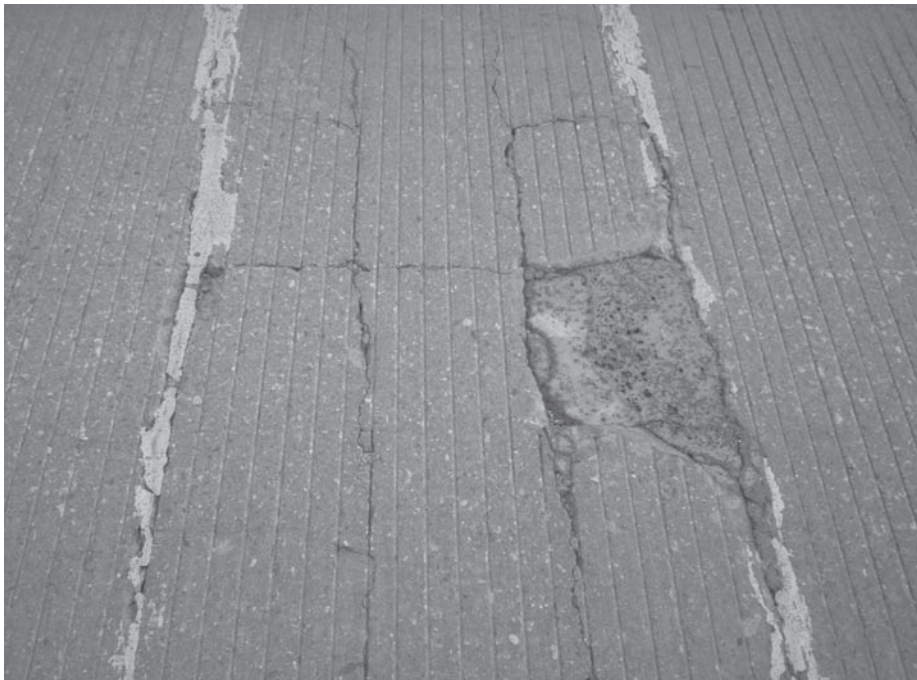
Figure 6. Failed area of deck panel.
