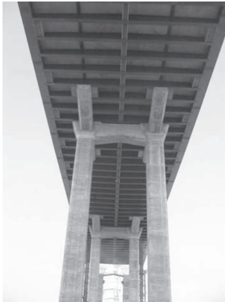
Figure 9. Underside of the superstructure at anchor piers showing, catwalk, platforms, and floorbeams. Counterweights are located at the tip of the cantilever arms.
