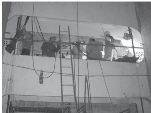
Figure 14. Cable connection frame inside the tower provides a convenient work platform for cable installation.
