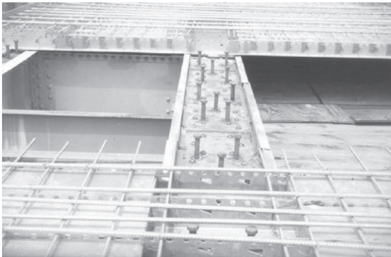
Figure 3. Steel grid panel and top mat reinforcement. (Note holes in transverse primary grid member. Concrete is placed from 4" above the grid to 1" below the grid thereby filling these holes and engaging the steel to the concrete).
