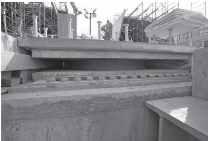
Figure 9. Disk bearing installed on I-35W Bridge showing containment plate.
