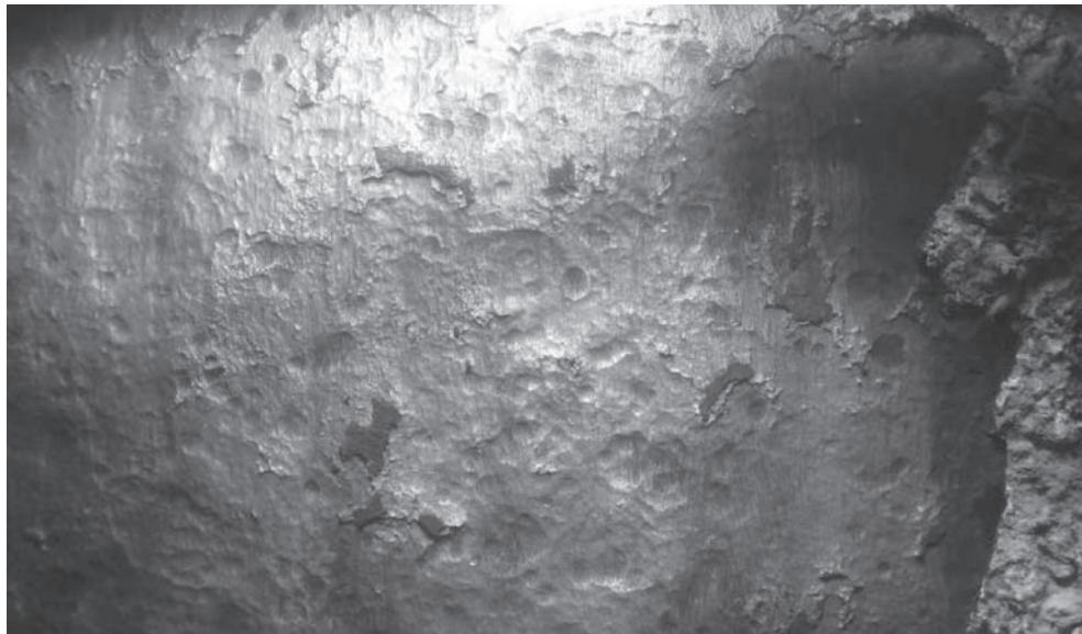
Figure 5. Dumbarton pier 6, Northwest caisson, SE Quadrant, 9.5-ft below MLW. Typical steel in 1-ft above to 10-ft below MLW, typical condition of steel shell.
