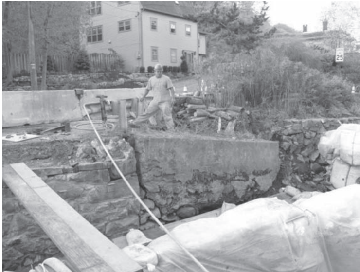
Figure 11. Movement of the southwest wingwall.
