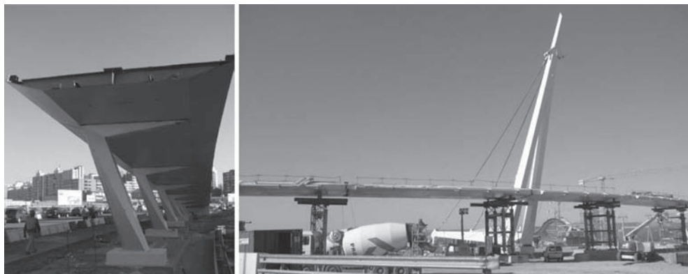
Figure 23. Access ramp (left) and main span during construction on temporary supports (right).
