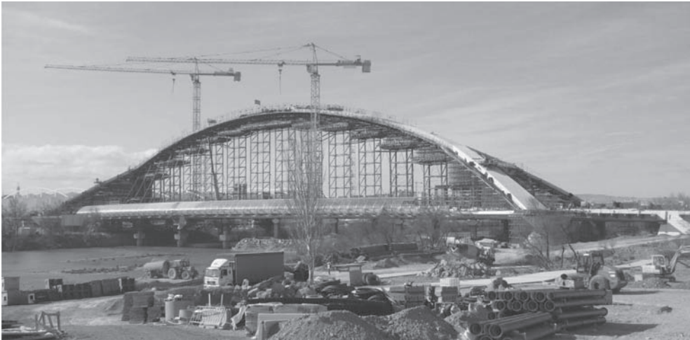
Figure 20. Constuction of the arch over a scaffolding supported by the previously launched deck.
