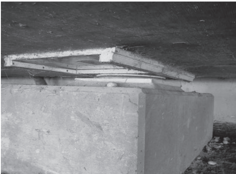
Figure 4. 30 year old disk bearing on the Pasco Kennewick Bridge.
