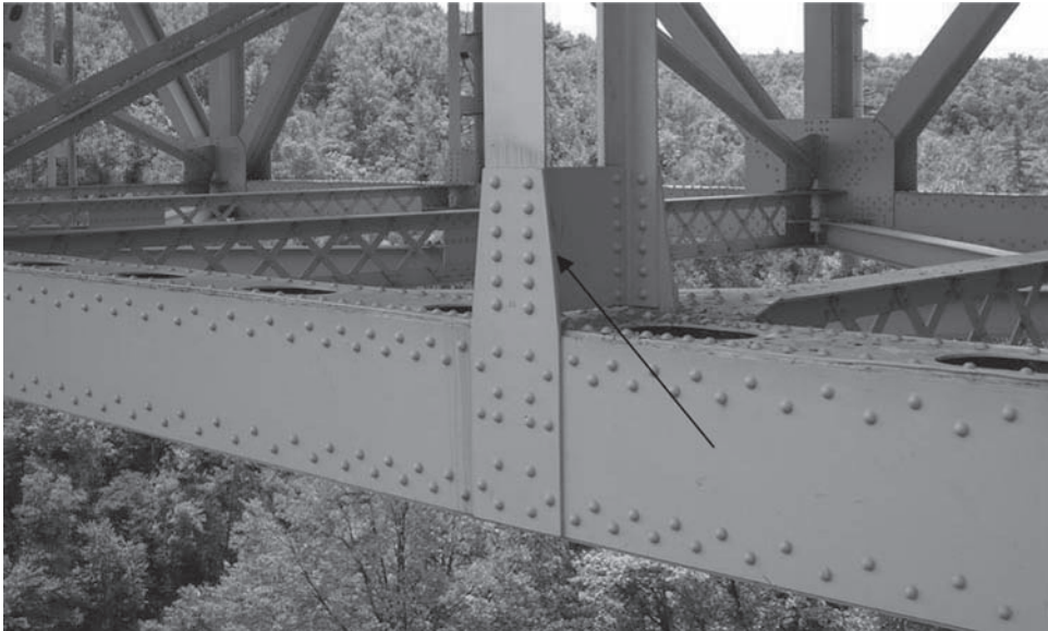
Figure 4. Typical lower, even numbered gusset plate, identifying unsupported edge. It can be seen that there are rivets near the edge for its entire length.
