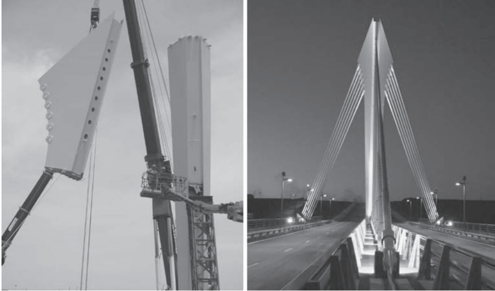
Figure 10. Erection of the steel inclined mast, and night view of the finished structure.
