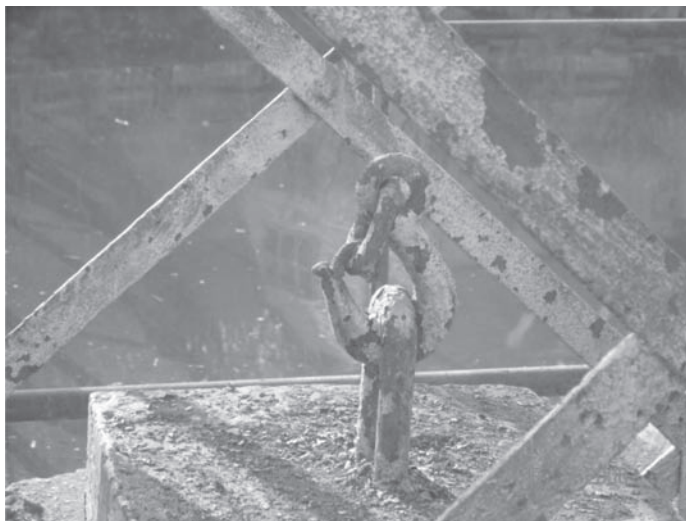
Figure 7. Severed link at northeast counterweight chain.
