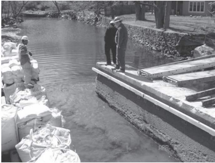
Figure 10. Concrete pier leaning toward the north.
