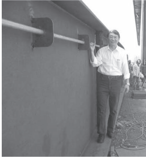
Figure 12. Walking on top of the floorbeam bottom flange is very comfortable and safe.
