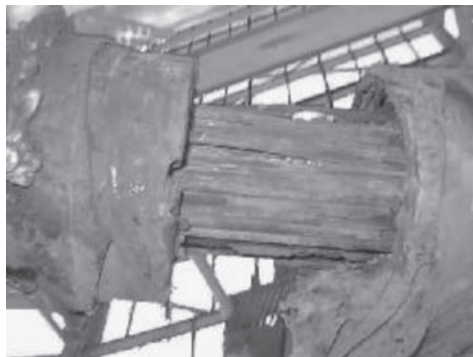
Figure 2. Example of gangrene effect on a PWS cable, Zarate Bridge, Argentina.
