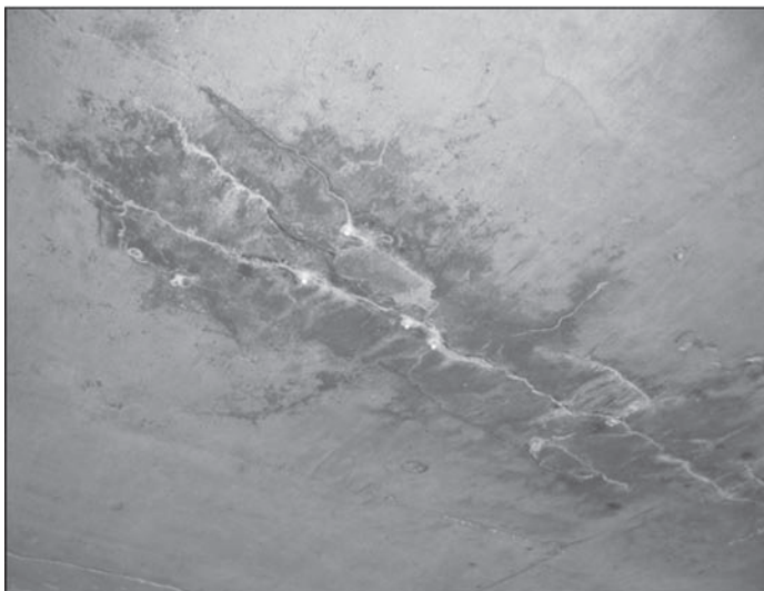
Figure 5. Photograph showing efflorescence, spalling, and rust-staining.
