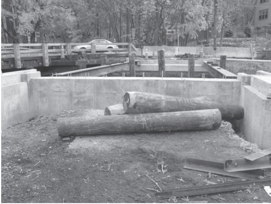
Figure 14. View looking south from behind the north abutment. Note new timber piers and the reconstructed southwest wingwall.
