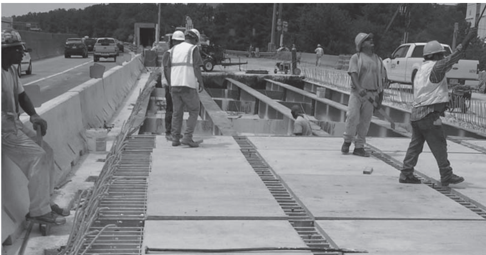
Figure 4. Precast panel installation on I-285 near Atlanta, GA (Photograph courtesy of L.C. Whitford).
