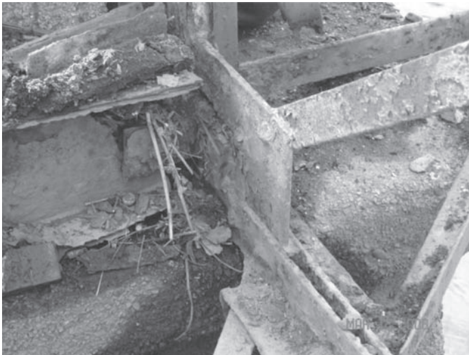
Figure 12. Severely corroded end floorbeam and truss gusset plate that were buried at the north abutment.
