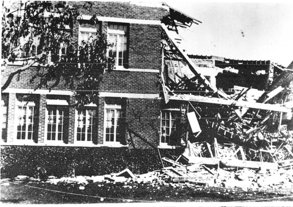
FIGURE 14. Collapsed roof and walls of Jefferson Junior High School building following the March 10, 1933 Long Beach, California earthquake ( M_L = 6.3 ). (Photo by Captain T. J. Maher. Courtesy of the National Oceanic and Atmospheric Administration, Environmental Data Service.)
