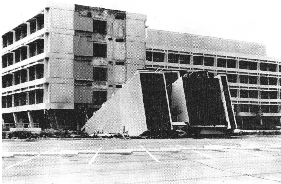
FIGURE 15. The Medical Treatment and Care Unit of the Olive View Community Hospital complex in Sylmar, California following the February 9, 1971 San Fernando earthquake ( M_L = 6.4 ). Three of four stair well and recreation towers overturned and pushed into the basement. Note the damage to first-story columns. There were three casualties at this facility. One person was killed as a direct result of the earthquake, and two people under intensive care died when an earthquake-caused power failure severed the operation of all electrical life-support systems. (Courtesy of James L. Ruhle and Associates, Fullerton, Calif.)
