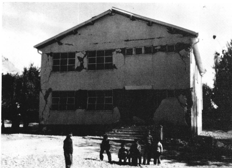
FIGURE 36. West-wall view of an unreinforced masonry high school building in Lice following the September 6, 1975 Lice, Turkey earthquake ( M_s = 6.7 ). All lateral resisting elements were shattered. Similar damage occurred to an adjacent high school building of identical construction. (Courtesy of Peter I. Yanev; URS/John A. Blume & Associates, San Francisco.)
