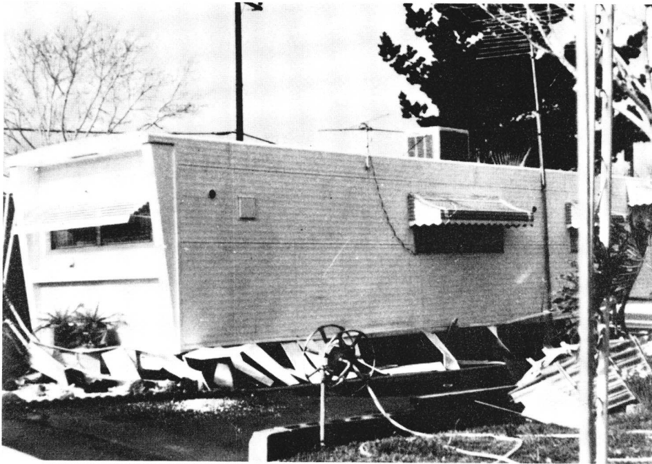
FIGURE 26. Mobile home in the San Fernando Valley shifted off its foundation by the February 9, 1971 San Fernando, California earthquake ( M_L = 6.4 ). Note damage to the aluminum skirting. (Photo by Drew P. Lawrence; courtesy of National Oceanic and Atmospheric Administration, Environmental Data Service.)
