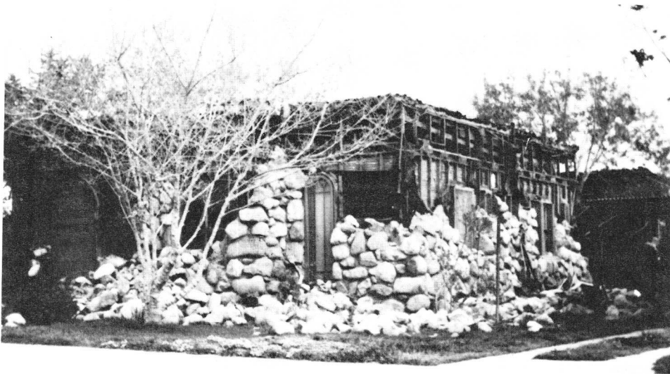
FIGURE 24. Severely damaged older wood-frame dwelling with unanchored stone veneer in San Fernando following the February 9, 1971 San Fernando, California earthquake ( M_L = 6.4 ). (Courtesy of National Oceanic and Atmospheric Administration, Environmental Data Service.)
