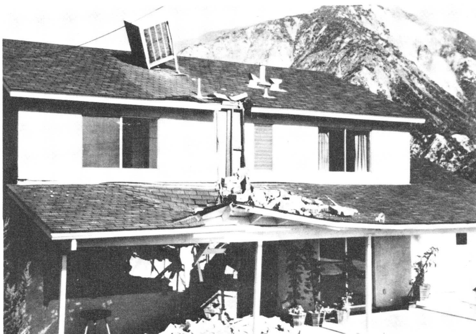
FIGURE 25. Severely damaged chimney and roof-mounted evaporative cooler at a residence in the San Fernando Valley following the February 9, 1971 San Fernando, California earthquake ( M_L = 6.4 ). (Los Angeles City Department of Building and Safety photograph; courtesy of National Oceanic and Atmospheric Administration, Environmental Data Service.)
