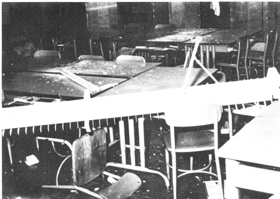
FIGURE 28. Pendant-mounted light fixtures that were torn loose from their ceiling support base plates at the Herrick Avenue Elementary School during the February 9, 1971 San Fernando, California earthquake ( M_L = 6.4 ). (Los Angeles City Department of Building and Safety photograph; courtesy of National Oceanic and Atmospheric Administration, Environmental Data Service.)
