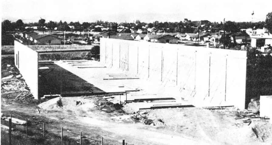
FIGURE 14. Precast, tilt-up concrete building under construction in Los Angeles, California. (Courtesy of James L. Ruhle and Associates, Fullerton, Calif.)
