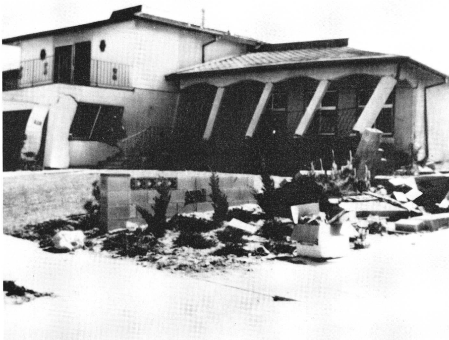
FIGURE 23. Partially collapsed garage section of modern split-level dwelling in Sylmar following the February 9, 1971 San Fernando, California earthquake ( M_L = 6.4 ). (Courtesy of National Oceanic and Atmospheric Administration, Environmental Data Service.)
