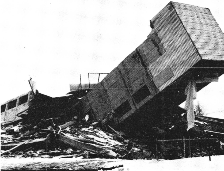
FIGURE 12. Collapsed Four Seasons apartment building in Anchorage following the March 27, 1964 Alaskan earthquake ( M_s = 8.5 ). An adjacent two-story wood-frame building was undamaged. 947 (From Berg, G. V. and Stratta, J. L., Anchorage and the Alaska Earthquake of March 27, 1964 , American Iron and Steel Institute, New York, 1964, 20. With permission.)
