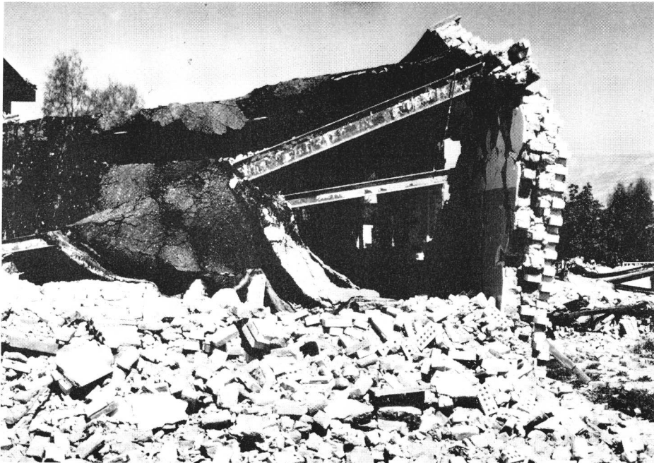
FIGURE 31. The steel beam masonry Malaria Eradication Center building in Ghir following the April 10, 1972 Fars Province, Iran earthquake ( M_s = 6.9 ). Note the absence of reinforcing steel in the bearing wall. (Courtesy of James W. Dewey, U.S. Geological Survey.)
