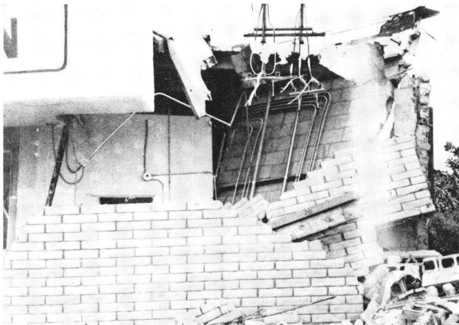
FIGURE 17. Collapsed southeast corner of Stone's Liquor Store in Sylmar following the February 9, 1971 San Fernando, California earthquake ( M_L = 6.4 ). The building was constructed in 1969; it had a plywood roof and reinforced hollow concrete walls. Structural failures could have been caused by a severing of the roof-to-wall connection when the bearing walls were subjected to ground accelerations normal to their planes. The ability to resist lateral loading along the south elevation may have been further impaired because the vertical reinforcement did not appear to extend more than 1.8 m above the floor, thus leaving the top portion of the wall unreinforced. Portions of other walls with reinforcing steel did not appear to contain grout. This building, valued at $35,000 prior to damage, had to be demolished shortly after the earthquake. 977 (Courtesy of National Oceanic and Atmospheric Administration, Environmental Data Service.)
