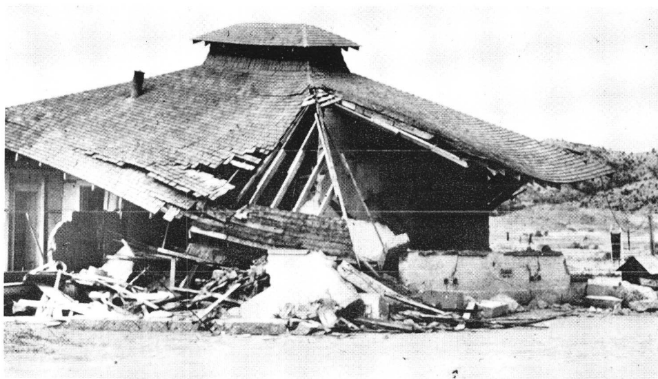
FIGURE 5. Collapsed Cummings Valley School following the July 21, 1952 Kern County, California earthquake ( M_L = 7.7 ). The school, built about 1910, 948 was constructed of reinforced concrete walls and wood roof. (Courtesy of National Oceanic and Atmospheric Administration, Environmental Data Service.)
