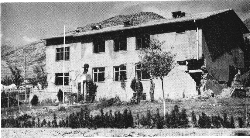
FIGURE 35. Unreinforced masonry police building in Lice following the September 6, 1975 Lice, Turkey earthquake ( M_s = 6.7 ). Note the severe damage to the first floor corner of the building, the shear failure of the piers between the windows, and the toppled brick chimneys. (Courtesy of Peter I. Yanev; URS/John A. Blume & Associates, San Francisco.)
