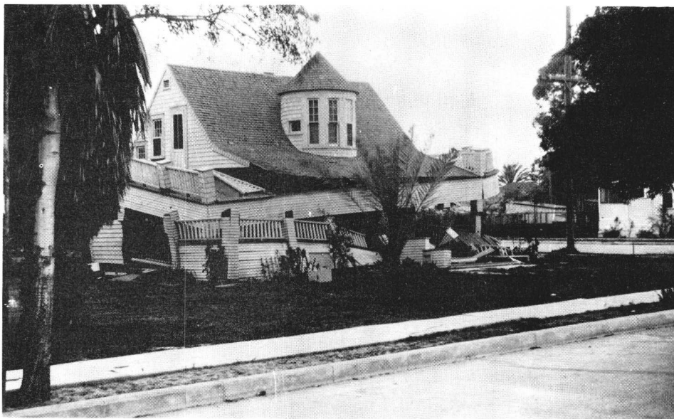
FIGURE 3. Wood-frame house severed from its foundation as a result of March 10, 1933 Long Beach, California earthquake ( M_L = 6.3 ). The studding had been weakened by termites. (Photo by Mr. Merritt; courtesy of National Oceanic and Atmospheric Administration, Environmental Data Service.)
