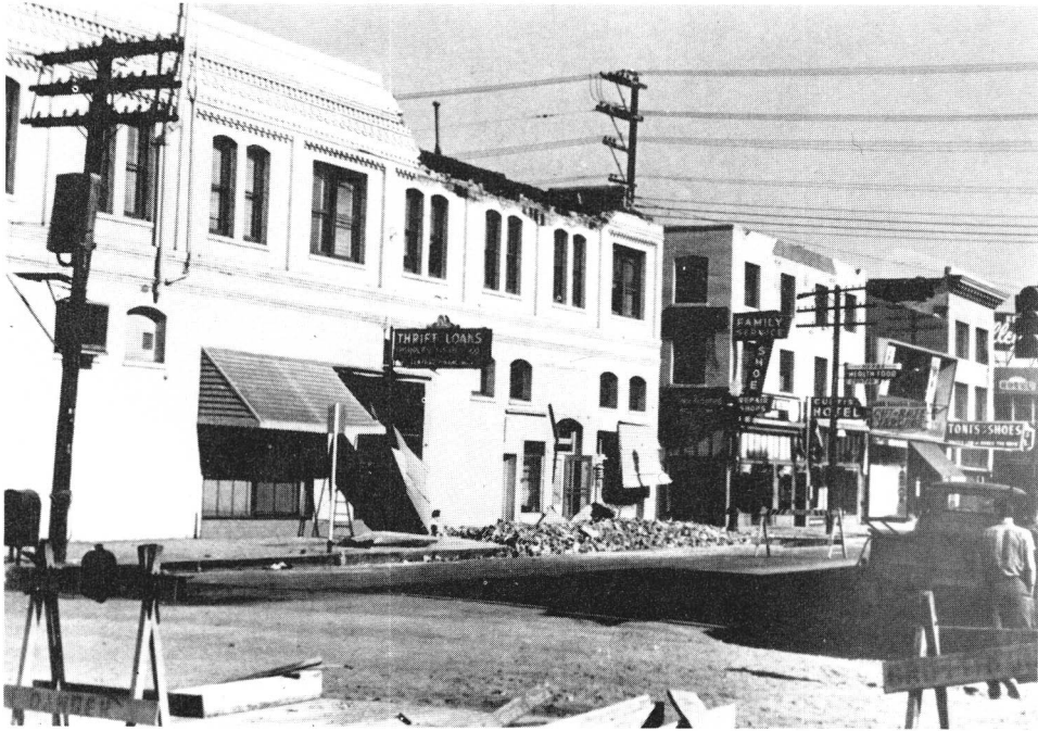
FIGURE 10. Parapet damage to structures in Bakersfield, California following the July 21, 1952 Kern County earthquake ( M_L = 7.7 ). (Courtesy of the National Oceanic and Atmospheric Administration, Environmental Data Service.)
