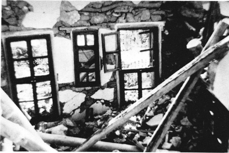
FIGURE 38. Interior view of a traditional stone dwelling in Lice showing collapsed timber and mud roof following the September 6, 1975 Lice, Turkey earthquake ( M_s = 6.7 ). (Courtesy of Peter I. Yanev; URS/John A. Blume & Associates, San Francisco.)
