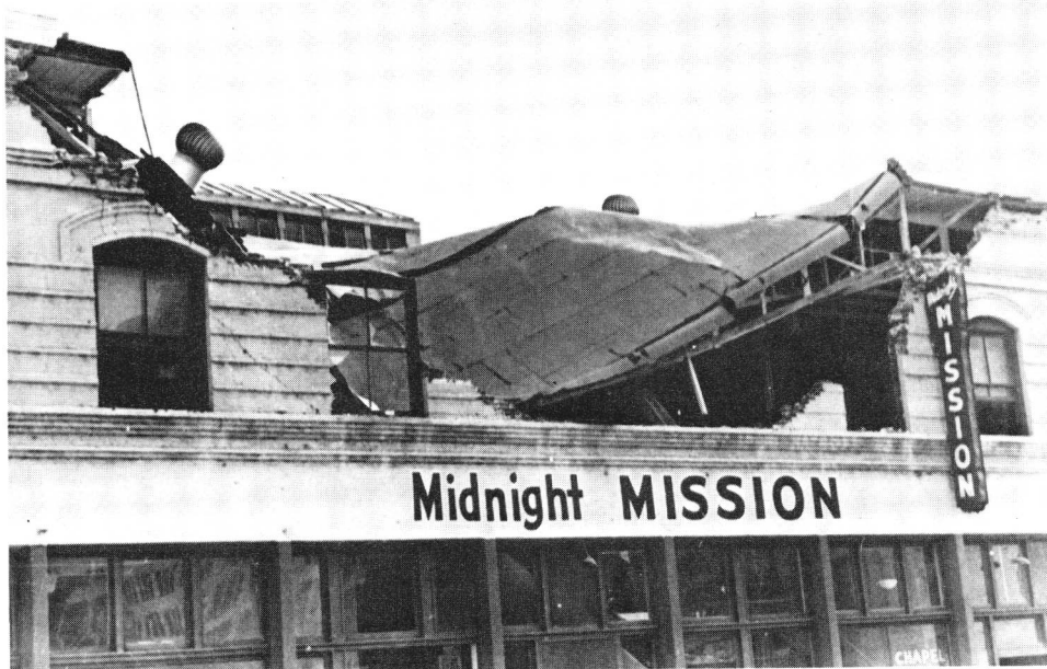
FIGURE 21. Front elevation of the unreinforced masonry Midnight Mission building in downtown Los Angeles showing partial collapse of a room and second-story wall following the February 9, 1971 San Fernando, California earthquake ( M_L = 6.4 ). Although only a 6.1-m portion of the second story wall fell, the remainder of the wall was displaced outward from 2.5 to 5.0 cm; further movement and collapse probably were prevented by the joist anchors installed as a part of the Los Angeles parapet correction program (described in Volume II, Chapter 3). One resident ran from the building at the beginning of the earthquake and was killed by falling bricks. 970 (Los Angeles City Department of Building and Safety photograph; courtesy of National Oceanic and Atmospheric Administration, Environmental Data Service.)
