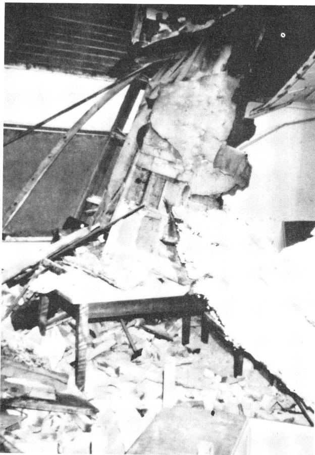
FIGURE 20. Classroom at Los Angeles High School following the February 9, 1971 San Fernando, California earthquake ( M_L = 6.4 ). Portion of a parapet wall fell through the classroom roof. (D. K. Jephcott photograph; courtesy of National Oceanic and Atmospheric Administration, Environmental Data Service.)
