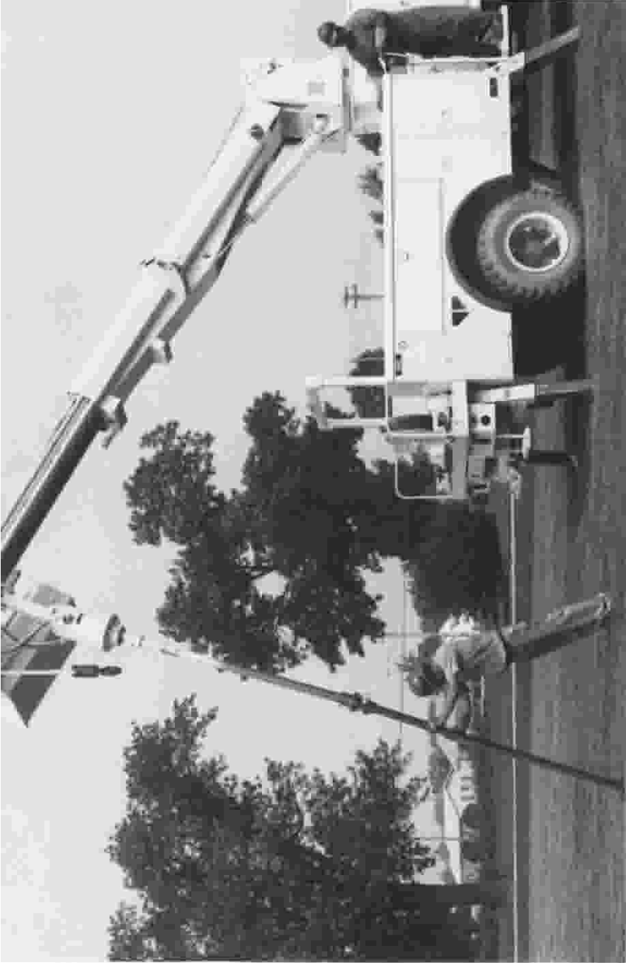
Figure 1-11 Photograph of installation of helical anchor (courtesy of A. B. Chance Co., Centralia, Missouri, USA)
