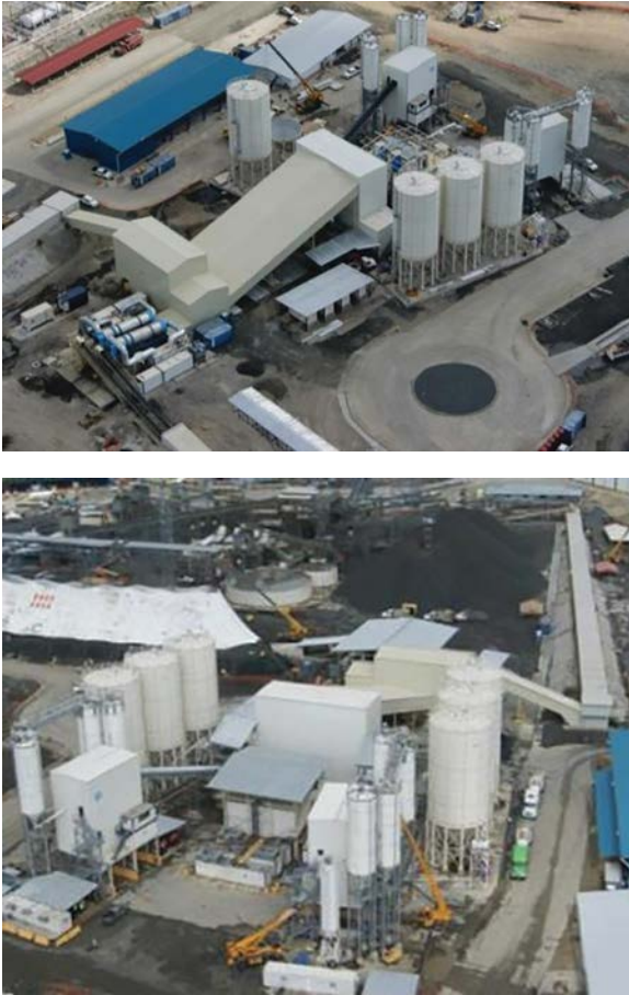
Figure 10.13 View of the Pacific concrete plant for the new Panama Canal, with the silos and the refrigeration plant.
