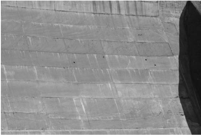
Figure 4.13 Efflorescence on downstream face of a dam at Ocean Falls, British Columbia; the dam was constructed in 1925. (Courtesy of S. Mindess.)
