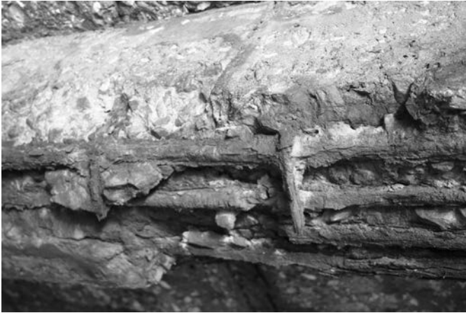
Figure 4.16 Pitting corrosion. (Courtesy of H. Beushausen.)
