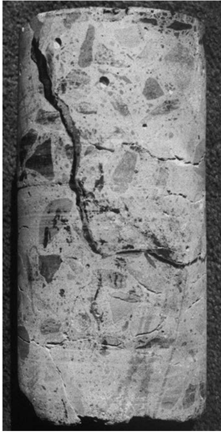
Figure 4.10 AAR-induced cracking representing a macrocrack, which may allow further deterioration to occur (core diameter 100 mm).
