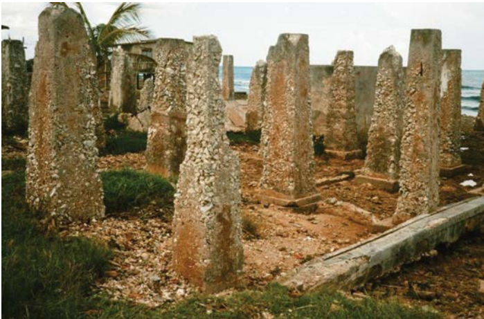
Figure 4.14 Damage due to salt crystallization of concrete columns after about 1 year. (Courtesy of S. Mindess.)
