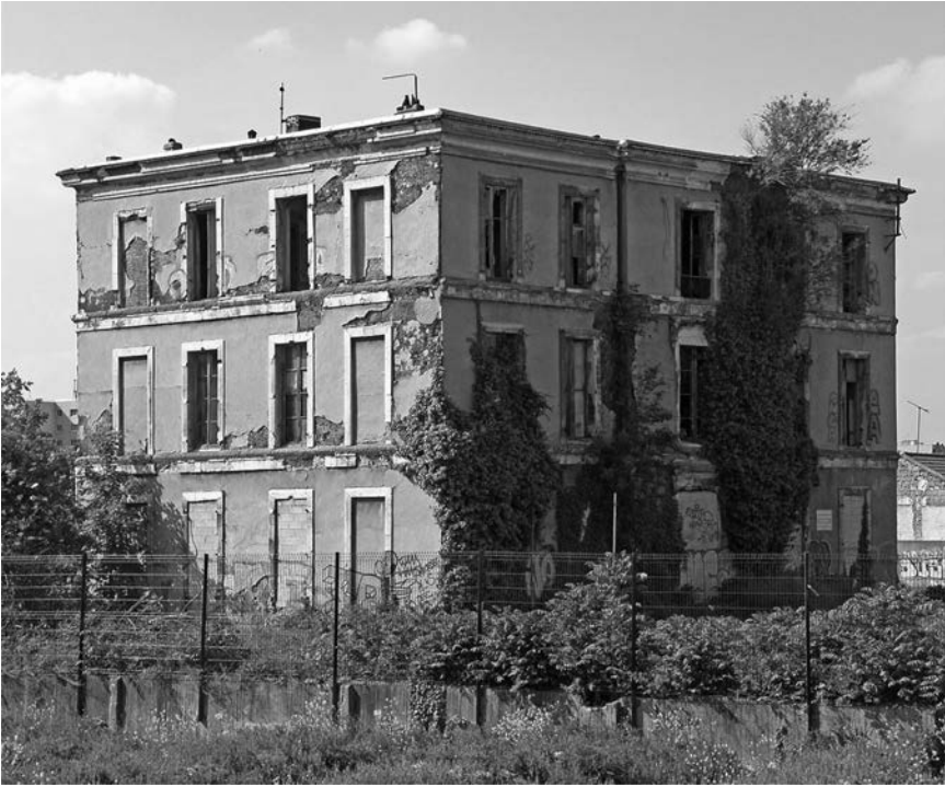
Figure 1.6 First house built with reinforced concrete, by Francois Coignet, Paris, 1853; now in a state of serious disrepair. (Courtesy of Bajart, E., 2010, Maison de Francois Coignet , available at: http://commons.wikimedia.org/wiki/File%3AMaison_Fran%C3%A7ois_Coignet_2.jpg , accessed on February 27, 2016.)
