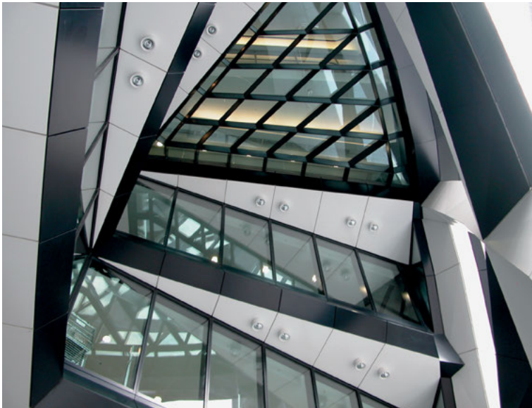
A view from exterior grade up through the triangular shafts. The extreme level of care in the design and fabrication of the multiple cladding systems is evidenced by the coordination of the sizing and joint lines of the systems that converge in this detail.
