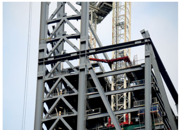
The exposed structure of The Leadenhall Building made use of intumescent fire protection to permit its structure to be expressed as part of its double façade system.
