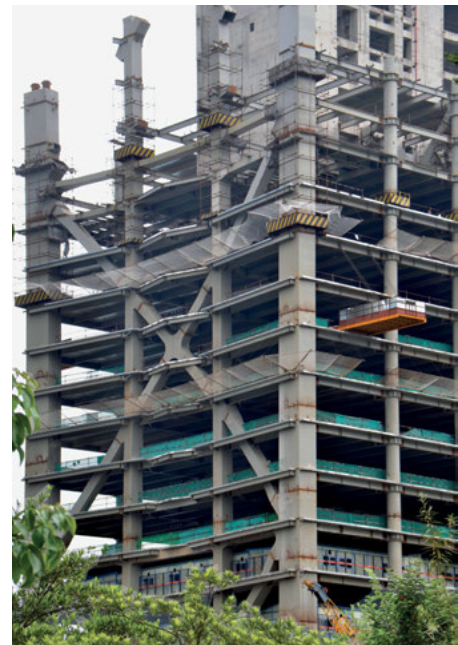
Guangzhou Fortune Center is a diagonalized core building in Guangzhou, China. This image of the future 309m/1,015ft Supertall, under construction in 2012, illustrates the use of custom box sections that will be filled with concrete to create the steel structure, which is a very common construction method in China. The splices on the columns and diagonals are welded. The structure will be concealed. The core is reinforced concrete.
