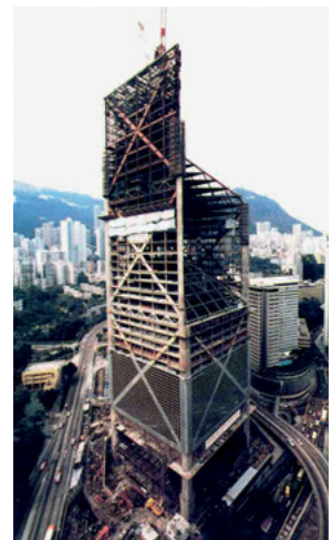
This image of the Bank of China Tower in Hong Kong under construction in 1988 was originally published by Engineering News Record in a discussion of the merits of the composite construction system. The hierarchy of the members and the relationship of the large diagonals to the stabilization of the system is evident.
