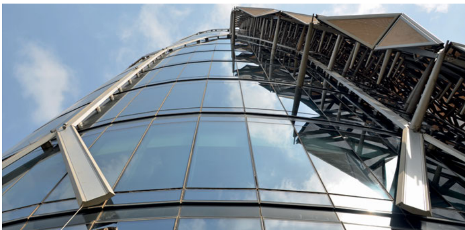
The rectilinear curtain wall of the Al Bahar Towers is installed continuously. The banding that highlights the location of the honeycomb structure sits proud of the curtain wall. It is fitted with an LED lighting system to showcase the structure of the towers at night.
