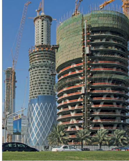
This construction image of the Tornado Tower (left) reveals that the rectilinear curtain wall has been installed continuously and that the bright bands highlighting the placement of the diagrid behind have been installed in front of the curtain wall. At the right is the Doha Tower under construction, its diagrid concealed by the mashrabiya screen that is erected over the curtain wall to provide shading.
