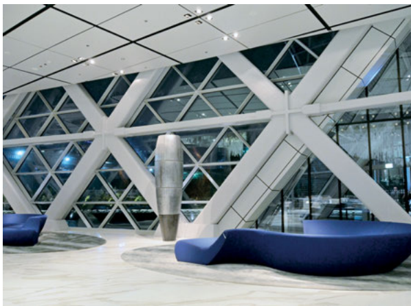
Intumescent fire protection is used on the architecturally exposed steel structure of Capital Gate. The expression of the members and their connections is a very important aspect of the design and so an intumescent coating was the applicable choice.
