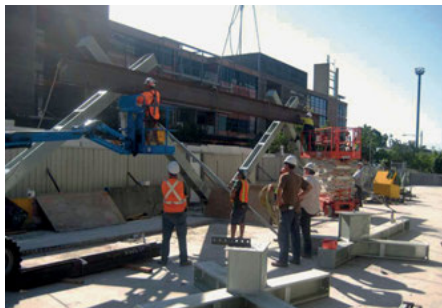
One Shelley Street in Sydney, Australia, designed by Fitzpatrick + Partners with Arup, was designed with constructability and safety as a premier concern. The part of prefabrication work was maximized. The majority of diagrid connections were made by bolting. The amount of work done at height was minimized.
