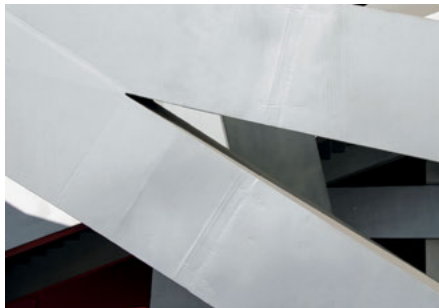
The Beijing National Stadium (Bird's Nest) in Beijing, China, designed by Herzog & de Meuron/Ai Weiwei/Arup, used custom-fabricated square sections that were welded on site. The temporary bolting tabs were removed and ground. Although traces of the connections are visible in some lighting conditions, the scale of the project is such that the final product is more than sufficient in quality.
