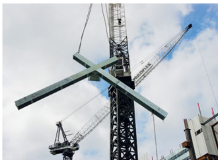
The X-nodes and two diagrid elements for One Shelley Street were preassembled in the staging area, making the erection simpler and limiting the work done at height. Steelwork was completed by Bluescope.
