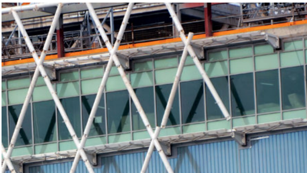
A close view of the installation of the diagrid double façade system at the Cleveland Clinic in Abu Dhabi, UAE, designed by HDR Architecture. Special discreet bolted connections have been designed to make for both a detail and quick erection. The connection is recessed to preserve the clean visual lines of the white diagrid. The system is braced back to the primary structure to complete the triangulation. This results in a two-storey diamond module. The diagrid is separated from the building to allow for cleaning access via the catwalk that also acts as a shading strategy. A fairly standard curtain wall system sits behind the outer double façade layer.
