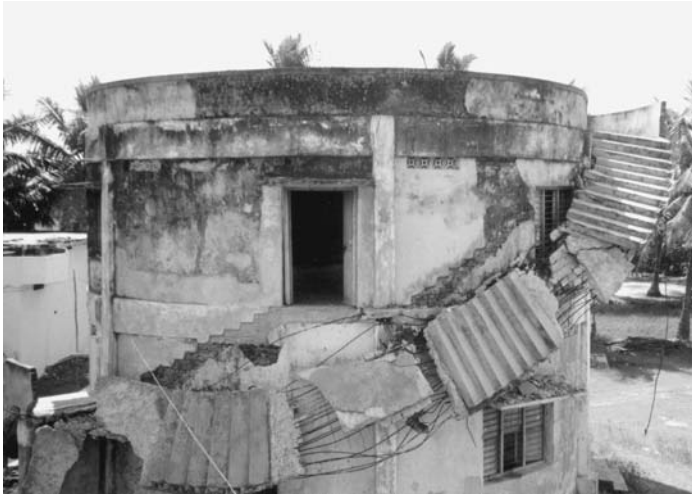
Figure 12.3 Another example of a poorly constructed cyclone shelter and community centre. This cyclone shelter in East Godavari, is another example of an important local asset that has been made redundant through poor construction practices, inadequate materials and little or no maintenance.
