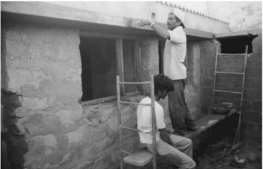
Figure 3.5 Self-help intervention. A self-help structure is being constructed in Bhuj using stones and concrete blocks, without employing any earthquake-resistant features.
