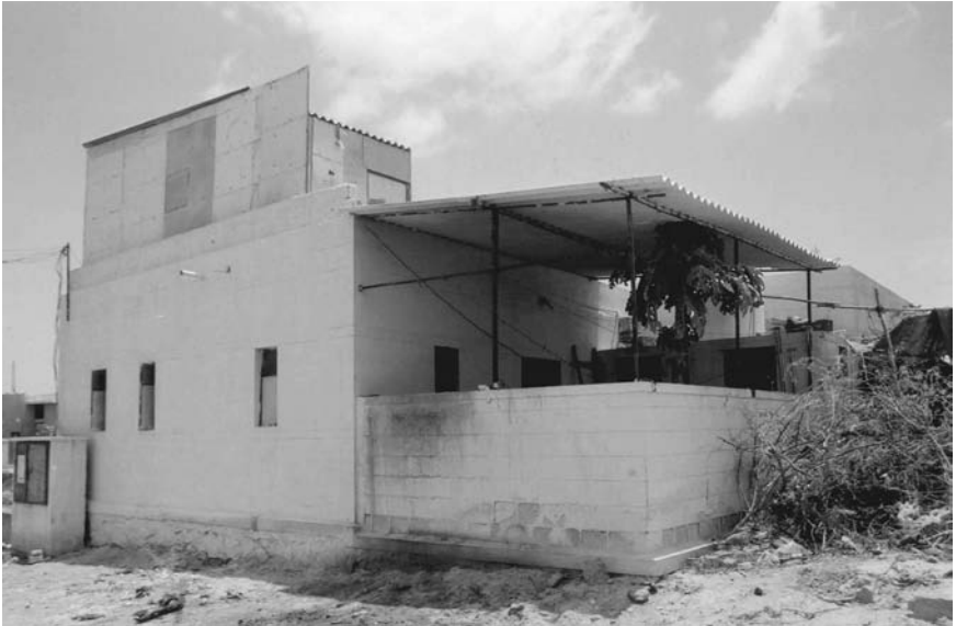
Figure 3.4 Temporary structures in Bhuj. A temporary structure has been added on top of a reconstructed structure in the relocated urban colony in Bhuj, along with other additions.
