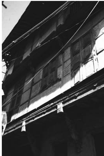
Figure 3.6 Traditional structures in Limbdi. One of the surviving traditional structures in Limbdi town has earthquake-safe qualities due to its timber-framed construction with masonry infill.
