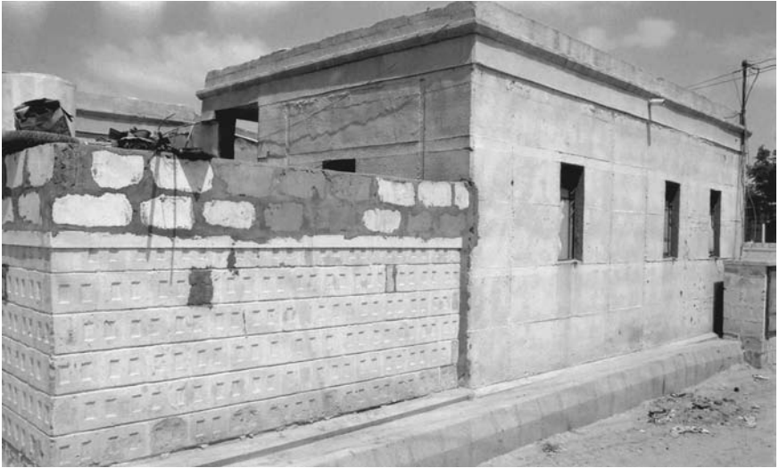
Figure 3.2 Piecemeal additions made to the reconstructed structures. These additions, using various materials such as clay blocks and stones, increase their vulnerability to earthquakes. Bhuj, Gujarat.
