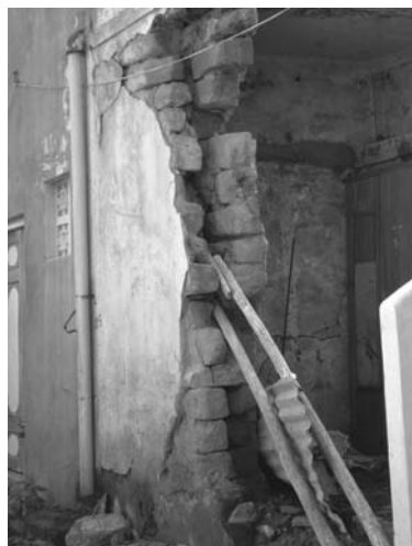
Figure 3.1 Poorly constructed stone masonry structures. This building in Limbdi collapsed during the February 2001 Gujarat earthquake.
