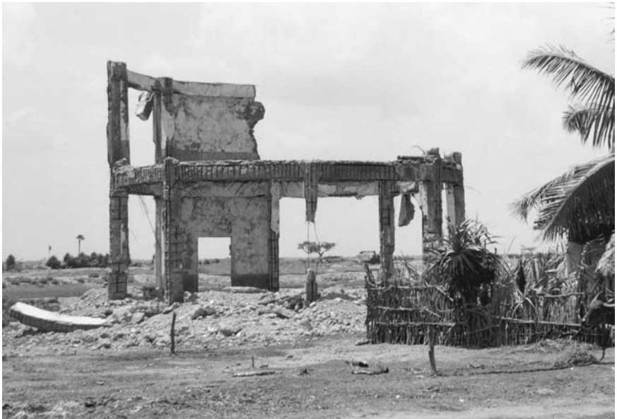
Figure 12.2 Shell of cyclone shelter devastated by poor construction, inappropriate materials and inadequate maintenance. A cyclone shelter in East Godavari, Andhra Pradesh that was built during 1997 in the aftermath of a tropical cyclone that affected the village the previous year; the photograph was taken in July 2001. The cyclone shelter was not destroyed by an extreme natural event but by poor construction practices, inadequate materials and little or no maintenance, and is testament to the problems associated with the hasty construction of built assets.
