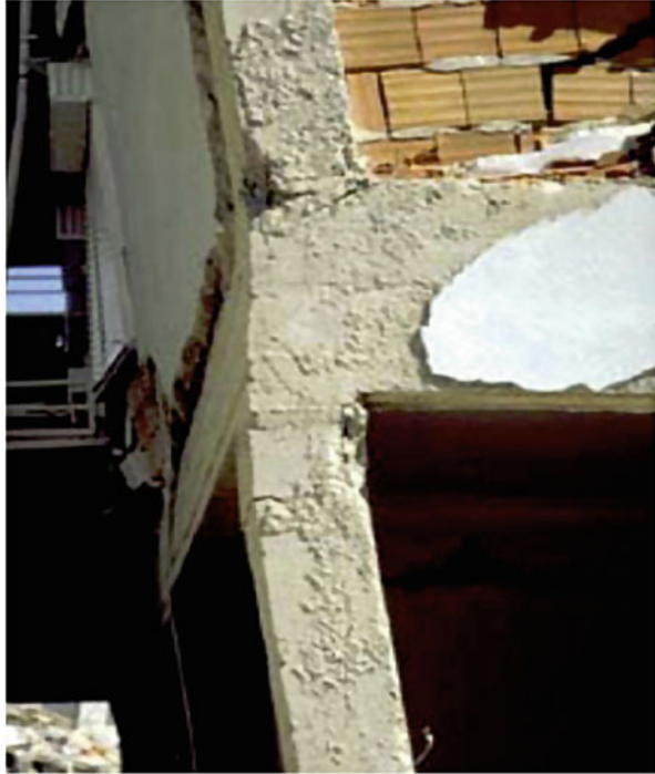
Fig. 2.14 Moment frames: consequences of non-compliance with the “strong columns – weak beams” rule
