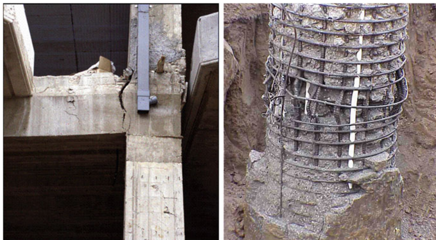
Fig. 1.11 Flexural damage observed at the end of a beam and at the base of a column
