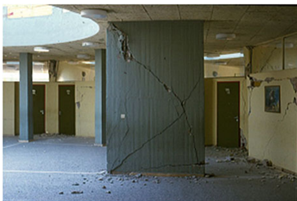
Fig. 1.4 Requirement for major level earthquakes: damage to structural elements is accepted, yet collapse probability must remain sufficiently low
