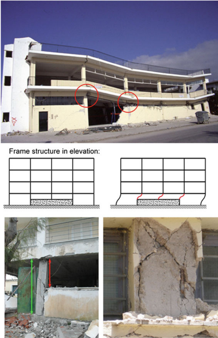
Fig. 2.3 Short column due to ex post masonry infill walls ( left ) and to initial architectural facade requirement ( right )
