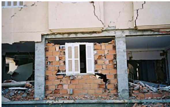
Fig. 1.3 Requirement for moderate level earthquakes: damage to non-structural in-fill walls is acceptable, yet only minor, repairable damage to structural elements is permitted
