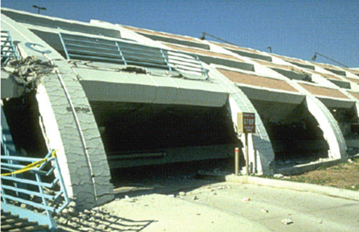
Fig. 1.13 Structural collapse of a parking station during the Loma Prieta earthquake (source: http://ghestalt.egloos.com/2530520 )
