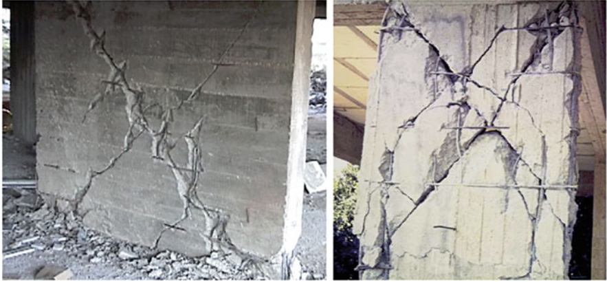
Fig. 2.18 Brittle shear failure of r/c walls at the ground floor of buildings to be avoided
