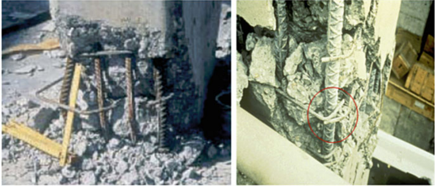
Fig. 2.11 Examples of premature column failures due to opening-up of inadequately end-detailed hooks
