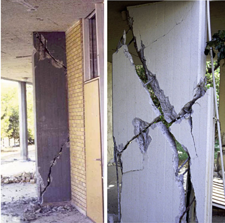
Fig. 2.12 Brittle (shear) failure due to inadequate lateral reinforcement
