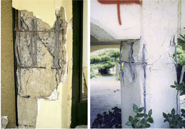
Fig. 2.9 Longitudinal steel bar buckling and concrete cover spalling due to inadequate sparse spacing of stirrups
