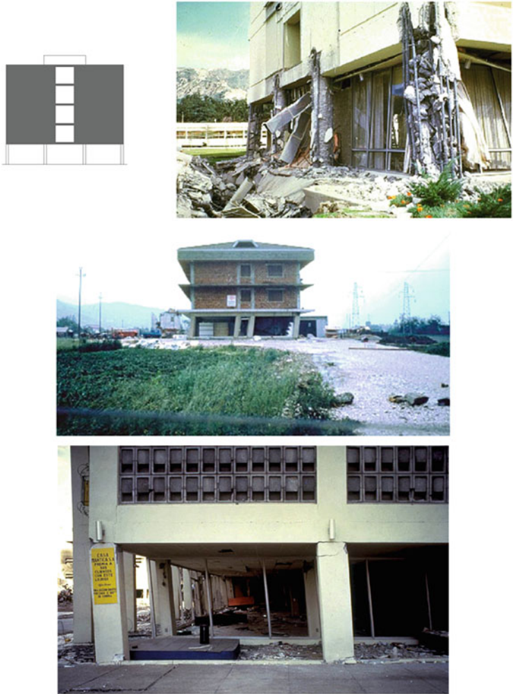
Fig. 2.4 Soft storeys (pilotis): r/c walls supported by columns and moment frames with no infills in the ground floor
