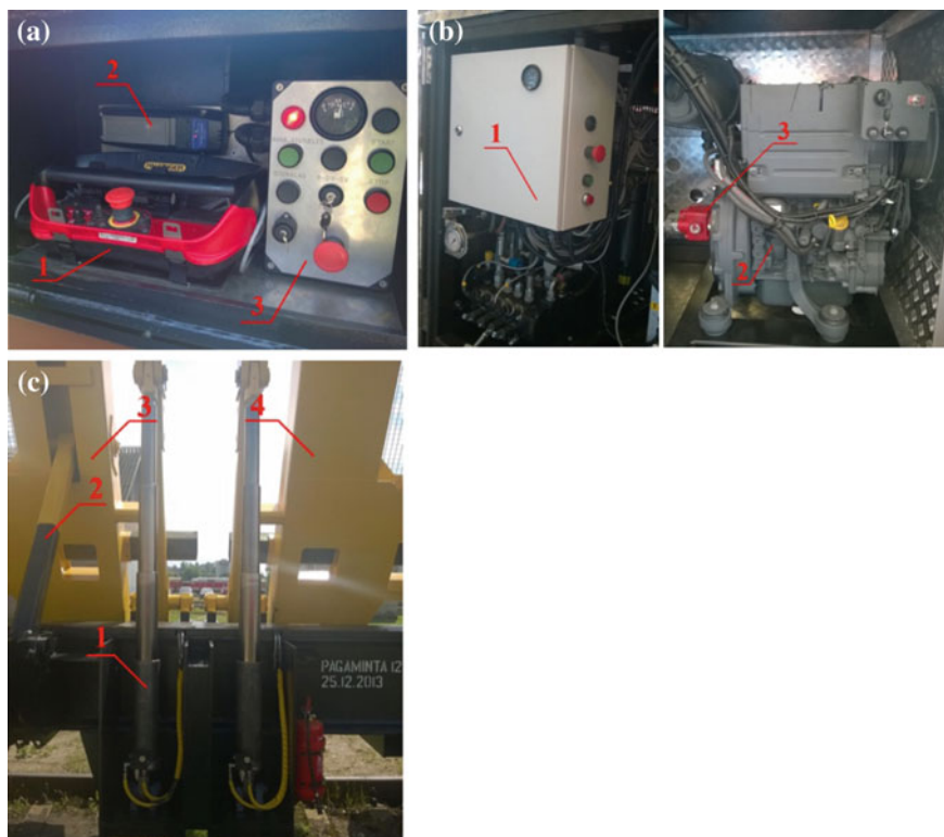
Fig. 69 Control equipment of platform MPP-61. a Designations: 1—remote controller of platform MPP-61; 2—transmitter of the remote control system; 3—manual control panel. b Designations: 1—electrical cabinet; 2—diesel engine; 3—hydraulic pump. c Designations: 1—hydraulic cylinder; 2—support; 3—part A of tilt platform; 4—part B of tilt platform
