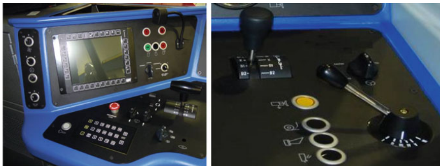
Fig. 27 Control panel with automatic speed regulation keyboard of the TEM LTH diesel-electric locomotive
