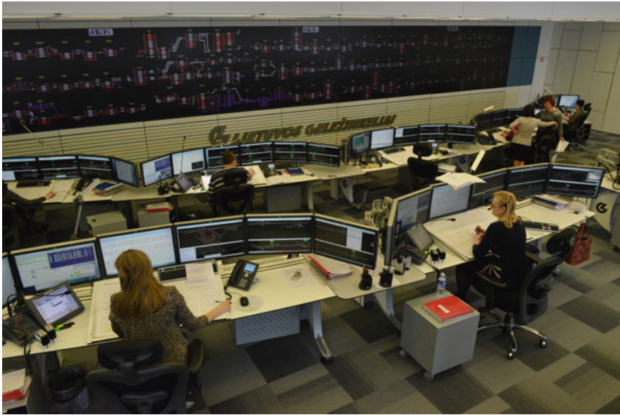
Fig. 52 A photo of a new LG traffic control center
