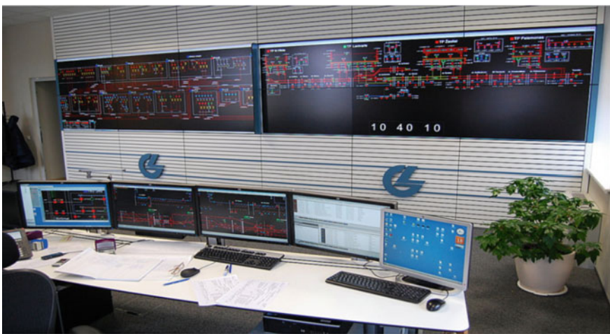
Fig. 53 A photo of LG contact network equipment remote control
