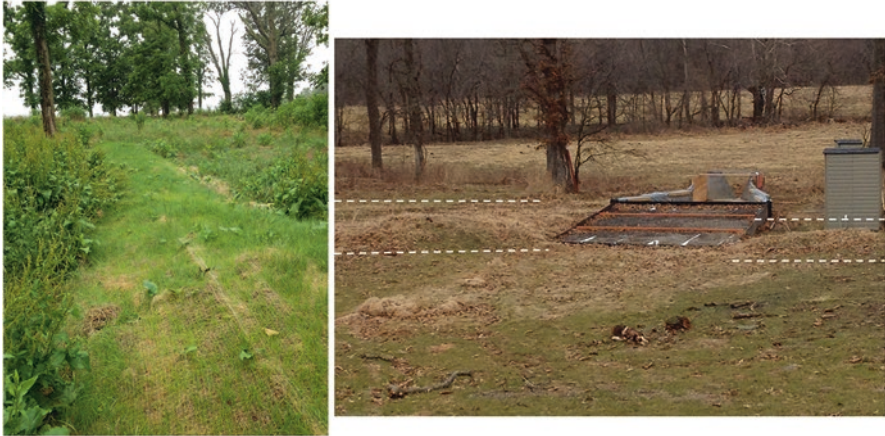
Fig. 3.5 The earthen berms in the left photograph were constructed to channel water into the entrance of the P removal structure ( right photo ). View in the right photo is from the uphill side looking downward into the direction of water flow. Berms are highlighted between the dashed lines . Photo credit: Stuart Wilson, TLDR consulting.
