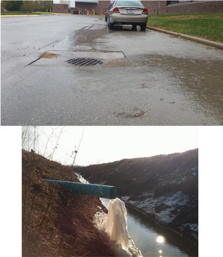
Fig. 3.4 Storm water drop inlets in urban areas and subsurface drainage lines represent areas where water flow is concentrated and therefore a potential location for a P removal structure if the dissolved P concentrations are elevated. Lower photo is courtesy of Stan Livingston, USDA-ARS
