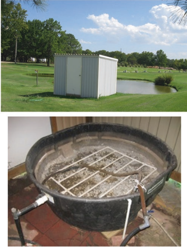
Fig. 3.13 Pond filter style P removal structure. This type of P removal structure is more costly if a pump is needed. Water from the pond is pumped into the building ( upper photo ), which contains a bed of PSMs ( lower photo ). The water drains through the PSMs, allow dissolved P to sorb to them, and drains back via gravity to the pond. Treating ponds is generally not recommended unless the dissolved P concentrations are very high. Photo credit: Chad Penn, USDA-ARS
