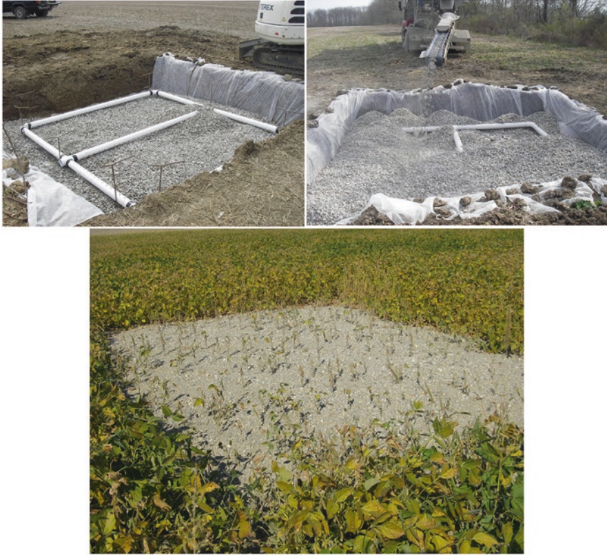
Fig. 3.15 Surface inlets for tile drainage can serve as P removal structures if constructed using a PSM. The surface inlet is constructed in a low spot where the surface runoff collects within a field. The frame of subsurface drainage pipe, which is ultimately plumbed into a tile drain pipe, is back-filled with an aggregate. Photo credit: Stan Livingston, USDA-ARS
