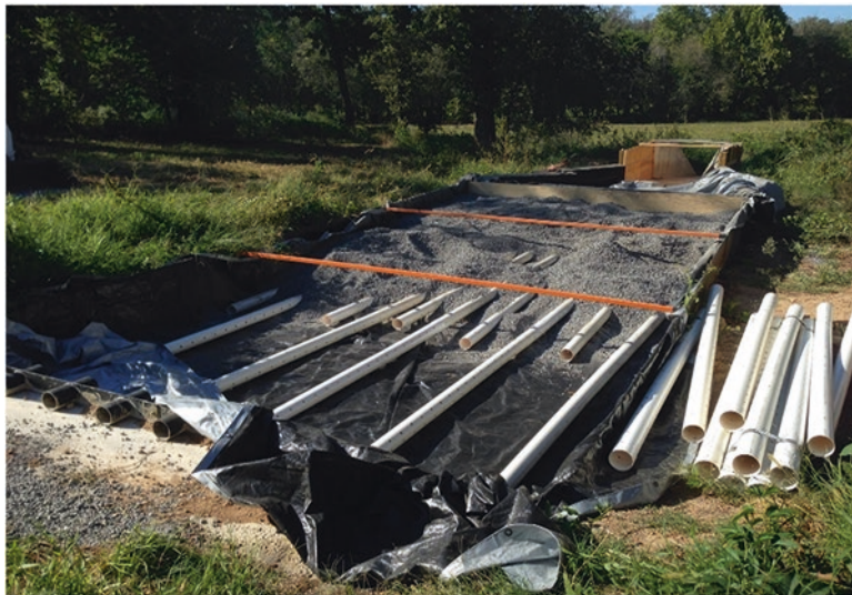
Fig. 6.7 The subsurface drainage layer of a P removal structure was exposed prior to the addition of the PSM. The drainage layer consisted of 4 in. (10.16 cm) diameter perforated PVC pipes
