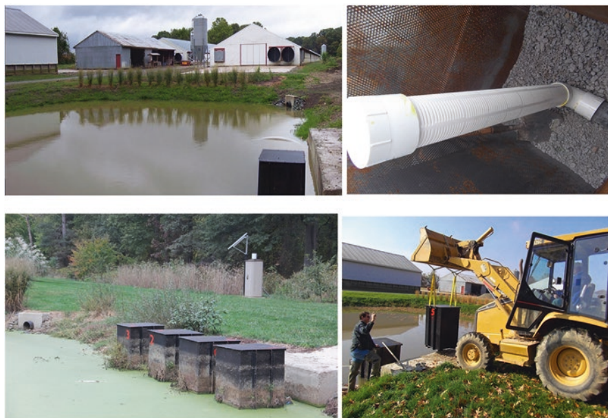
Fig. 3.8 Modular Box style P removal structure constructed on a poultry farm. Upper photo shows the poultry farms and the basin/pond in which all runoff flows into. The water in the pond can only exit by flowing through the perforated metal boxes shown in the bottom left photo . The perforated metal boxes are removable and inside consists of a perforated pipe and the PSM. Upper right photo shows the inside of the box before being completely filled with PSM. The perforated pipe is plumbed to a drain that carries the treated water to a nearby drainage ditch. Photo credit: Josh McGrath, University of Kentucky
