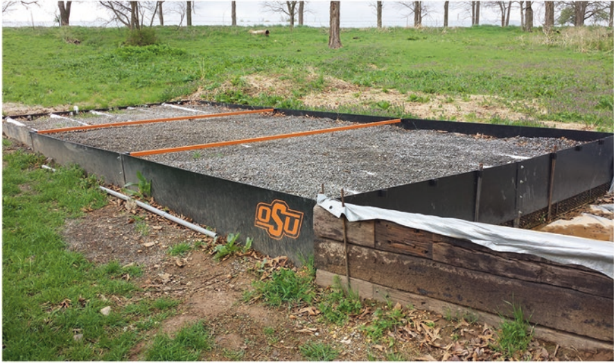
Fig. 2.14. Example of a P removal structure that treated runoff from a poultry CAFO. High P water flowed into the structure on the upslope side, where it filtered through the contained PSM (treated steel slag) and drained out on the other side. This structure removed about 3 lb of dissolved P per year while it was monitored (2.5 years). Structures can be designed to achieve desired P removal targets and lifetimes
