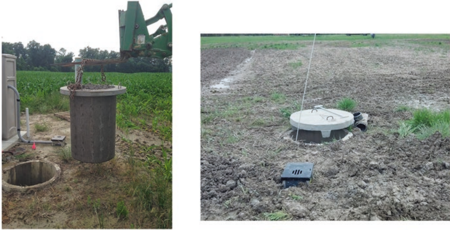
Fig. 3.12 Example of a large cartridge style P removal structure for treating surface drainage. This large PSM cartridge treats surface runoff that flows into it, and is easily removed and replaced with a front-end loader or excavator. This particular style of P removal structure is ideal for surface inlets in urban areas. Photo credit: upper photographs - Josh McGrath, University of Kentucky; lower photographs - Barry Husk, Blue Leaf
