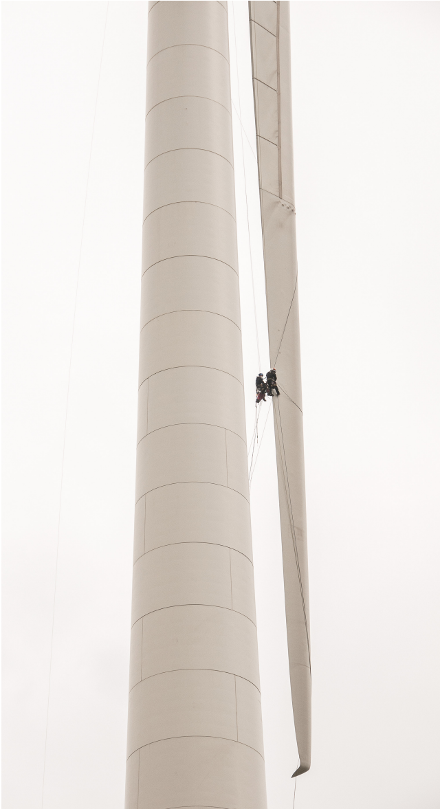
Fig. 6.1 Implementation of maintenance strategies requires courage, in particular at offshore sites
