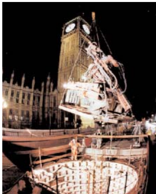
Fig 10.7 Drilling rig lowered into shaft for installation of TAMs beneath the Big Ben Clock Tower © AMEC
