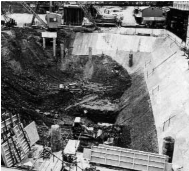
Fig 4.9 Britannic House, London: North diaphragm wall after bulk excavation and before excavation for struts
