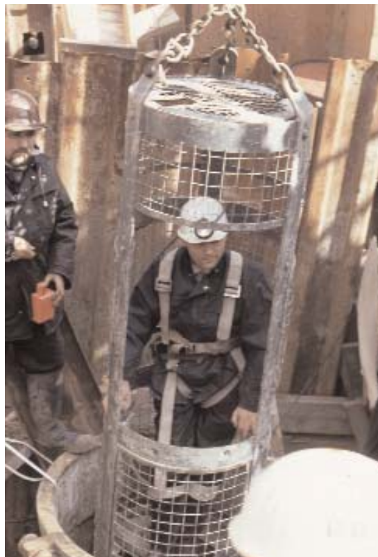
Fig 1.1 Ground profile exploration being carried out for the foundations and deep basement of the YMCA, London in the mid-seventies. Present requirements for the descent of augered shafts are covered by BS 8008:1996.
