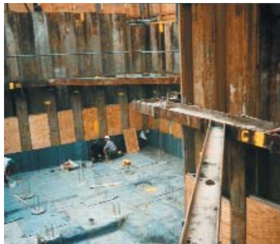
Fig 11.6 Water resisting membrane construction on a sheet pile wall for a deep basement
