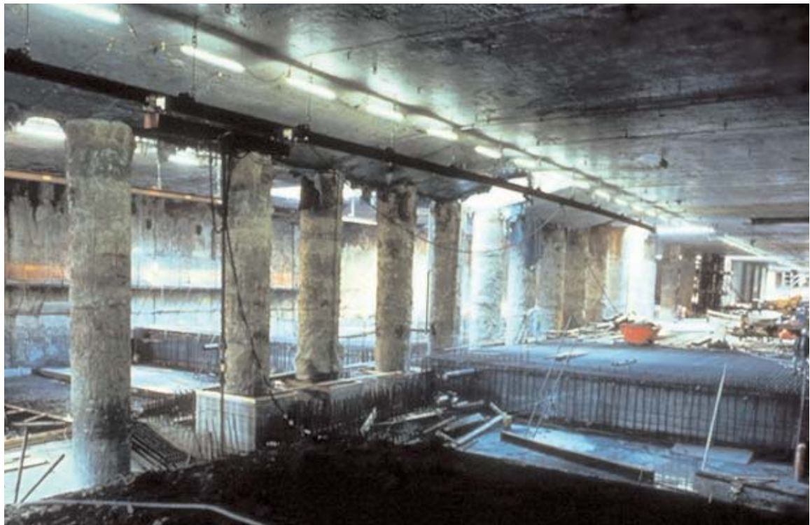
Fig E.3 Results of value engineering: omission of struts by using the OM, temporary roof support and lighter slabs © Benaim
