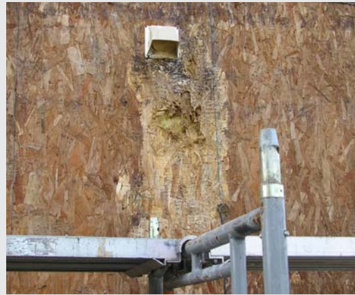
Figure 2.1-C Damage from Failure at Vent Penetration
