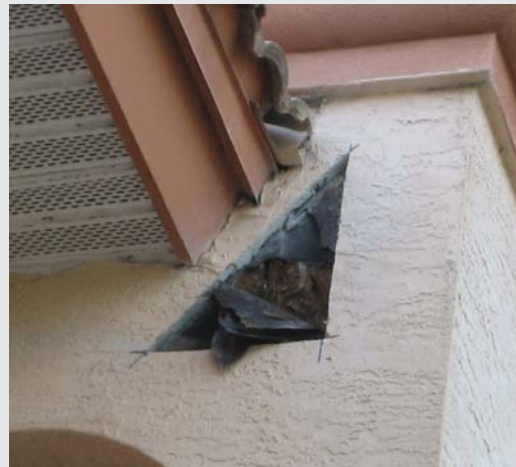
Figure 2.1-E Damage from Failure of the Roof Flashing Termination
