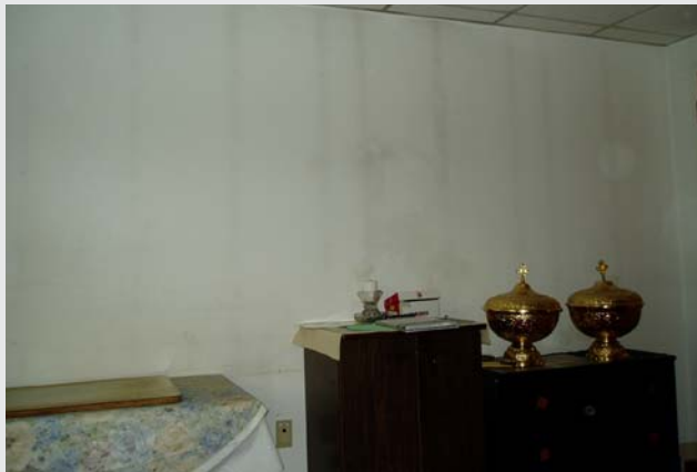
Figure 2.2-D Ghosting of Steel Studs on Walls Photograph copyright Wiss, Janney, Elstner and Associates, Inc.
