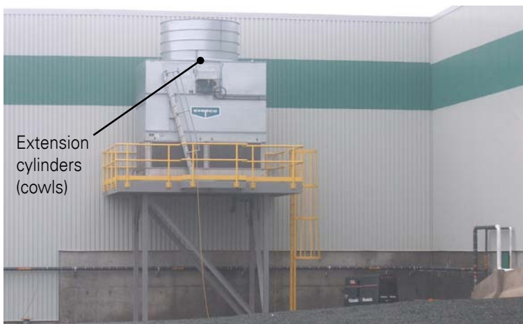
Figure 3.2-C Cooling Tower with Too Few Extension Cylinders (Cowls) Added to the Exhaust Plume Photograph copyright Evapco, Inc.
