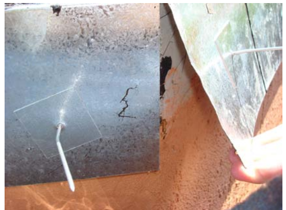
Figure 2.1-K Slab Foundation Example 2 Photograph copyright Liberty Building Forensics Group®.
