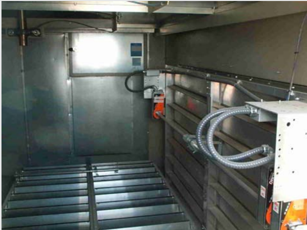
Figure 7.2-H Minimum Outdoor Air Dampers (to the Right) and Return Air Dampers (at the Bottom)
