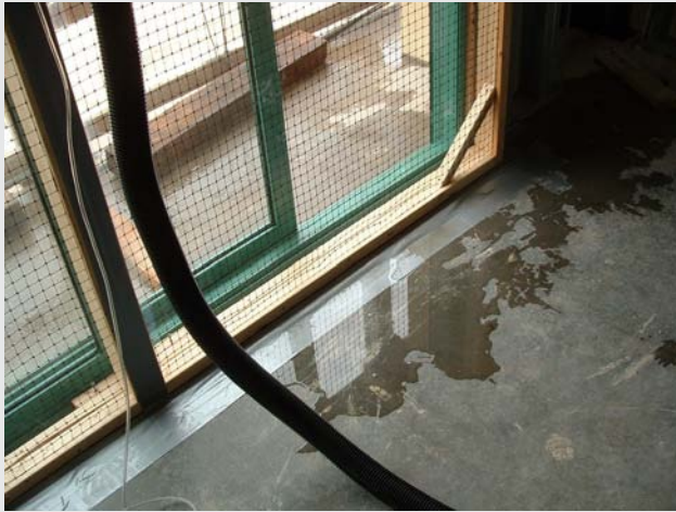
Figure 1.2-J Water Leakage Failure—Early Test Unit Photograph courtesy of Dave MacPhaul; copyright CH2M HILL.
