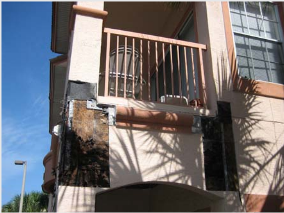
Figure 2.1-B Structure Damage from Failures in the Building Envelope
