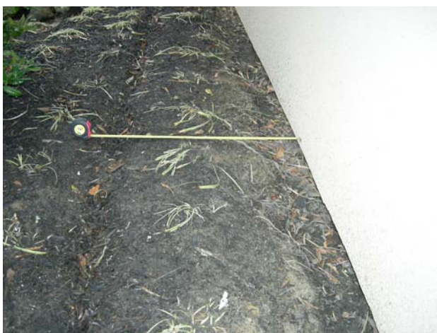
Figure 2.1-I Grade Example 2 Photograph copyright Liberty Building Forensics Group®.
