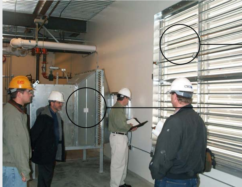
Figure 7.2-A Minimum Outdoor Air Fan and Main Outdoor Air Dampers of a Build-Up HVAC System Photograph courtesy of Leon Alevantis.
