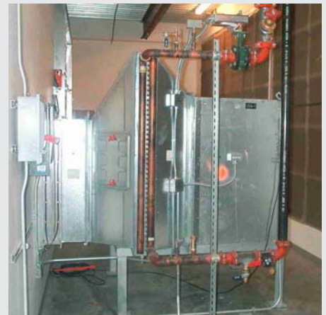
Figure 7.2-D Close-Up of Main Air Filters
