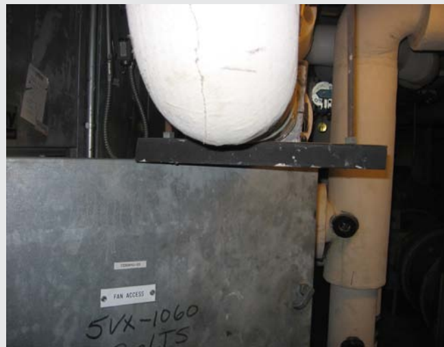
Figure 4.3-J Access Door Blockage
