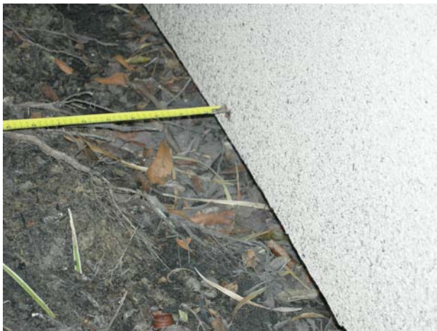
Figure 2.1-H Grade Example 1 Photograph copyright Liberty Building Forensics Group®.
