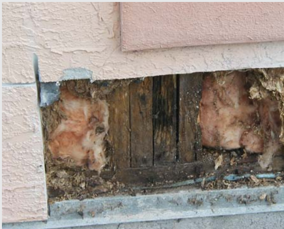
Figure 2.1-D Damage from Window Surround and Window Flashing Failures
