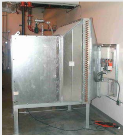
Figure 7.2-C Close-Up of Minimum Outdoor Air Intake Fan
