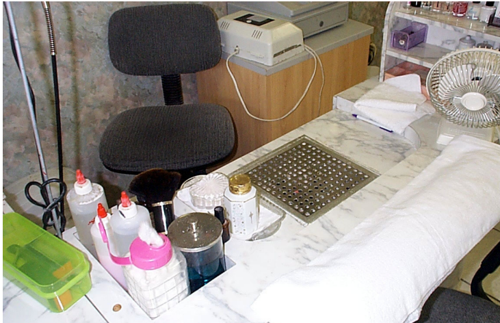
Figure 6.2-B Exhaust Vent Embedded in Nail Care Workstation Source: EPA (2007).
