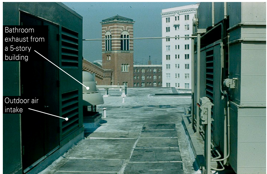
Figure 3.2-B HVAC Outdoor Air Intake Located Downwind of and in Close Proximity to Main Bathroom Exhaust of a Five-Story Office Building Photograph courtesy of Hal Levin.
