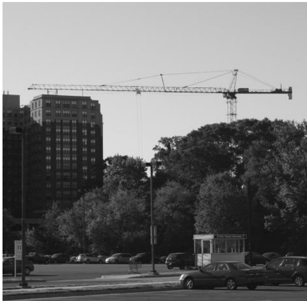
Figure D.1 A tower crane at a construction site at the University of Maryland, College park, 2010 (photo taken by Bilal Ayyub).
