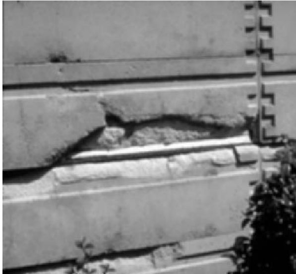
Fig. 7.2 The original precast ‘textile’ concrete blocks were made with fine aggregate, Portland cement and coquina shell. The blocks are highly porous and permeable owing to the absence of coarse aggregate and poor curing. They are therefore susceptible to a high moisture content and subsequent deterioration over successive cycles of wetting and drying. Poor cover to the reinforcement (due to inaccurate steel positioning and insufficient grout and mortar covering) has led to spalling of the blocks (courtesy Ove Arup Partnership).
