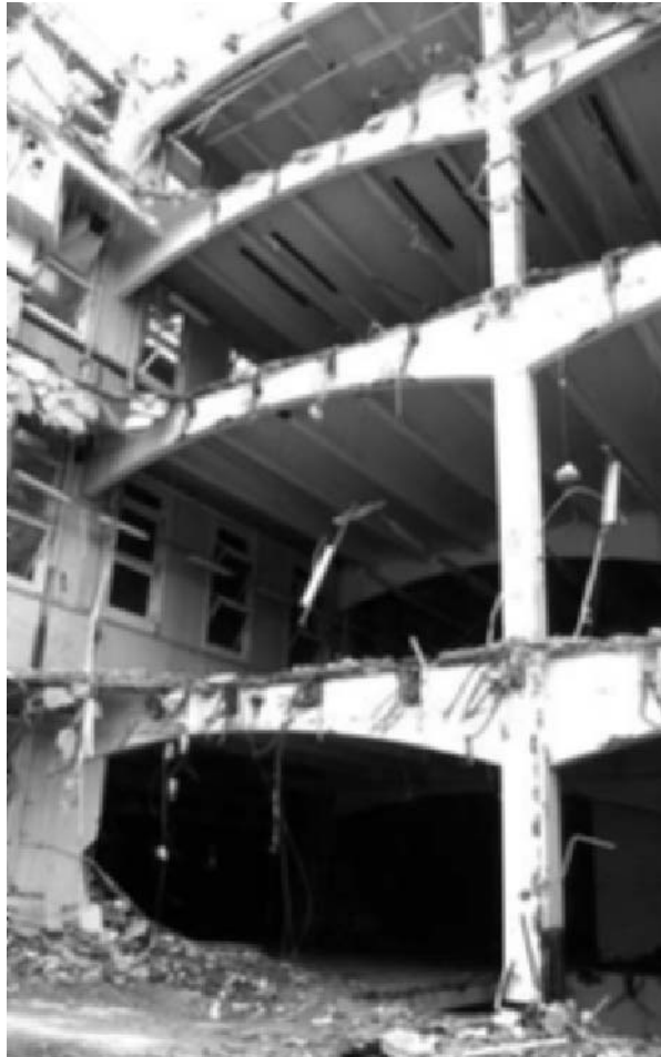
Fig. 2.6 King Edward Street Sorting Office in the City of London, during demolition (photo Michael Bussell).
