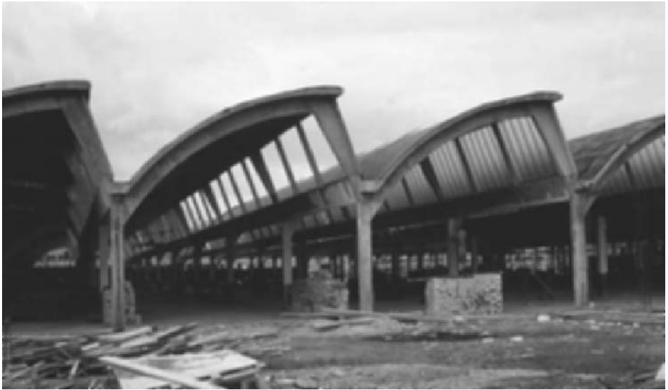
Fig. 2.27 A north-light, concrete-shell factory roof at Cadbury's factory, Moreton, Cheshire, under construction (courtesy Institution of Civil Engineers).
