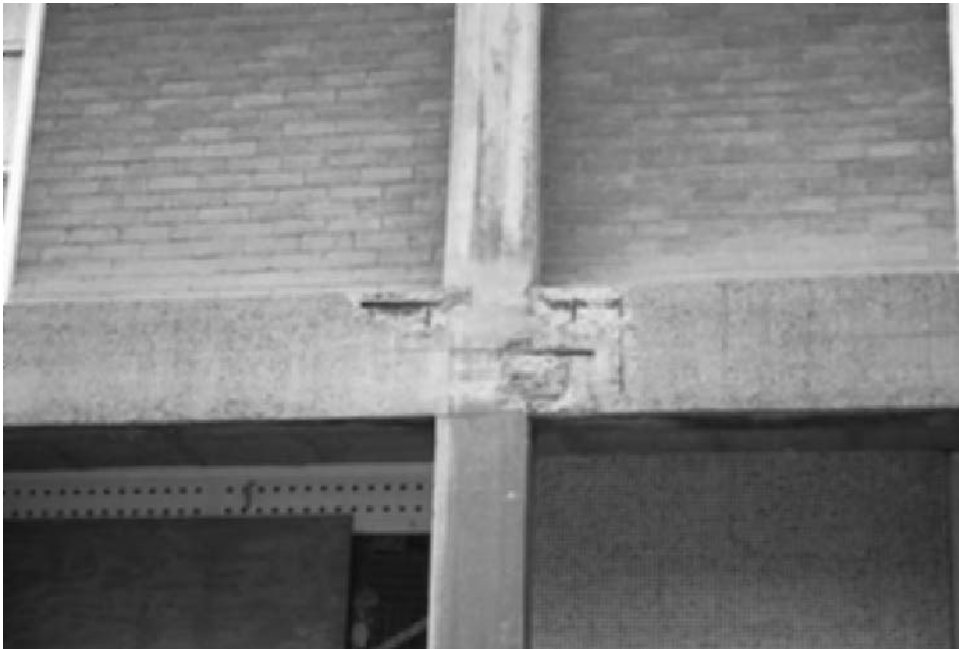
Fig. 4.4 Insufficient cover to reinforcement at Parkhill flats, Sheffield, is one of the most common causes of premature corrosion-induced concrete decay (photo Susan Macdonald).
