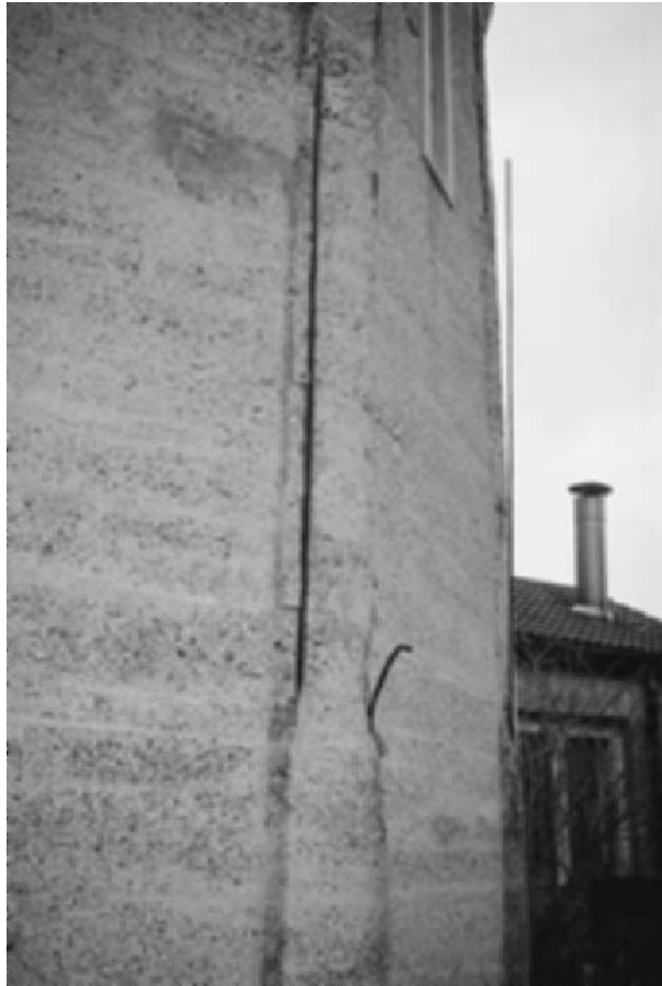
Fig. 1.2 St John and St Mary Magdalene, Goldthorpe, South Yorkshire. Despite the reasonably thick walls, the location of the reinforcement is variable and does not appear to have been well restrained horizontally, as can be seen in the photograph. The concrete is quite porous, and the building is suffering from prolonged deterioration with scant maintenance, which has resulted in some structural problems. Understanding the level of knowledge and types of materials used at the time when it was built is important to an analysis of the problems and may influence the repair decisions.
