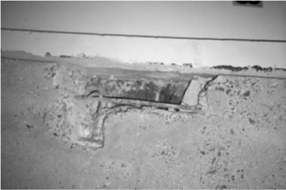
Fig. 5.5 Patch repairs in progress at Pullman Court. Note the thinness of the walls, which is characteristic of early modern architects' work in Britain. The concrete has always been painted (Susan Macdonald).
