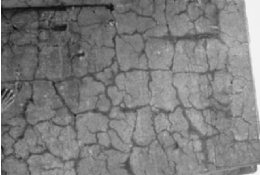
Fig. 4.5 Map cracking due to an alkali–silica reaction.
