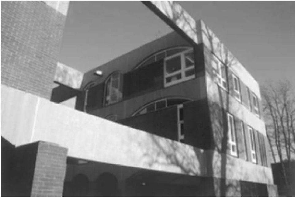
Fig. 8.16 Falmer House after repair. The crack repair through the beam is not particularly successful. The repair could have been improved visually by improved finishing. The other patch repairs to this corner of the building have blended in well with the parent concrete.
