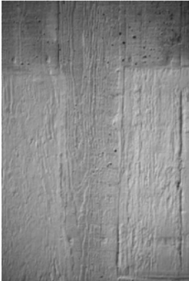
Fig. 5.2 Patch repairs at the Alexandra Road Housing Estate in Camden, London. This is a Grade II* listed building, and therefore it was important to match the repairs as closely as possible to the parent concrete. The high-quality, board-marked concrete finish was an important feature of the architect's design. A latex mould was used to replicate the timber-board-marked finish (photo Susan Macdonald).
