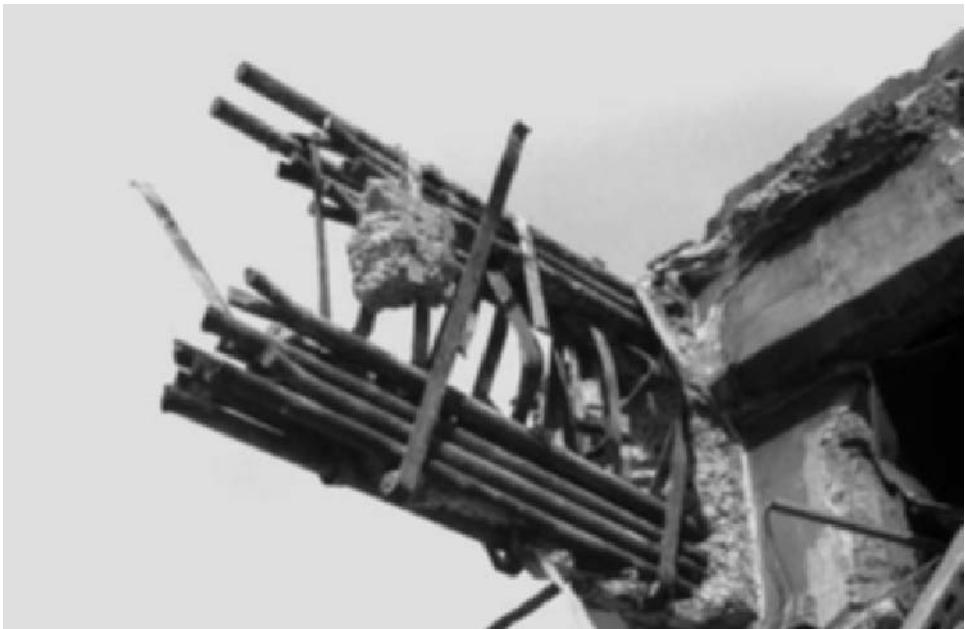
Fig. 2.11 King Edward Street Sorting Office. Column head with congested Hennebique main steel, exposed during demolition (photo Michael Bussell).
