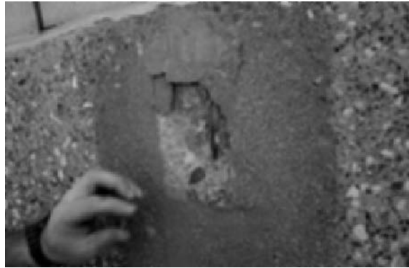
Fig. 8.8 Removal of a delaminated concrete repair: this repair was installed to the level of the reinforcing steel only (photo Paul Gaudette).
