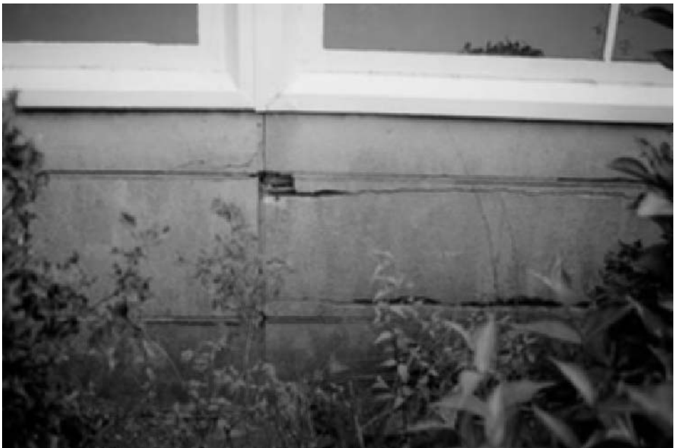
Fig. 8.14 Corrosion of the fixings at the corners and typical corrosion along the top and bottom of the precast panels. Note the junction with the window sill. Increasing the thickness of the panels creates a difficulty at the junction of the panels and the cover of the windows and door frames (photo Susan Macdonald).
