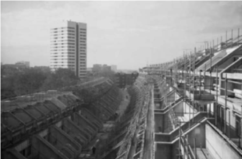
Fig. 5.8 The concrete repairs at the Alexandra Road Housing Estate in Camden were carried out in a manner that attempted to retain the original concrete finish and appearance. Previous repairs had resulted in numerous patches all over the building that were not a good match with the parent concrete (photo Susan Macdonald).
