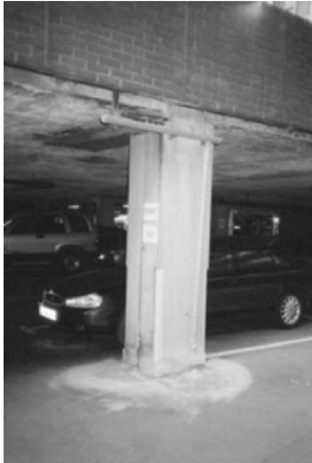
Fig. 4.6(a) Poor maintenance of this car park has led to the formation of a stagmite where the inadequate drainage keeps water off cars but does not cure or control leakage from the floor above.
