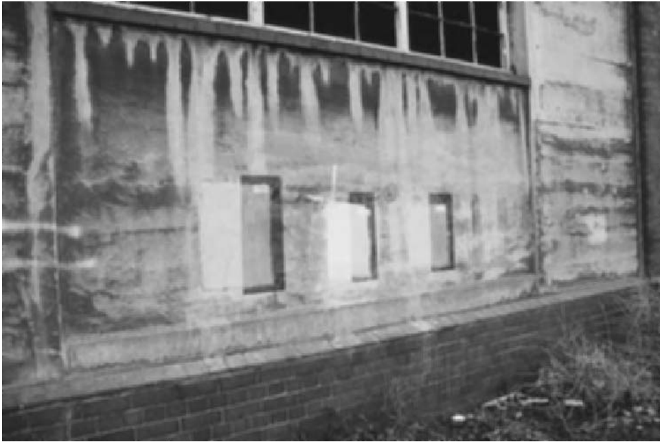
Fig. 6.2 Great Western Goods Shed, Bristol (1910). Note the soiling under the window ledges from environmental pollution in areas that are not regularly washed with water. Trials were an important part of the project during the writing of the specification. The figure shows trial external finishes (photo Susan Macdonald).
