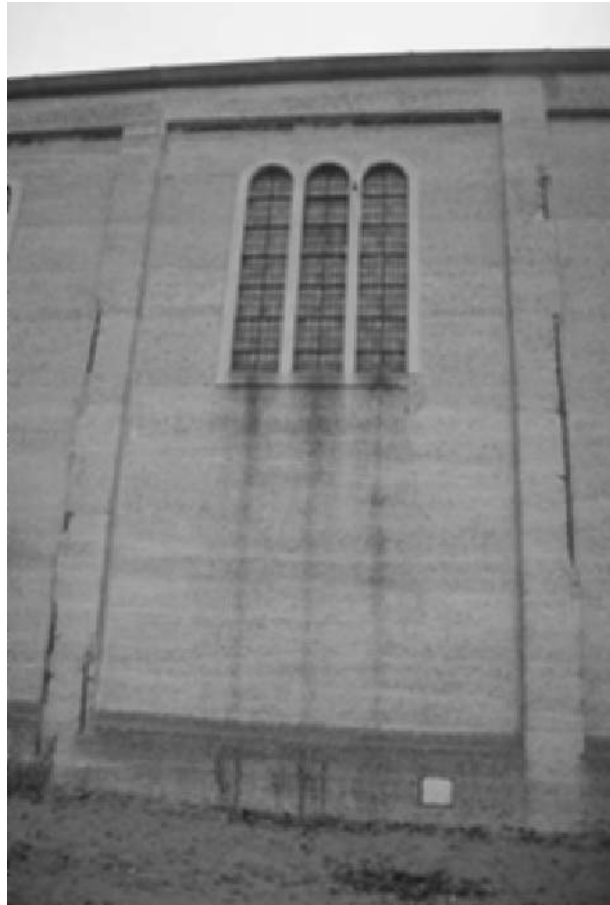
Fig. 6.3 St John and St Mary Magdalene, Goldthorpe, South Yorkshire, 1914–1916. Rust staining of the concrete below the windows due to the corrosion of the metal window guards (photo Susan Macdonald).
