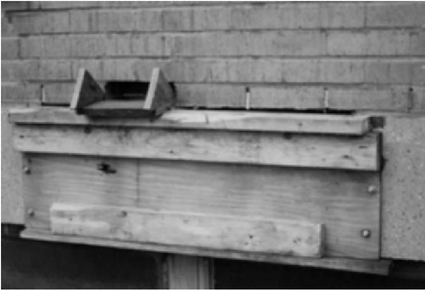
Fig. 8.11 Installation of formwork and a port for ease of concrete placement (photo Paul Gaudette).
