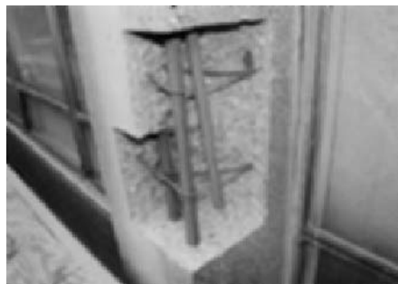
Fig. 8.10 Completion of the preparation works in the repair area prior to the installation of the formwork (photo Paul Gaudette).
