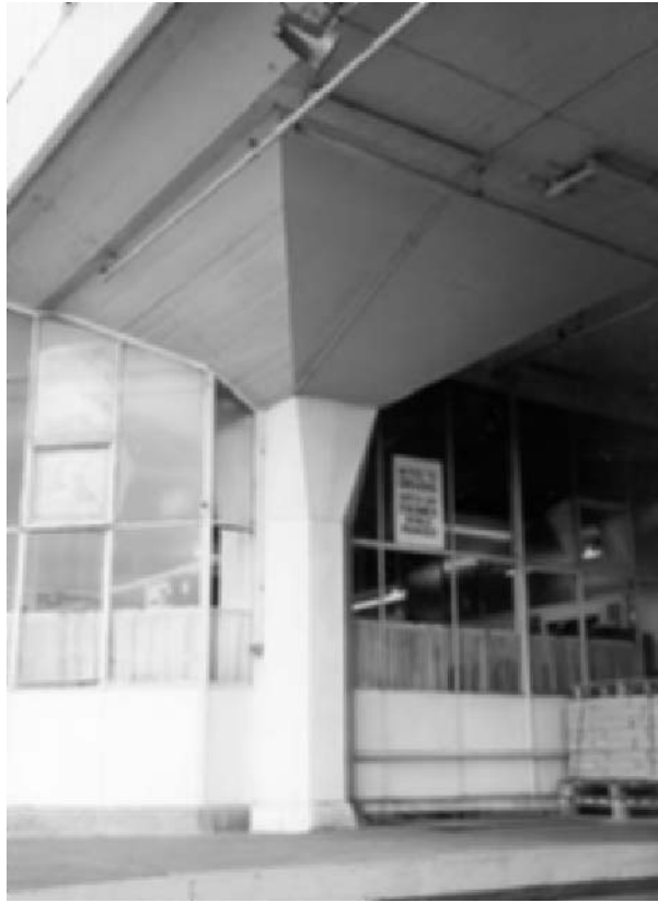
Fig. 2.17 Column detail in Boots 'drys' factory, Beeston, Nottingham, 1935–1936. Engineer and architect Owen Williams (photo Bill Addis).
