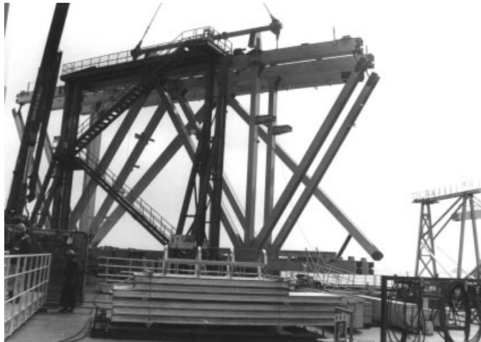
Figure 7.51 Prefabricated truss elements for the sway bracings and the vertical main trusses of the Akashi Kaikyo Bridge after being lifted onto the bridge deck at the pylons
