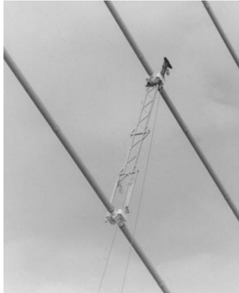
Figure 8.49 Clamps with dampers at the connection between the main stays and the cross-lattice members on the Normandy Bridge
