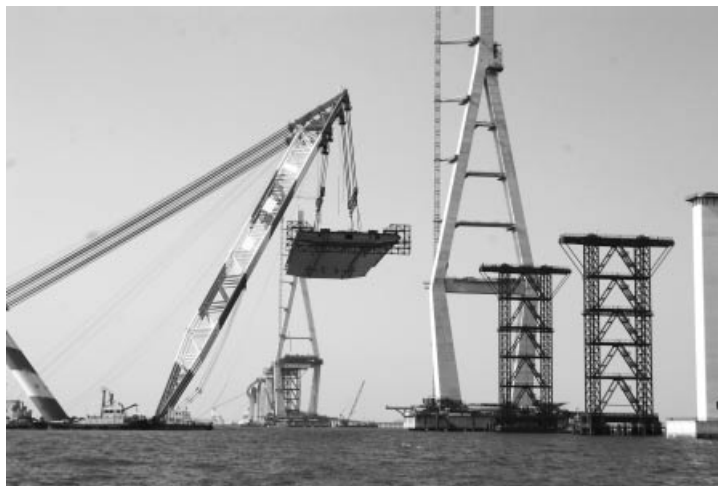
Figure 7.77 Erection of a truss element by two floating cranes during construction of the Incheon Bridge (courtesy of H. Tanaka, Samsung C&T)
