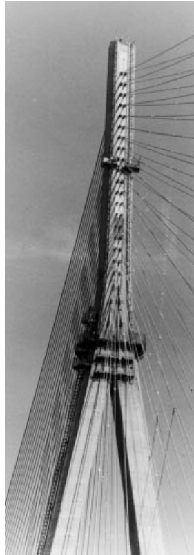
Figure 6.63 Anchor box at the top of the pylon in the Normandy Bridge
