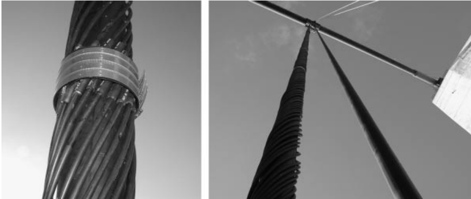
Figure 9.21 The EIDI system installed on selective hangers of the Storebælt Bridge (Photo credit: E. Laursen)
