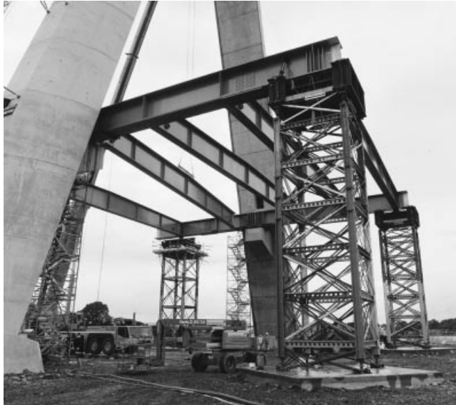
Figure 7.70 Initial erection of the deck on temporary supports at the pylon location (Photo credit: Arup)
