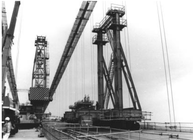
Figure 7.52 Multi-wheel trailer for transport of prefabricated truss elements along the deck of the Akashi Kaikyo Bridge
