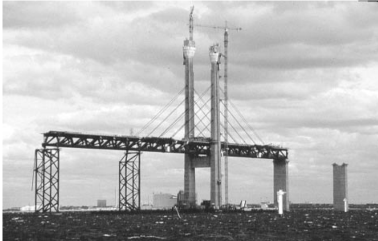
Figure 7.65 Erection of the stiffening truss of the Øresund Bridge by application of temporary piers in the main span
