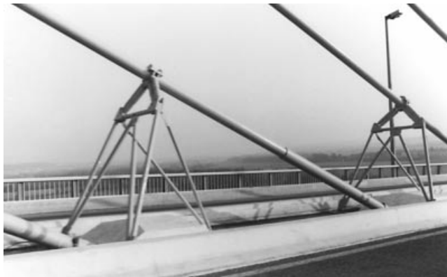
Figure 8.47 Shock absorbers erected to reduce local oscillations of the stay cables of the Brotonne Bridge
