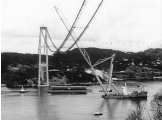
Figure 7.62 Erection of deck segments in the Askøy Bridge by a floating crane
