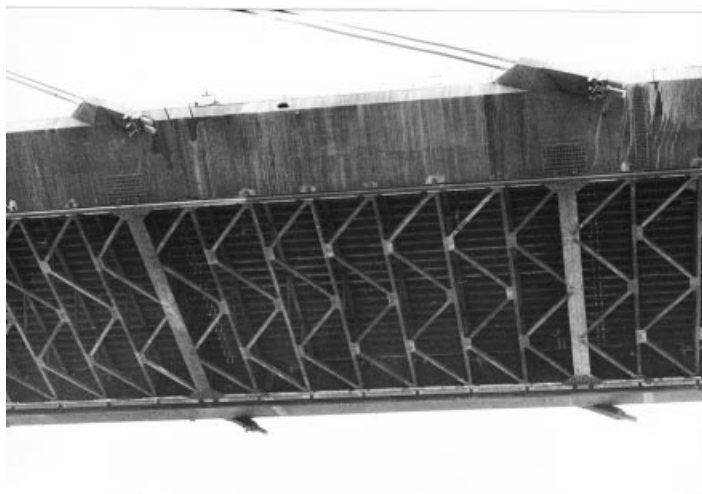
Figure 4.63 Lower lateral bracing in the Zarate-Brazo Largo Bridge to increase torsional stiffness of the deck
