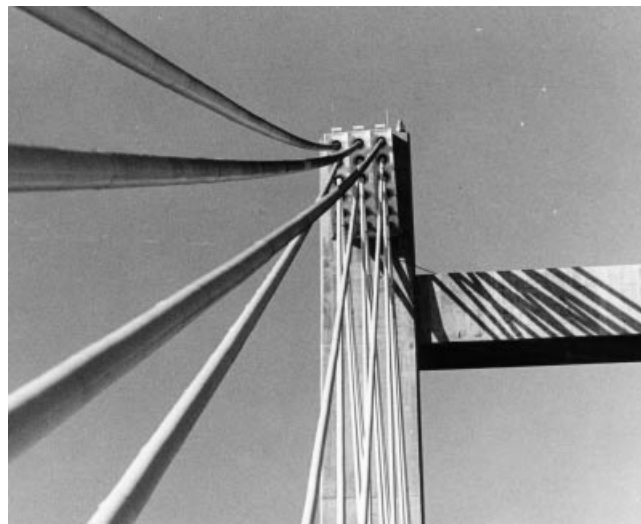
Figure 6.59 Pylon head with a lateral displacement of stay cables to allow the anchorages to be positioned side by side at the pylon head (Pasco-Kennewick Bridge)
