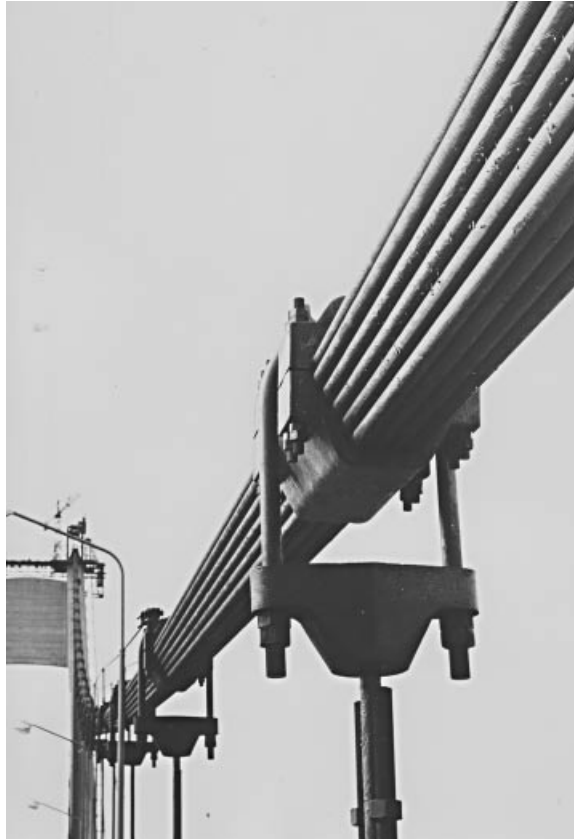
Figure 2.17 Suspension bridge main cable composed of tightly spaced locked-coil strands (original Tancarville Bridge)
