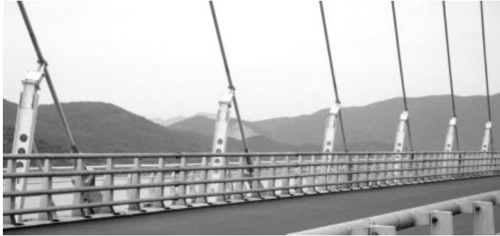
Figure 6.25 Stay cable damper positioned high above the roadway
