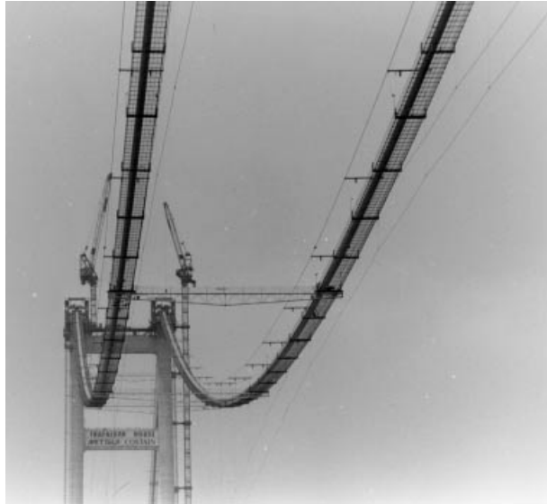
Figure 7.13 Suspension bridge with catwalks as installed during cable erection (Tsing Ma Bridge)
