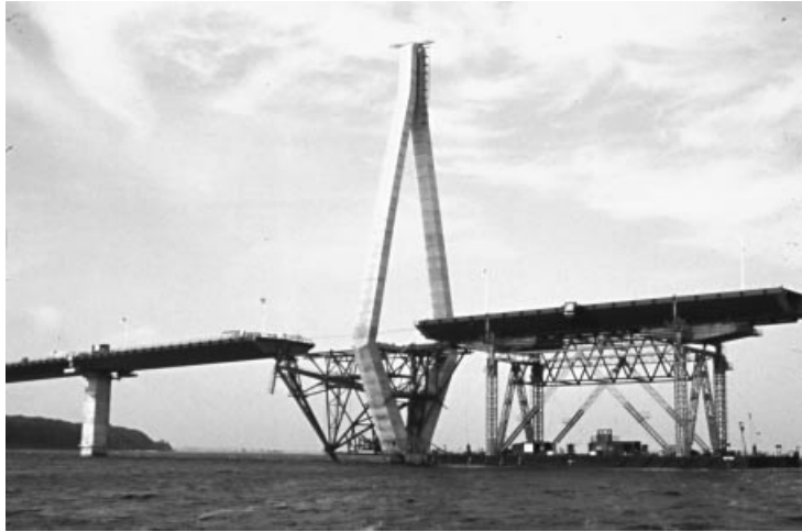
Figure 7.76 80 m long box girder element about to be pulled through the pylon during erection of the Farø Bridge
