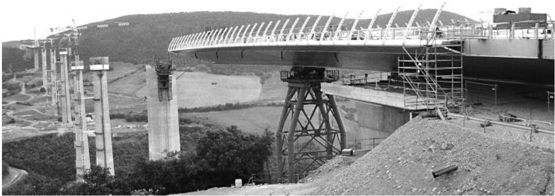
Figure 7.87 The deck of the Millau Viaduct during the initial launching via a temporary support onto the first permanent pier
