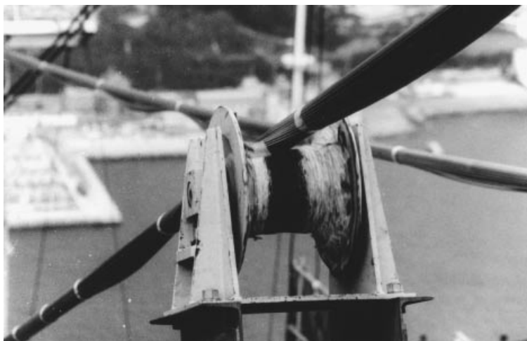
Figure 2.23 PPWS supported on a roller at the catwalk when pulled across from anchor block to anchor block (Akashi Kaikyo Bridge)
