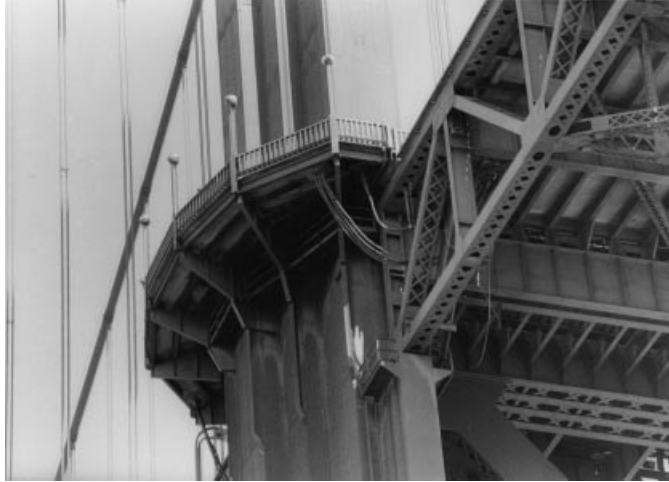
Figure 5.46 Cantilevered deck attached to the pylon for passing of pedestrian lane outside the pylon leg (Golden Gate Bridge)
