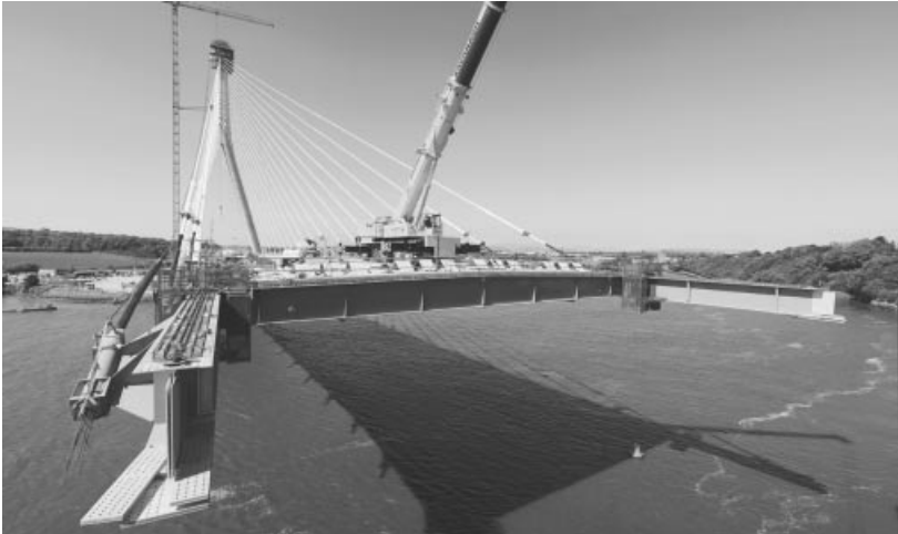
Figure 7.71 Free cantilever of a ladder deck in a cable stayed bridge (Photo credit: Arup)
