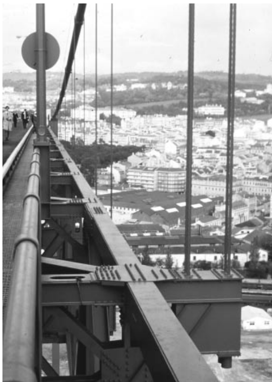
Figure 6.46 Hanger ropes of the 20th April Bridge spaced to avoid hanger clamps below the cable clamps
