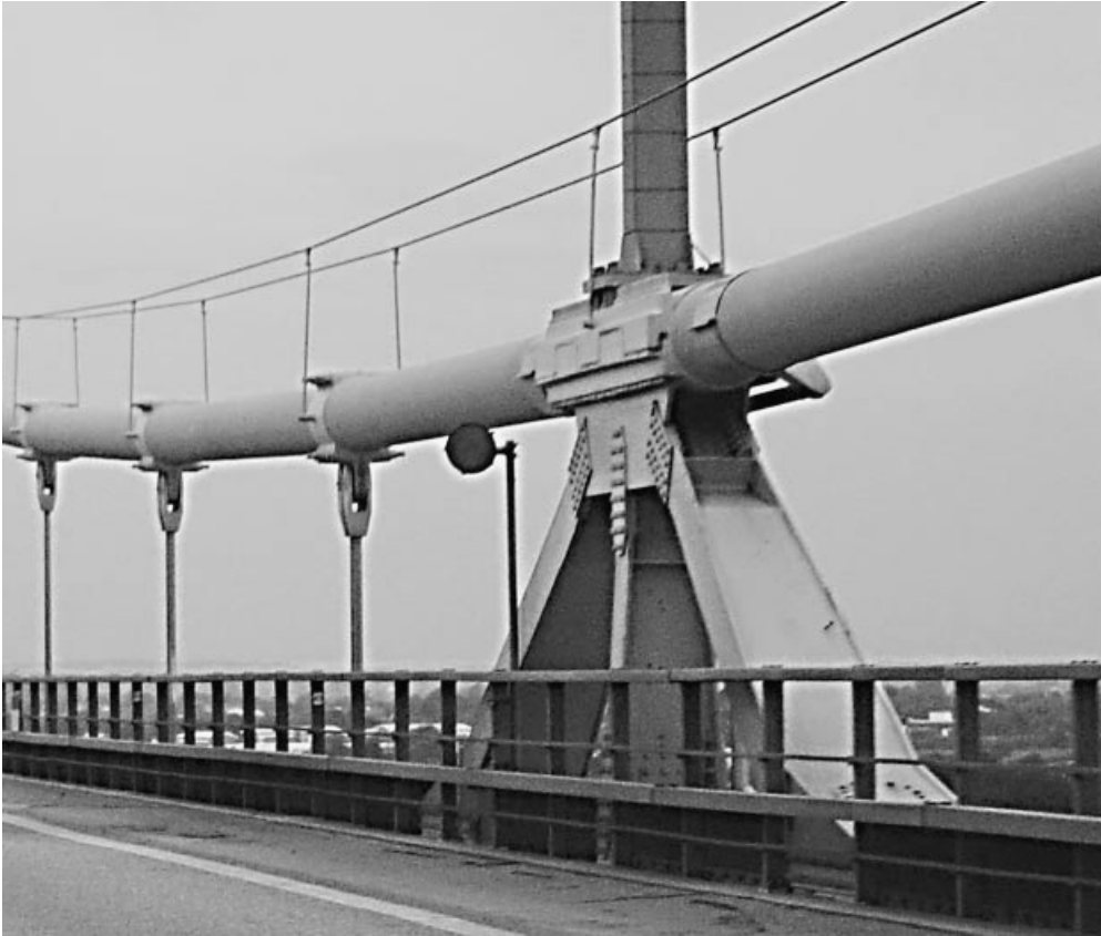
Figure 3.202 Bracing system between the central clamp and the deck of the Lillebælt Bridge
