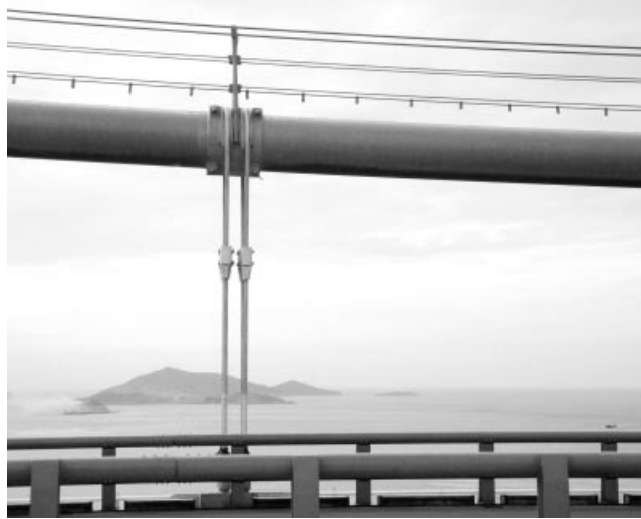
Figure 6.49 Grooved main cable clamp with helical hanger ropes in the Xihoumen Bridge from 2009
