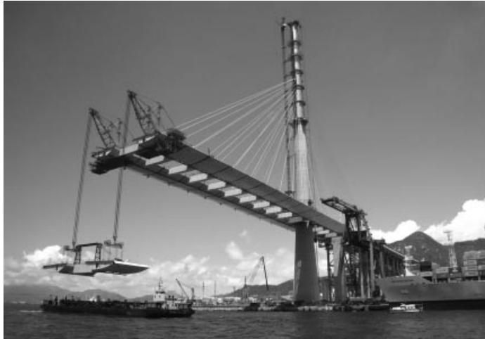
Figure 7.80 Purpose-built crane for lift of deck segments in the Stonecutters Bridge (courtesy of Steve Kite, Arup)
