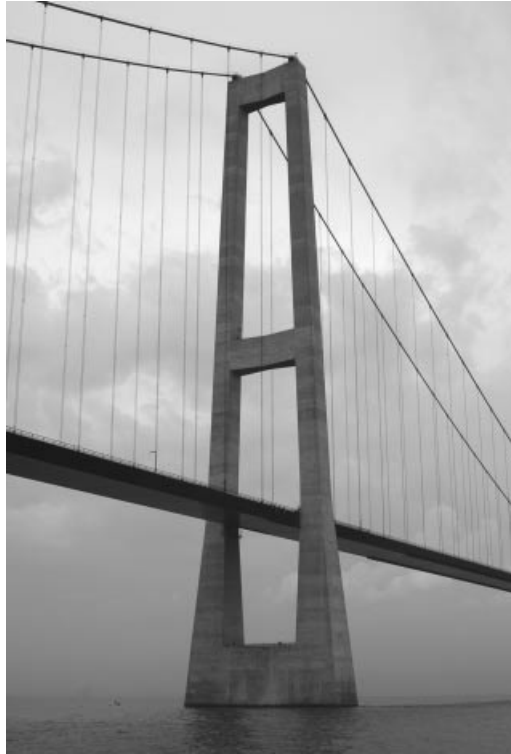
Figure 4.17 Pylon of the Storebælt East Bridge without a cross beam below the deck
