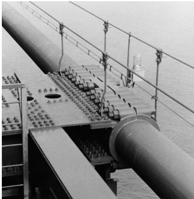
Figure 3.54 Central clamp connecting the main cable to the top chord of the stiffening truss in the 20th April Bridge
