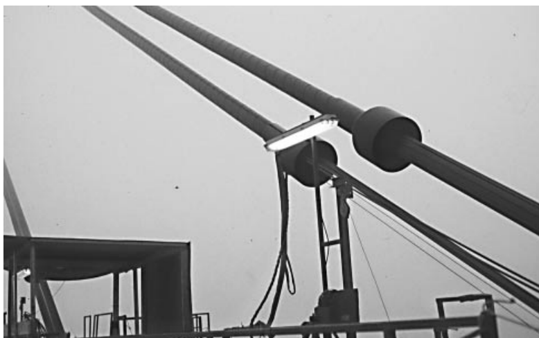
Figure 7.41 The permanent PE-tube erected to support seven-wire strands during erection (Øresund Bridge)
