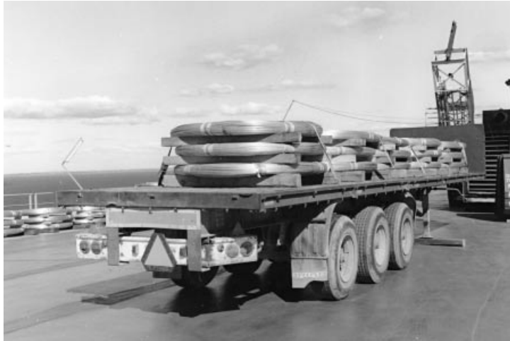
Figure 7.19 Wire coils transported by truck to the site of the Storebælt East Bridge
