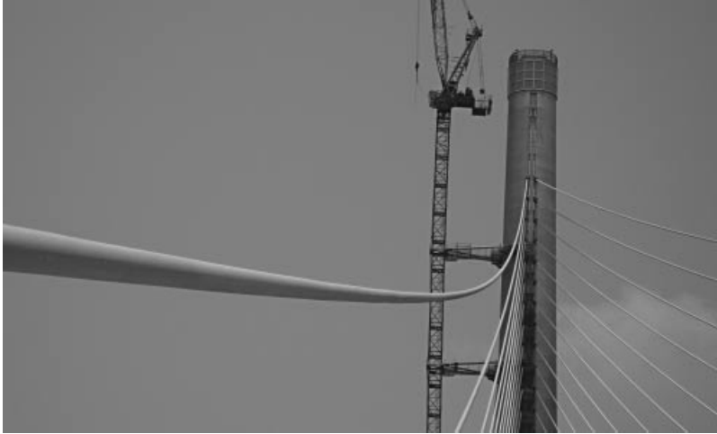
Figure 2.61 Visible sag of a stay cable in the Stonecutters Bridge
