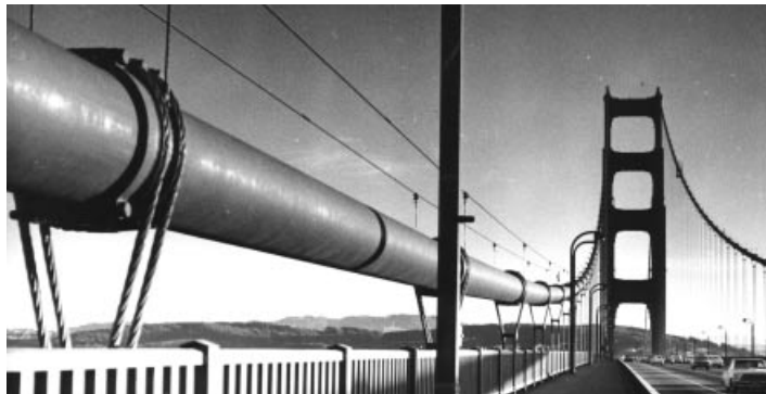
Figure 6.45 Hanger clamps below the main cable clamp to reduce hanger rope spacing (Golden Gate Bridge)
