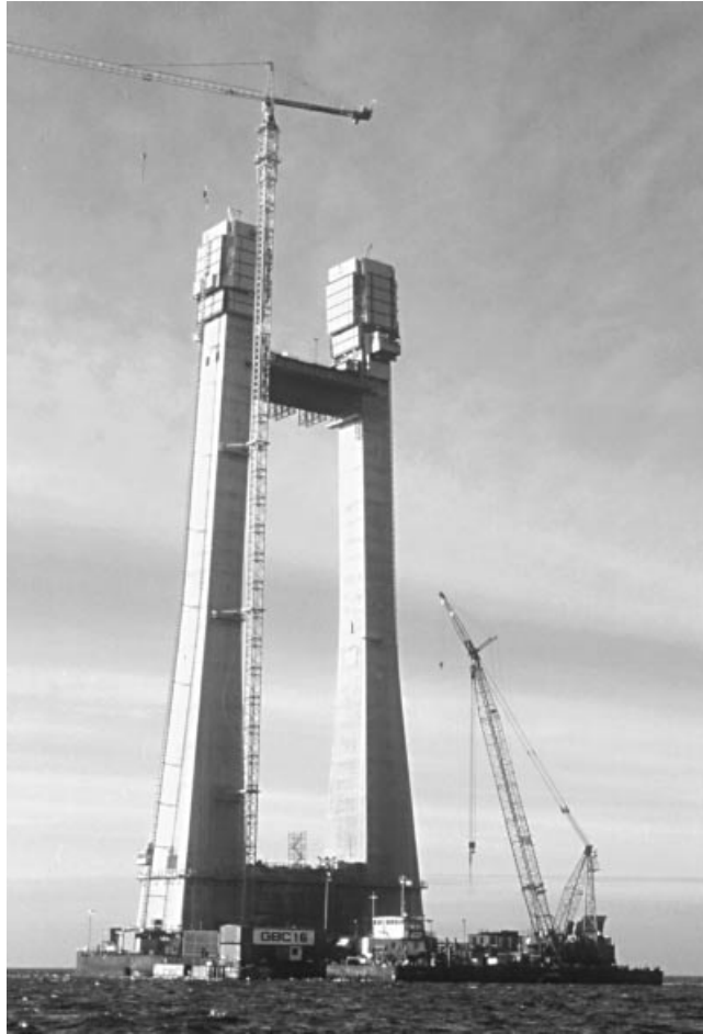
Figure 7.8 The East Bridge pylon after installation of the scaffolding beam for the lower cross beam
