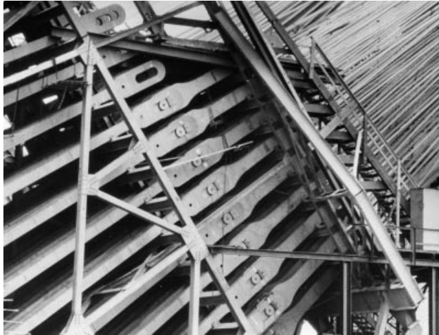
Figure 6.78 Eye-bar chains with elongated holes to allow adjustments by shimming (Verrazano Narrows Bridge)
