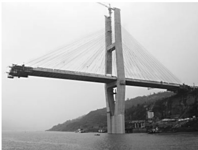
Figure 7.82 Form traveller at the tip of an in situ cast ladder deck in concrete
