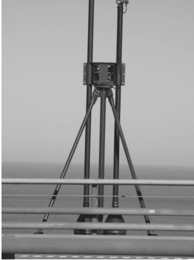
Figure 8.43 Storebælt Bridge point viscous dampers
