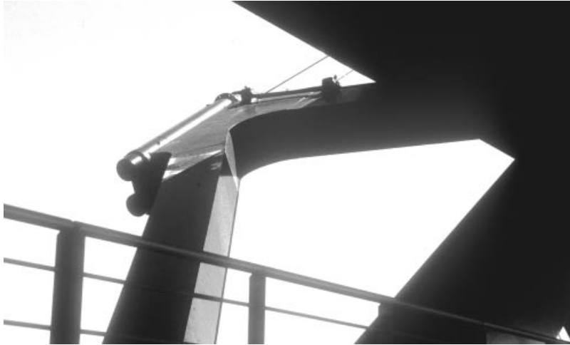
Figure 6.37 Stay cable anchored to a triangular outrigger outside the main trusses in the Øresund Bridge
