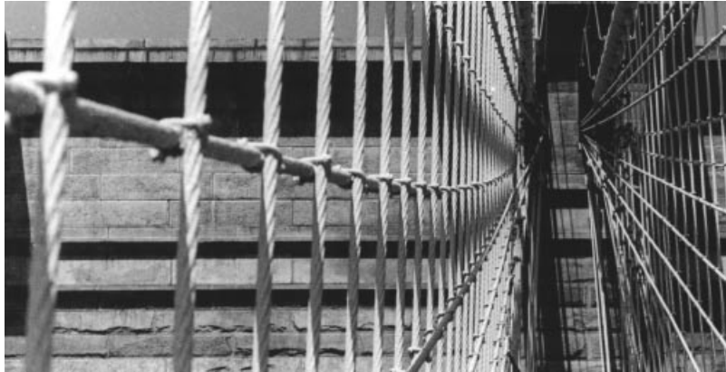
Figure 3.131 Sagging stays of the Brooklyn Bridge, as seen from the bridge deck
