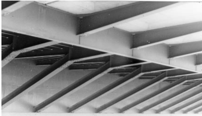
Figure 4.50 Deck of the Friedrich Ebert Bridge with all floor beams supported by inclined struts
