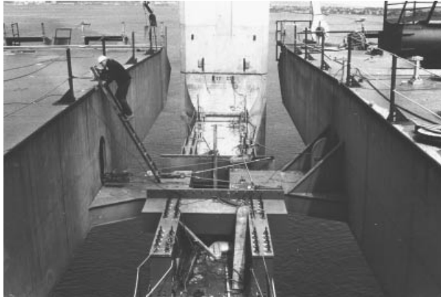
Figure 4.11 Wind bearings between the deck and the pylon cross beam (Lillebælt Bridge)
