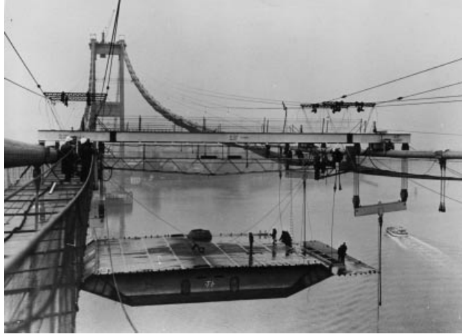
Figure 7.59 Erection unit of the Severn Bridge box girder lifted by a single lifting strut
