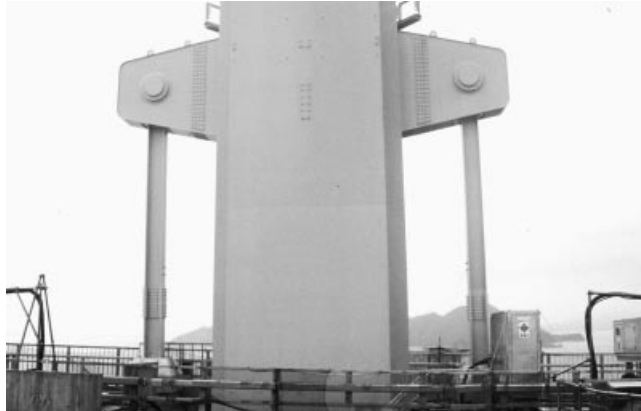
Figure 4.9 End links to transfer vertical forces from the deck to the pylon (Kurushima Bridge)
