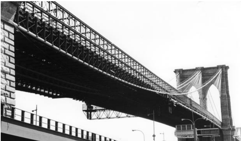
Figure 3.40 Brooklyn Bridge with the main cable below the stiffening truss adjacent to the anchor blocks
