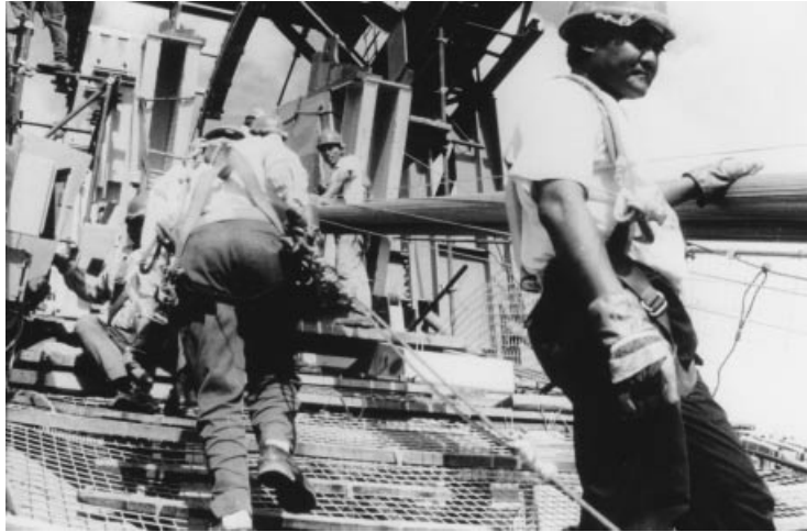
Figure 7.25 Sag adjustment of individual wires during spinning operations at the Tsing Ma Bridge
