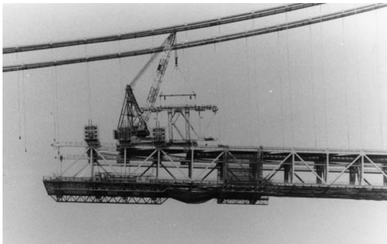
Figure 7.53 Derrick crane at the tip of the stiffening truss of the Akashi Kaikyo Bridge. The crane is about to pick up a sway bracing element and move it into position between the previously erected main truss extensions
