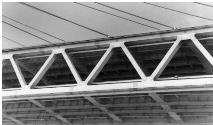
Figure 4.94 The stiffening truss of the Higashi Kobe Bridge as seen from below
