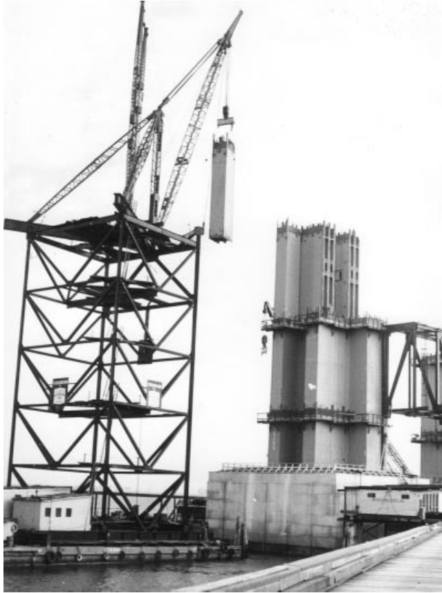
Figure 7.1 Erection of the lower part of the Verrazano Narrows Bridge pylon by a floating derrick crane
