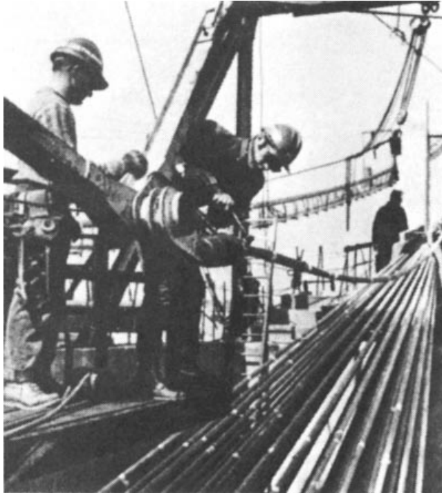
Figure 1.44 Hauling of a prefabricated parallel-wire strand during construction of the Clairborne Pell Bridge (Newport Bridge)
