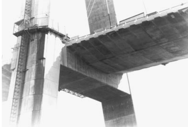
Figure 4.25 Monolithic joint between the deck and the pylon in the Normandy Bridge
