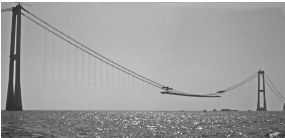
Figure 4.120 Deck erection of the Storebælt East Bridge from midspan towards the pylons
