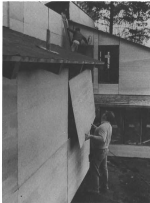
Fig. 8.68. Plywood sheathing is nailed to studs of a load-bearing wall. (Courtesy Western Woods Products Association)
