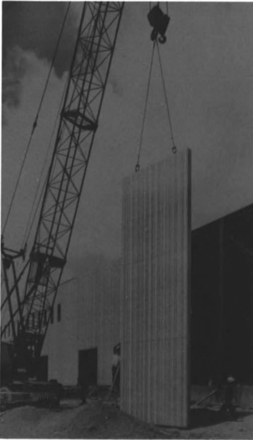
Fig. 15.9. Striated, precast-concrete panel being erected for a curtain wall. (Courtesy High Concrete Structures, Inc., of New Jersey)
