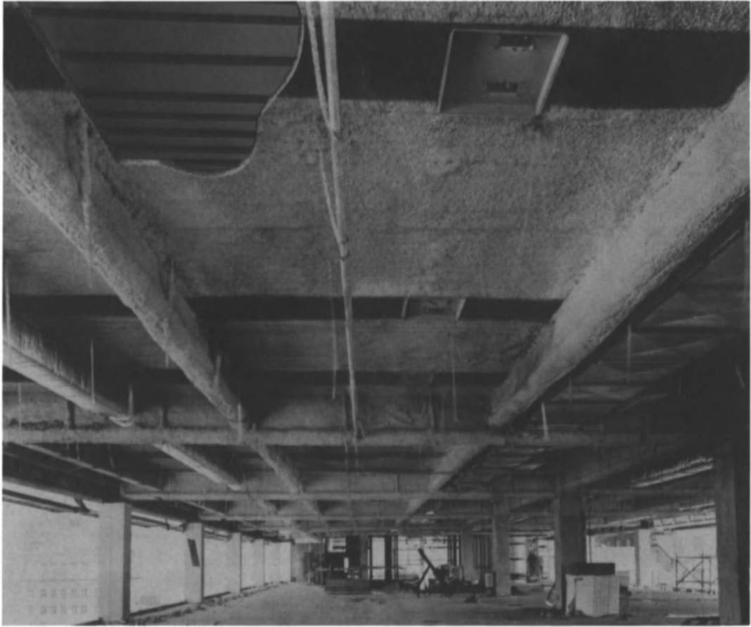
Fig. 8.63. Cold-formed steel deck supported on steel beams, with sprayed-on fireproofing. (Courtesy H. H. Robertson Co.)
