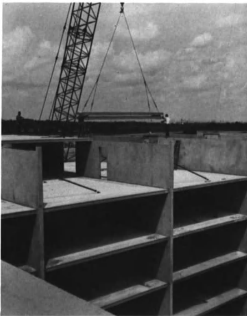
Fig. 2.12. Load-bearing concrete wall supports concrete floors in a multistory building. Floors and walls were prefabricated away from the building site. (Courtesy Formigli Corp.)
