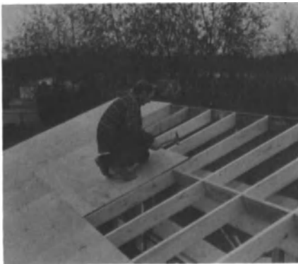
Fig. 8.62. Plywood deck is nailed to rafters spaced 24-in. center-to-center for a roof. (Courtesy American Plywood Association)
