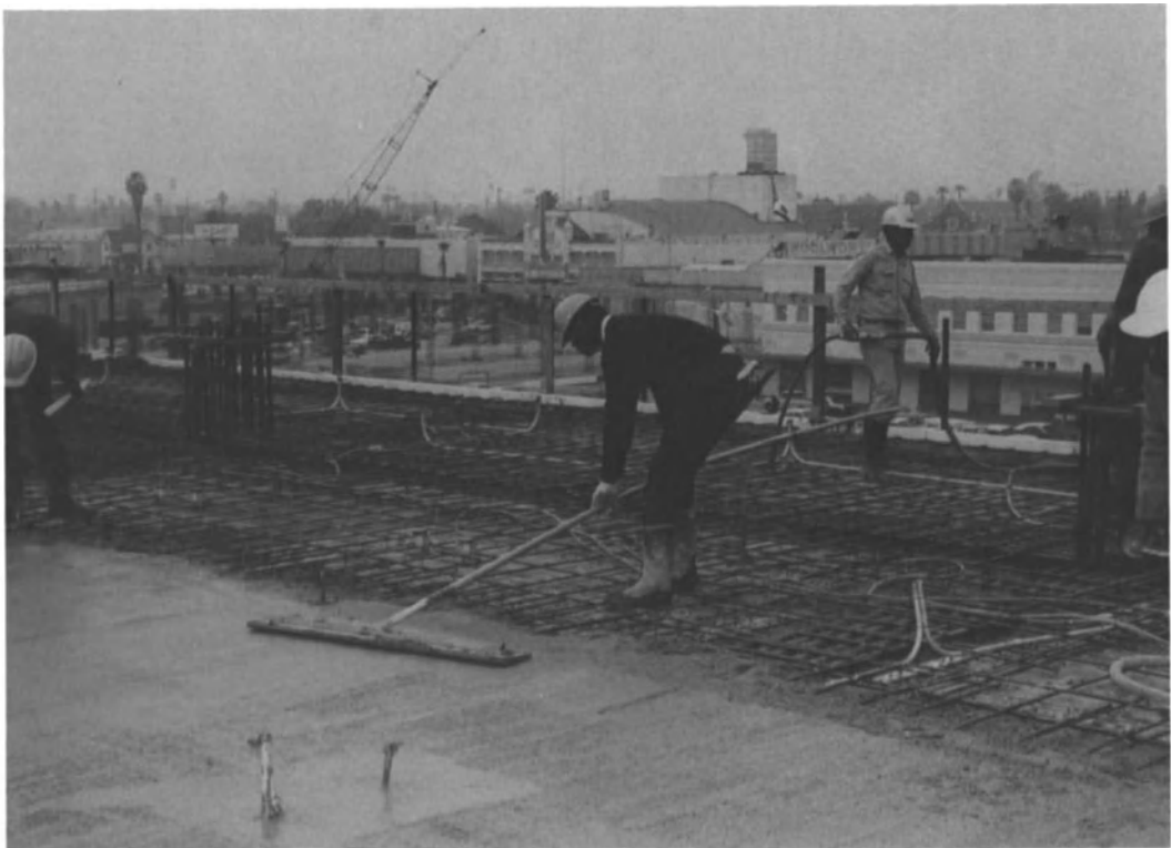
Fig. 8.61. Rebars and electrical conduit set on formwork, ready to receive concrete for a flat slab. (Courtesy Symons Manufacturing Co.)
