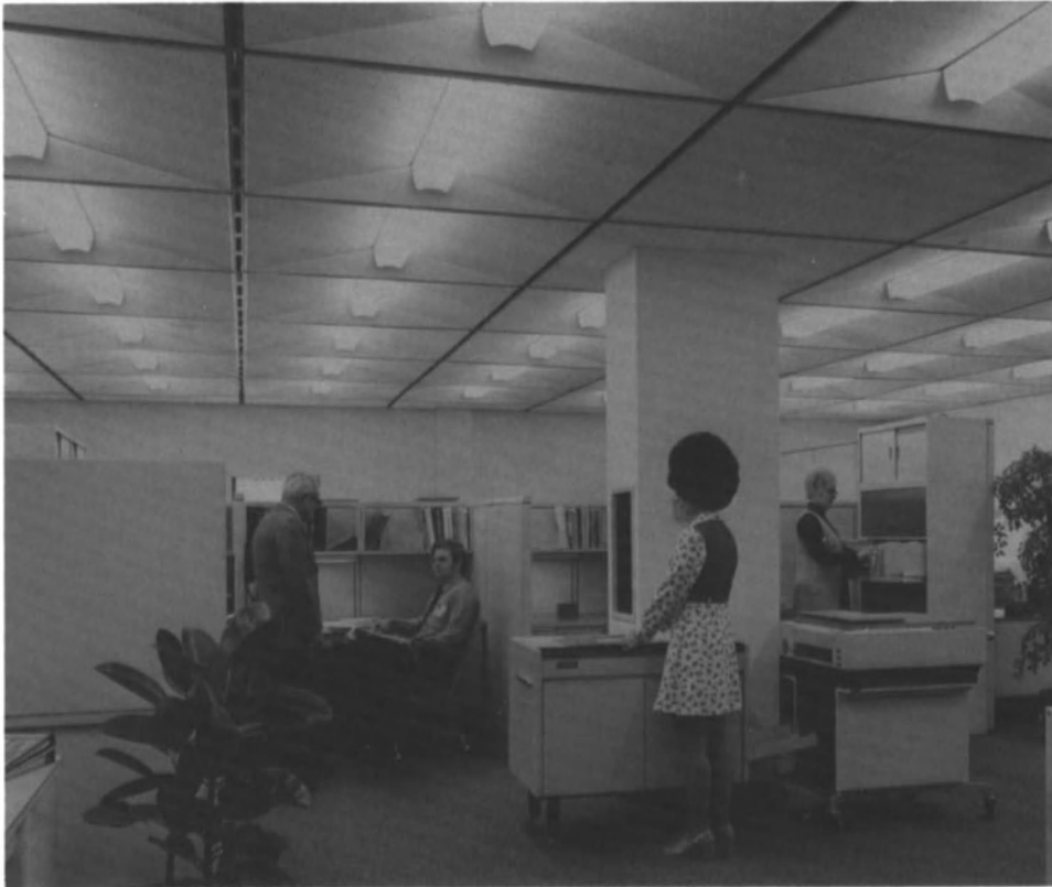
Fig. 11.5. Modular ceiling panels equipped with fluorescent luminaires and integrated with linear air-conditioning diffusers.
