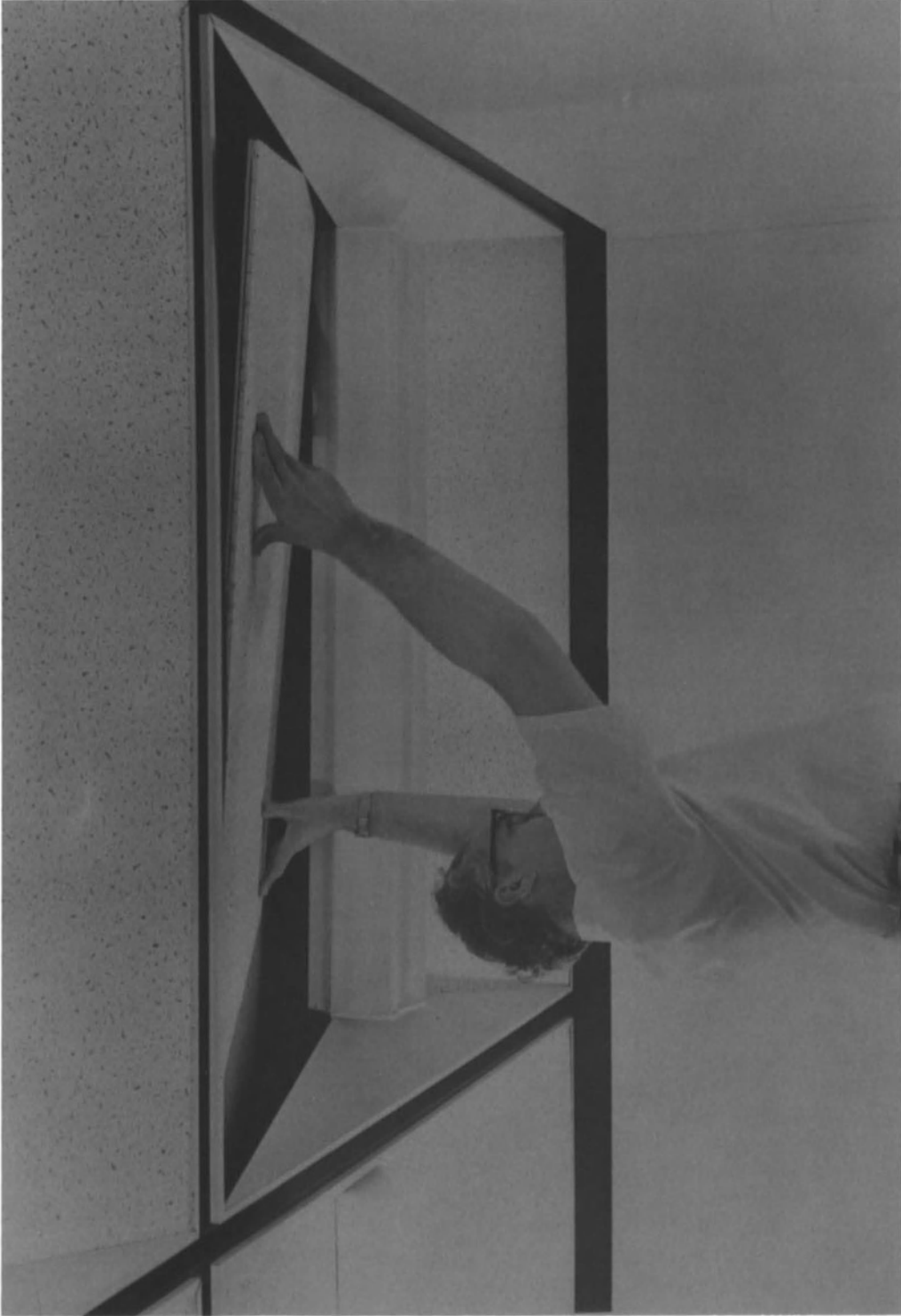
Fig. 12.1. Installation of a fissured acoustical tile in a coffered ceiling.
