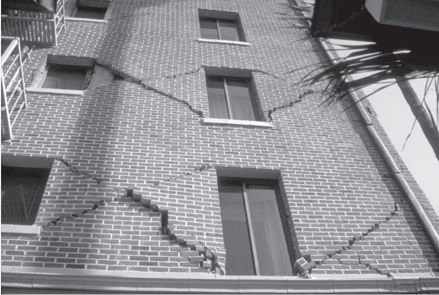
FIGURE 2.6 Structural damage to masonry building resulting from the 1994 Northridge, California, earthquake. Reproduced courtesy of the National Information Service for Earthquake Engineering, University of California, Berkeley.
