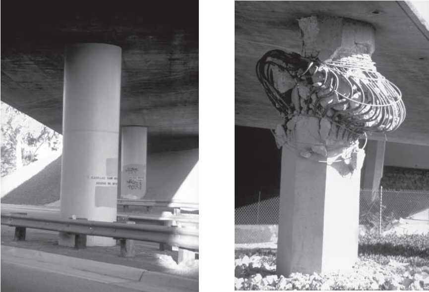
FIGURE 1.2 Comparison of retrofitted and unimproved concrete bridge columns following the 1994 Northridge, California, earthquake. Left: Cadillac Avenue ramp at Interstate 10 (Santa Monica Freeway). Right: Highway 118/Bull Creek Bridge. Reproduced courtesy of the National Information Service for Earthquake Engineering, University of California, Berkeley.
