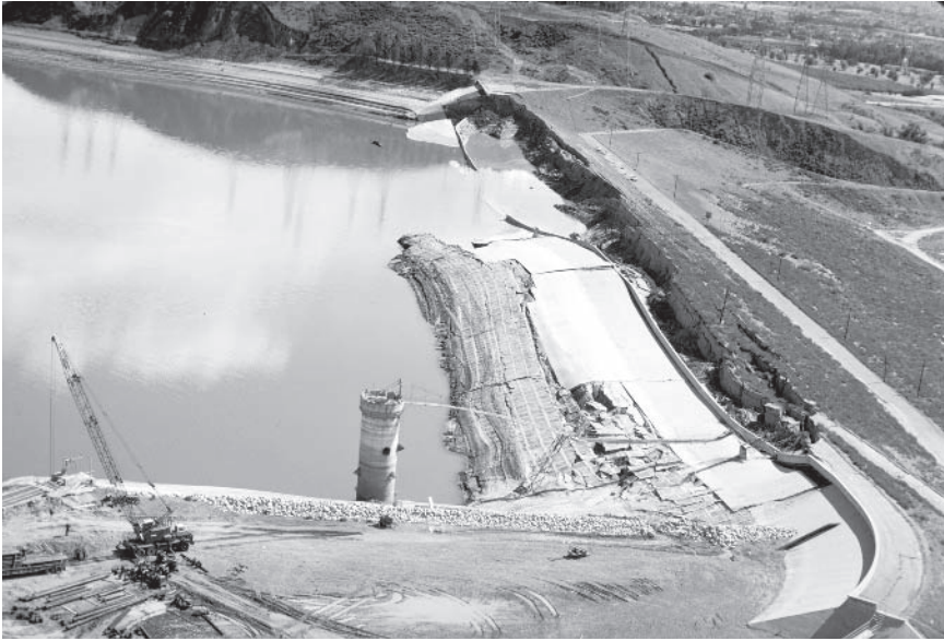
FIGURE 2.4 Embankment failure due to liquefaction at the Lower Van Norman Dam, 1971 San Fernando, California, earthquake. Reproduced courtesy of the National Information Service for Earthquake Engineering, University of California, Berkeley.
