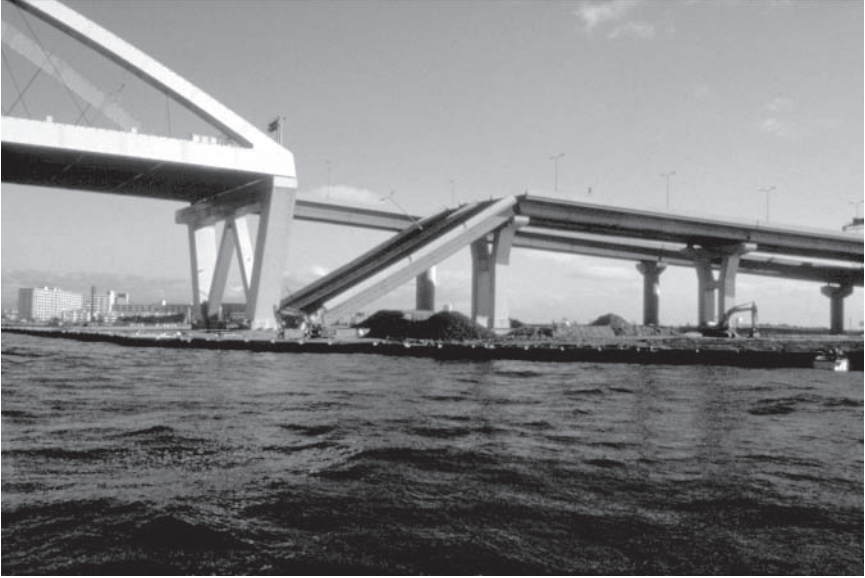
FIGURE 2.8 Failure of a span of the Nishinomiya Bridge during the 1995 Kobe, Japan, earthquake. Reproduced courtesy of the National Information Service for Earthquake Engineering, University of California, Berkeley.
