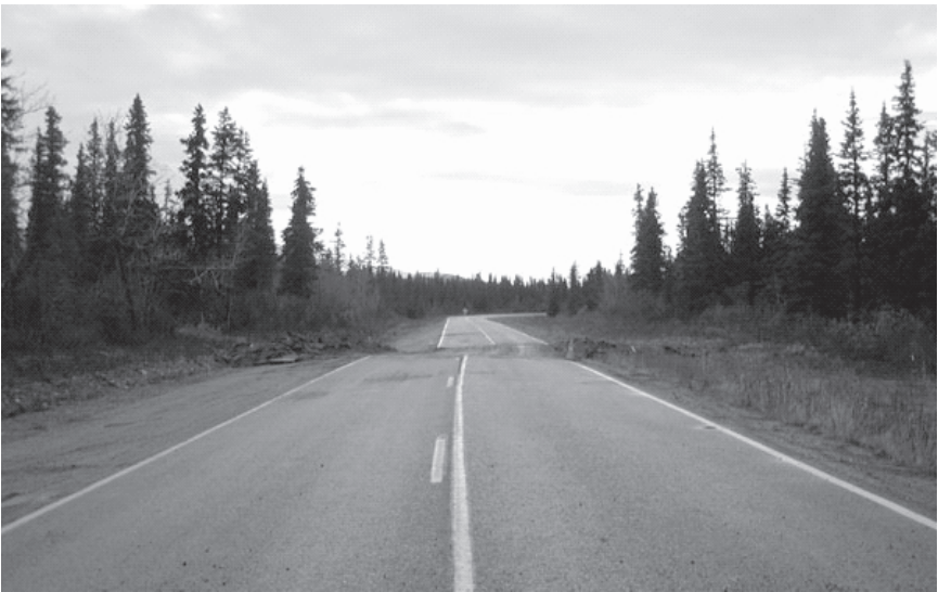
FIGURE 2.9 Lateral highway offset of 2.5 meters as a result of the 2002 Denali, Alaska, Earthquake. SOURCE: Alaska Department of Natural Resources. Photo by Patty Craw, Division of Geological and Geophysical Surveys.
