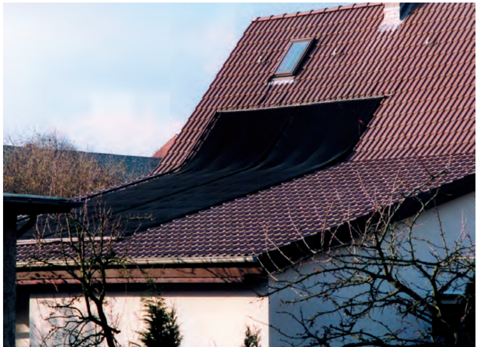
Figure 7.24. Private solar system for pool heating
