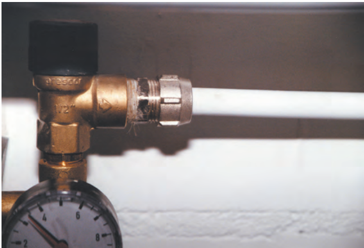
Figure 4.54 Incorrect PE pipe as exhaust line
