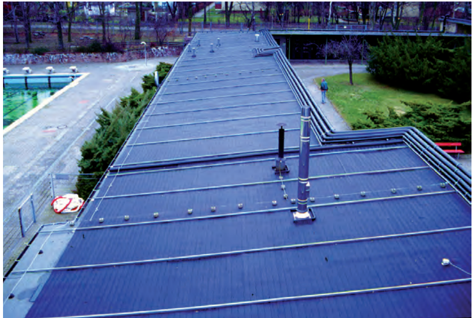
Figure 7.25. Solar system for heating open-air pool water in the Mariendorf summer pool, Berlin. Source: DGS
