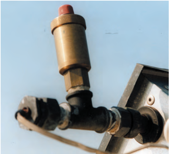
Figure 4.56 Unsuitable automatic air bleed and unclear sensor positioning
