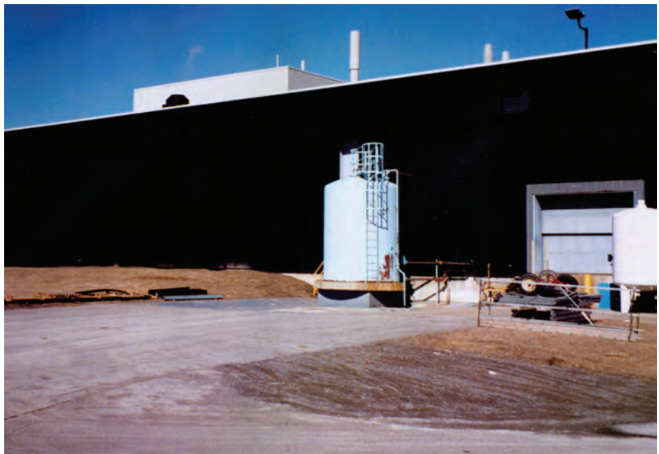
Figure 8.33 Solar wall on General Motors building in Ontario. Source: Conserval
