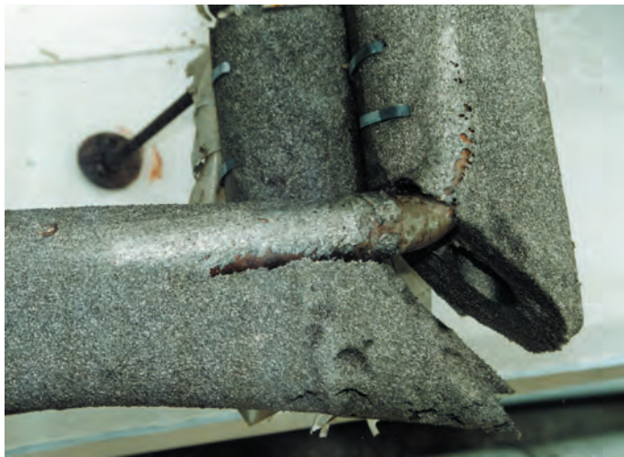
Figure 4.53 Damaged thermal insulation
