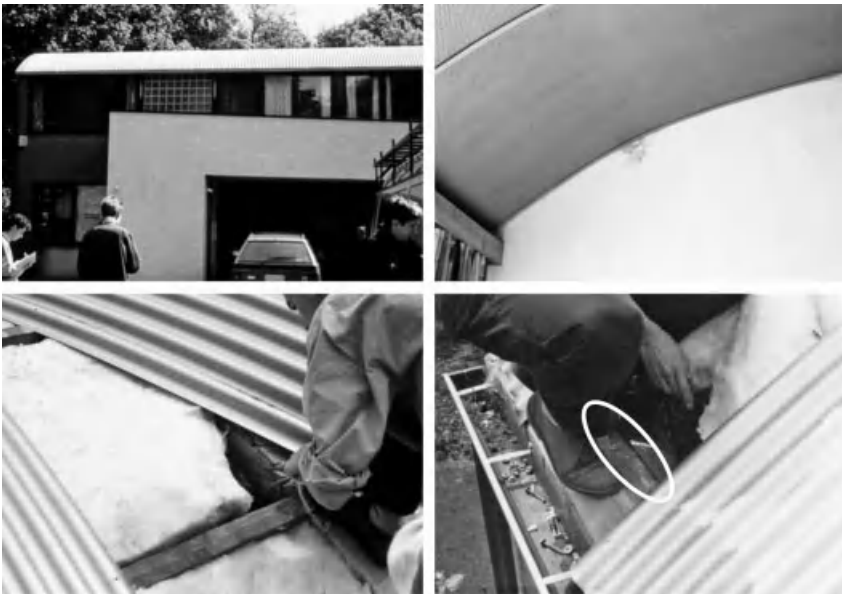
Figure 7.11. Dwelling. Up on the left a view of the metal roof, up on the right traces of moisture leakage, down on the left opening the roof, down on the right leaky vapour retarder along the perimeter.
