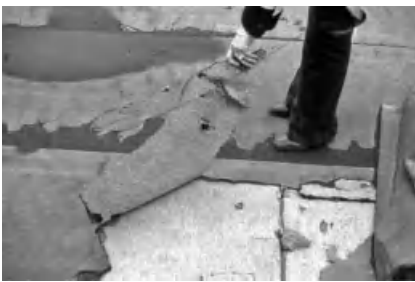
Figure 5.11. Lightweight roof, membrane torn off during a wind storm.
