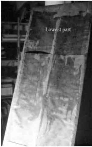
Figure 6.27. Cathedralized ceiling assembly 4, condensation on the underlay. Largest deposit at the lowest part of the underlay.
