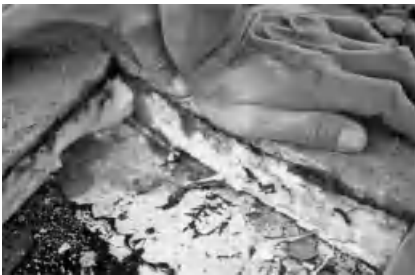
Figure 5.25. Heavy deck roof without vapour retarder above an indoor climate class 5 building, interstitial condensation in the PUR-insulation.
