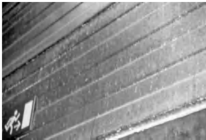
Figure 2.4. Well insulated cellular outer wall without thermal cuts, surface condensation.
