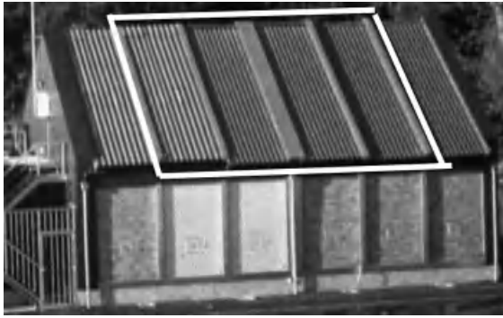
Figure 6.32. Test building used for testing the two times four saddle roofs (the four in the parallelogram).
