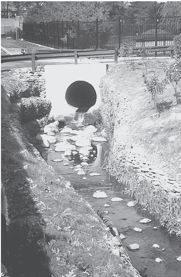
Figure 4.17 Maguire Avenue after installation of gabions, boulders to deflect culvert outflow, and plantings. (Project: New York City Department of Environmental Protection. Photo: Dean Cavallaro.)
