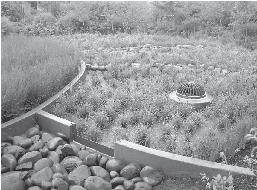
Figure 5.9 This bioswale, part of Glencoe School's green street in Portland OR, uses check dams, a “flash-board” level-setting device in the weir, and overflow drain to treat and infiltrate stormwater. (Project: Portland Bureau of Environmental Services. Photo: Kevin Robert Perry and Portland Bureau of Environmental Services.)
