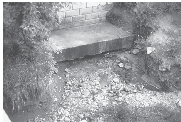
Figure 2.I4 Rigid structures protect only the soil they can shield from water. Along the hard edges, erosive undercutting is actually increased. (Photo: Kim Sorvig.)
