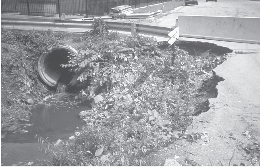
Figure 4.16 Erosion undercut pavement at Maguire Avenue and prevented plants from re-establishing. (Project: New York City Department of Environmental Protection. Photo: Dean Cavallaro.)
