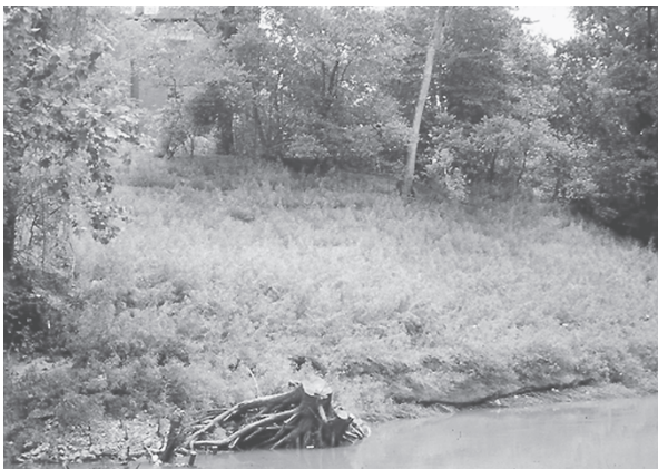
Figure 3.6a–c BTEC techniques form a flexible toolkit, often used in combination, as in stabilizing this bank at Crestwood (Houston TX). Note the large stump, left as added protection, visible in the before, during, and after photos. (Project and Photo: Robbin B. Sotir.)
