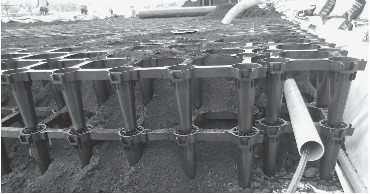
Figure 3.27 “Pits” are created by leaving out cells; the whole trench is backfilled after placing trees, and pavers rest atop the cells. Rectangular Strata Vault system is shown; Silva Cells are similarly shaped. Roots (and utilities) pass easily through such support structures. (Project and Photo: Citygreen.)
