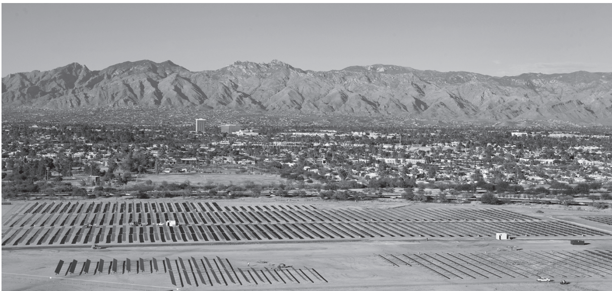
Figure 7.2 PV panels cover 170 acres at Davis-Monthan Air Force Base, Tucson AZ, the largest Department of Defense solar installation. The US military is transitioning to alternative energy far faster than are US politicians. Siting a huge “energy farm” next to a dense user community is the only time such vast centralized features make sense—and in most places, it would likely be opposed by the adjacent residents. (US Air Force photo: 1st Lt. Sarah Ruckriegle.)
