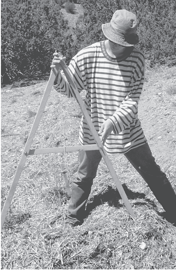
Figure I.7 The Egyptian A-frame is a simple, site-friendly way of establishing level and the fastest way to lay out points along a contour line. (Photo: Kim Sorvig.)
