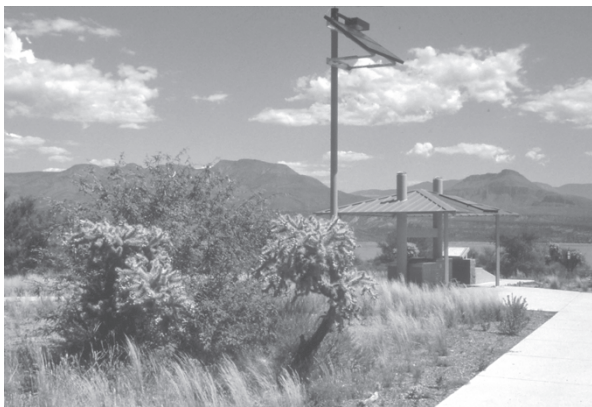
Figure 7.9 Solar electricity for lights and other uses saved hundreds of thousands of dollars in utility installation at Cholla Campground, near Phoenix. Operating costs are near zero. (Project: USFS. Photo: Kim Vander Hoek.)
