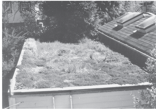
Figure 3.21 Even small-scale ecoroofs decrease runoff, support habitat, and clean the air. Tom Liptan replaced his conventional garage roof with this one. (Project and Photo: Tom Liptan.)
