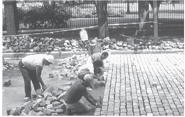
Figure 5.14 Traditional granite setts being laid on sand in Philadelphia’s historic district. Joints are somewhat permeable if not mortared. (Photo: Kim Sorvig.)
