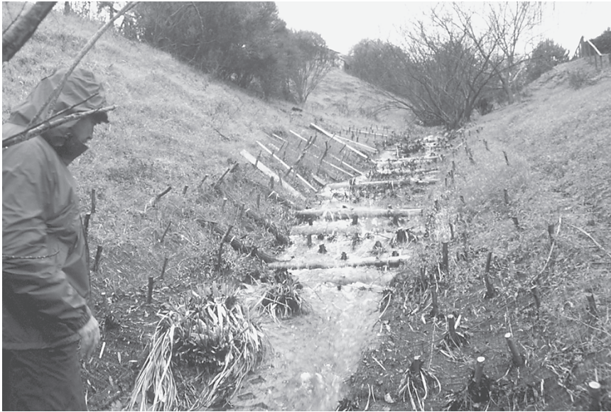
Figure 3.5 Fabric anchored with logs, live stakes, and fast-sprouting grass, in place only a few weeks when this storm struck, survived with no losses. (Project and Photo: Andrea Lucas.)
