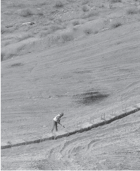
Figure 4.5 Straw bales pinned to the ground provide temporary control of erosion and sedimentation. (Photo: New Mexico Department of Mining and Minerals.)
