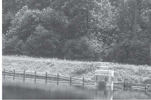
Figure 4.7 The T-shaped opening in this wetland structure sets the water level. Small rises in level flow out through the “trunk” of the T; if major flooding raises the level higher, the top of the T permits faster drainage. (Project and Photo: Rick Scaffidi, EQR.)
