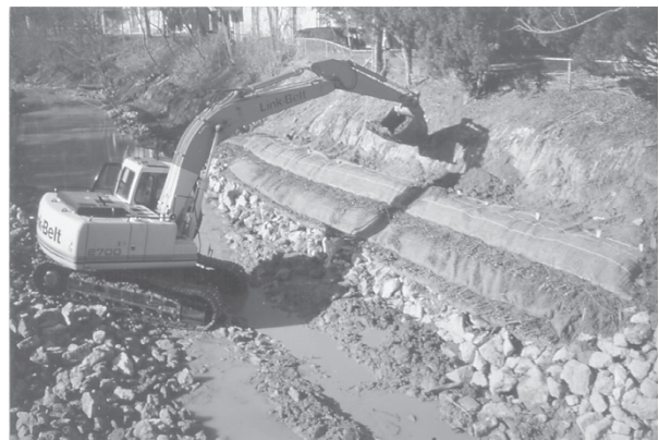
Figure 3.4 Brushlayer installation can be done by hand or aided by equipment. (Project and Photo: Biohabitats Inc.)
