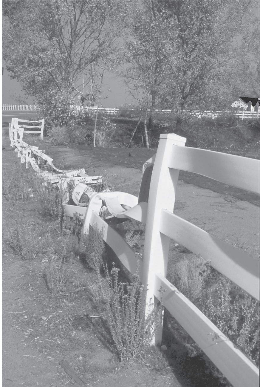
Figure 2.19 In fire-adapted ecosystems, structures must adapt. Plastic fencing melted and the house (right rear) narrowly escaped (San Diego area). (Photo: Kim Sorvig.)
