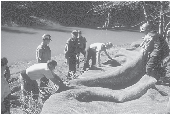
Figure 3.2 Lakeshore stabilization at Whiskeytown CA. Soil wraps are being constructed on top of brushlayers. (Project: Salix Applied Earthcare. Photo: John McCullah.)
