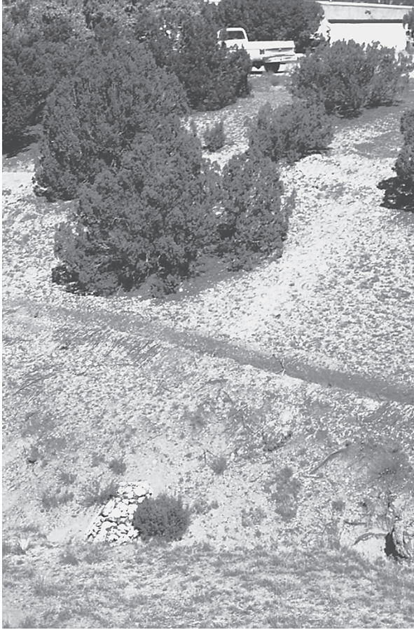
Figure 4.3 Contour-line infiltration trenches, plus check dams in the gully at bottom, stop erosion and raise soil moisture in this Permaculture project in arid New Mexico. (Project: Arina Pittman. Photo: Kim Sorvig.)
