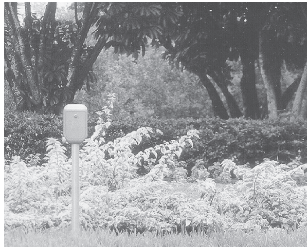
Figure 4.29 Small, solar powered, and radio controlled, LEIT irrigation controllers were among the first to save electricity as well as fuel used in site visits. (Photo: Altec Co. [now DIG Corp.] )
