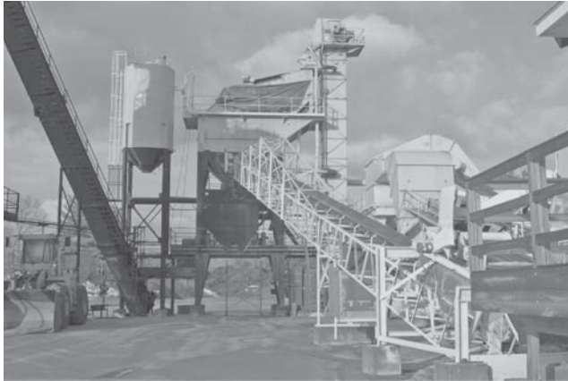
FIGURE 16.1 Hot mix asphalt plant. (Courtesy of Matthew Teto, All States Asphalt, Sunderland, MA.)
