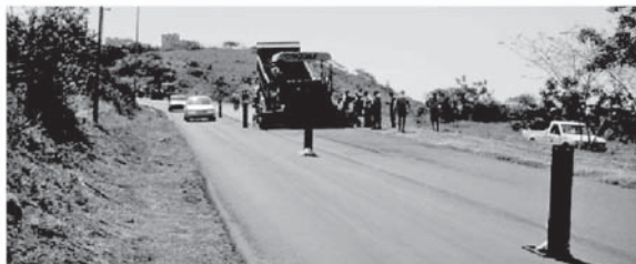
Paving the second lane: First lane opened to traffic immediately after compaction
