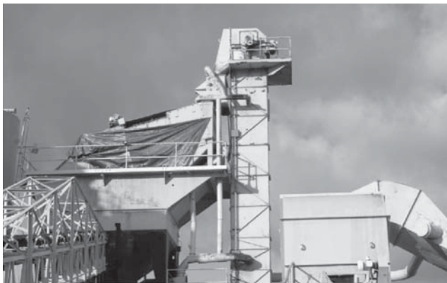
FIGURE 16.5 Hot elevator. (Courtesy of Matthew Teto, All States Asphalt, Sunderland, MA.)
