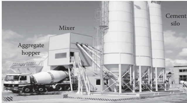
FIGURE 17.1 Concrete plant with mixer, aggregate hopper, and cement silos. (Courtesy of Kim Franklin, Northeast Cement Shippers Association, Castleton, NY.)
