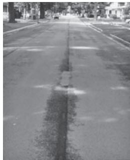
Longitudinal crack at joint
