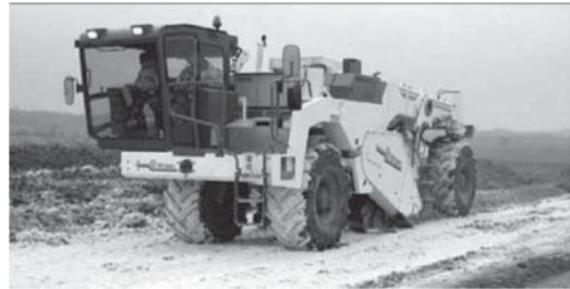
Lime stabilization with Wirtgen WR 2000 Working width: 6 ft 7 in., Working depth: 0–20 in. Engine output: 400 HP, Weight: 49,060 lb
