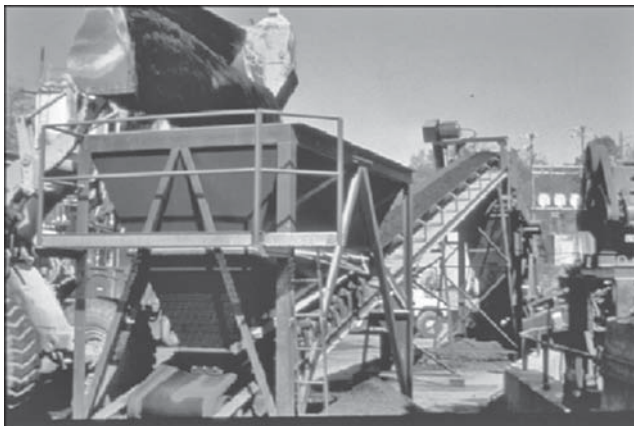
FIGURE 18.15 Reclaimed asphalt pavement (RAP) feeder in a batch plant.
