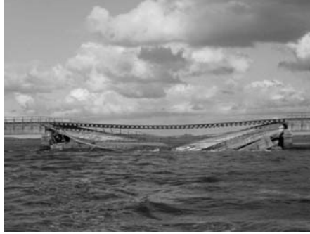
Figure 1.3: Collapse of railway bridge in Malahide, Dublin, Ireland in August 2009, Photo Courtesy Sarah McAllister
