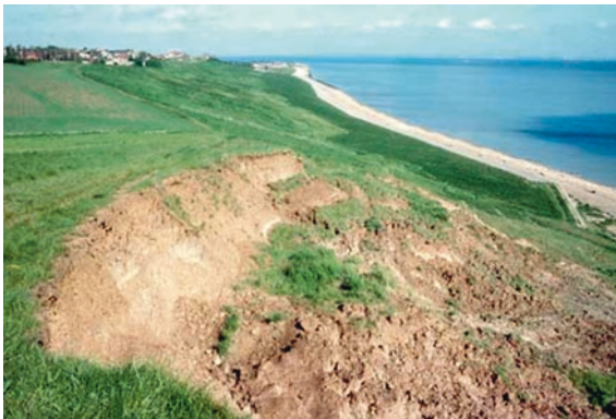
Fig. 7.4 A slumping clay cliff on the north coast of the Isle of Sheppey, Kent, has been largely stabilised, but there is still local erosion. © Geostudies
