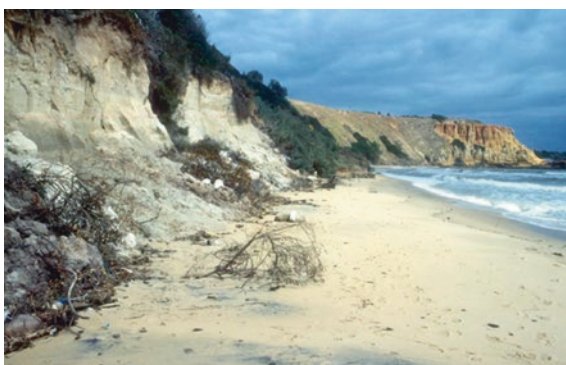
Fig. 2.45 Erosion at the base of the bluff at Sandringham, Victoria, Australia, has followed depletion of the bordering beach. © Geostudies
