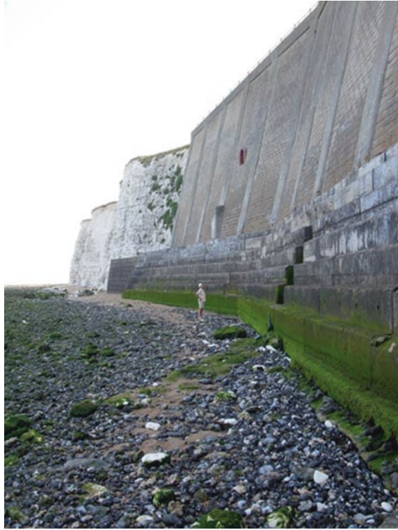
Fig. 7.5 Recession of a sector of Chalk cliff on the Isle of Thanet, Kent, halted by concrete walling. © Geostudies
