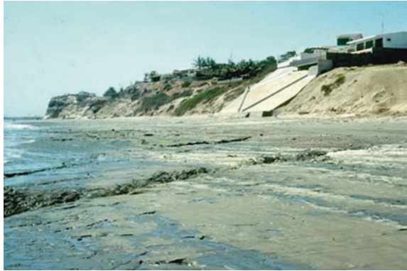
Fig. 7.6 Artificial concrete slope fronting a house on the coast of Ecuador. Erosion continues on adjacent sectors of sloping clay cliff. © Geostudies
