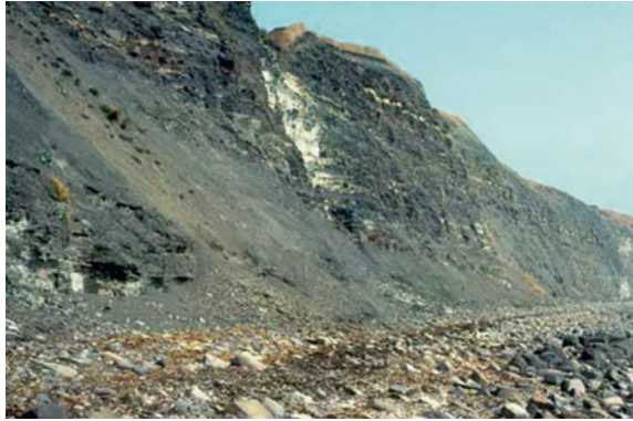
Fig. 3.17 Desiccation caused weathering of clay on cliffs at Kimmeridge in Dorset during a dry summer. © Geostudies
