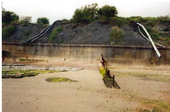
Fig. 3.16 Drainage pipes inserted in the 1980s to evacuate groundwater from Church Cliff at Lyme Regis, Dorset. © Geostudies
