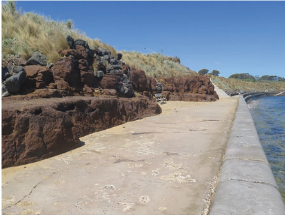
Fig. 7.1 Sea wall protecting a cliff at Black Rock, Port Phillip Bay, Australia. © Geostudies
