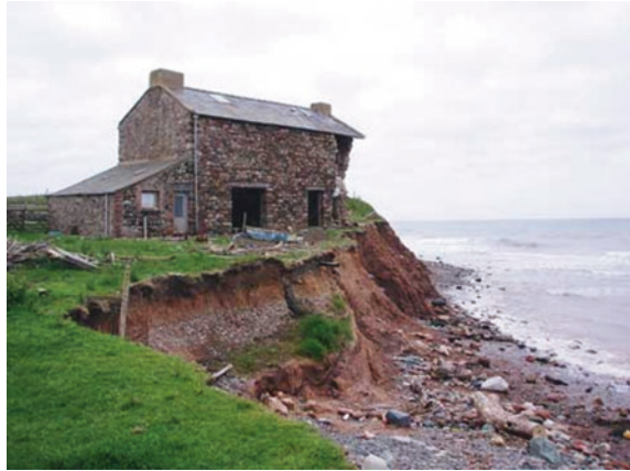
Fig. 1.1 Cliff recession becomes a problem when it results in the undermining and destruction of buildings, as in this example on the Cumbrian coast in NW England. © Geostudies
