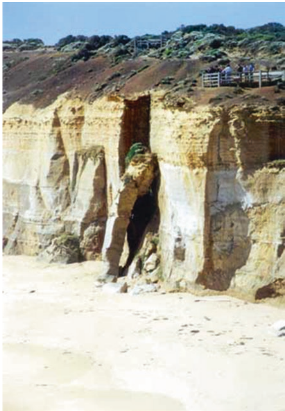
Fig. 3.2 Toppling column on cliff of Miocene siltstone near London Bridge, Victoria, Australia. © Geostudies
