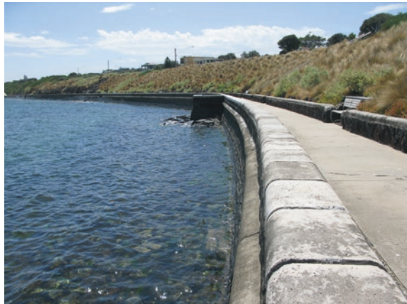
Fig. 7.7 Former vertical cliffs were graded and stabilised behind a sea wall at Black Rock, Port Phillip Bay, Australia, in 1939, but the beach disappeared as the result of wave reflection from the sea wall. © Geostudies
