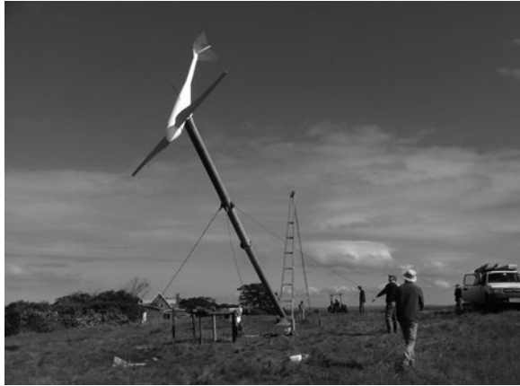
Fig. 7 A 5 kW turbine being raised on a guyed tower using a gin pole. Photo by Ben Fox
