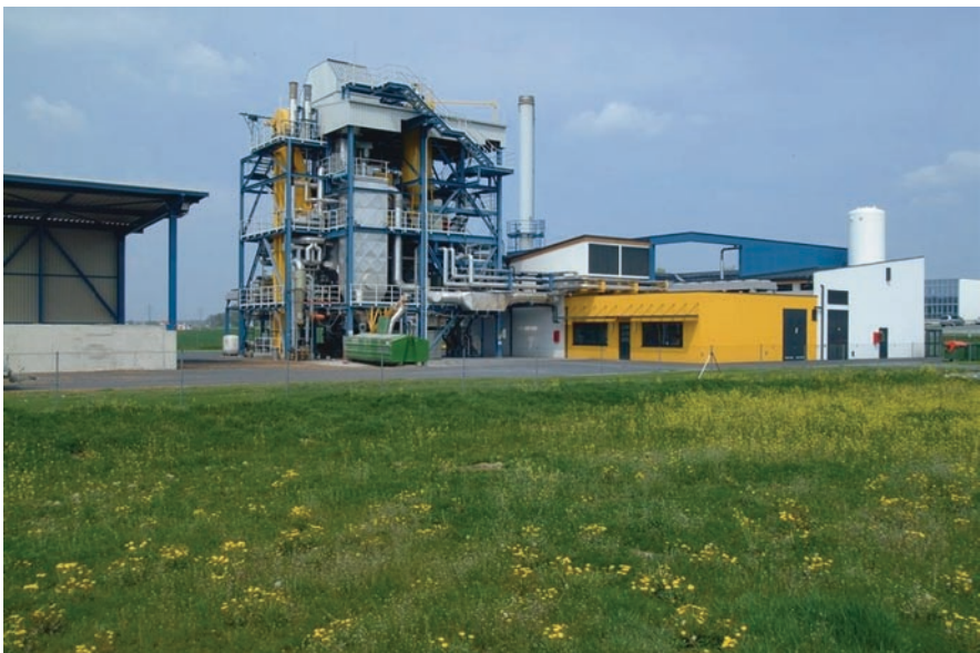
Fig. 6.1.2.1 The first co-generation biomass plant to use direct gasification of wood chips instead of burning the biomass (Courtesy: EEE/RENET)
