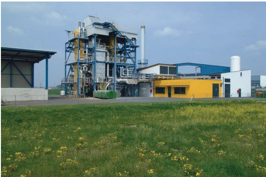
Fig. 6.1.2.1 The first co-generation biomass plant to use direct gasification of wood chips instead of burning the biomass (Courtesy: EEE/RENET) (see Color Plates )
