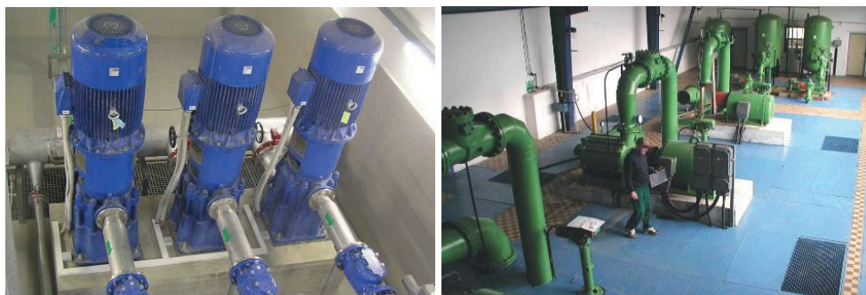
Figure 11. PS Častohostice – old horizontal pumping units (on the left) needed larger space than new vertical pumping units space (on the right). A pumping unit contains three pumps. Each pump is equipped with a frequency converter for smooth power regulation.
