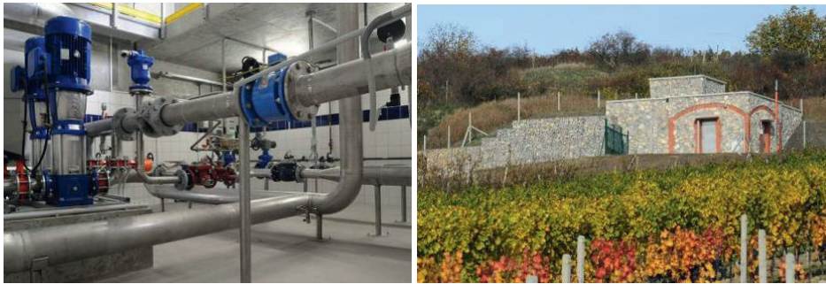
Figure 7. WT Březí – traditional architecture of the wine region – water tank as a wine-cellar.
