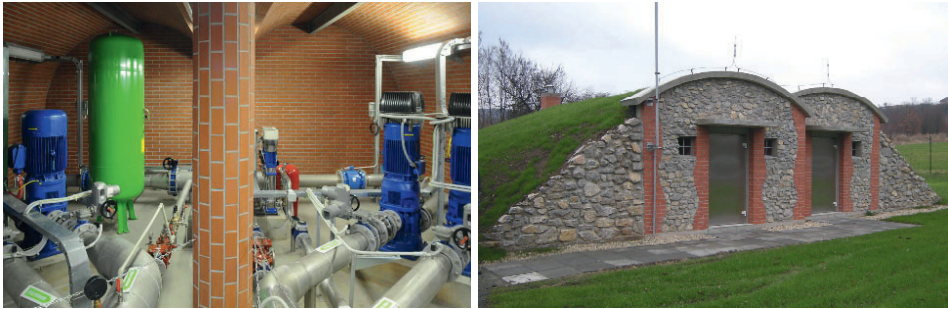
Figure 6. PS Mušlov – traditional architecture of the wine region – pump. station as a wine-cellar.
