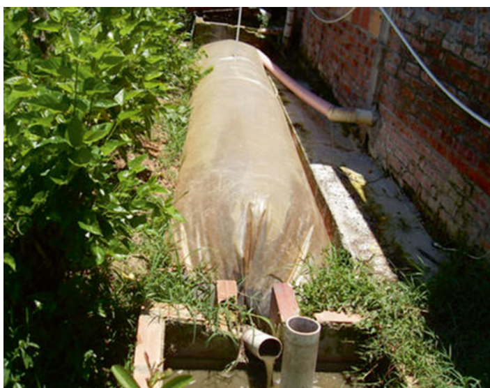
Photo 21 Three biodigesters receive washings from the pig pens and from the family toilets
