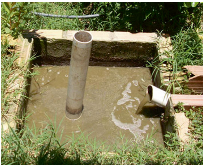
Photo 23 Effluents from all the biodigesters are recycled to the crops and forages as fertilizer
