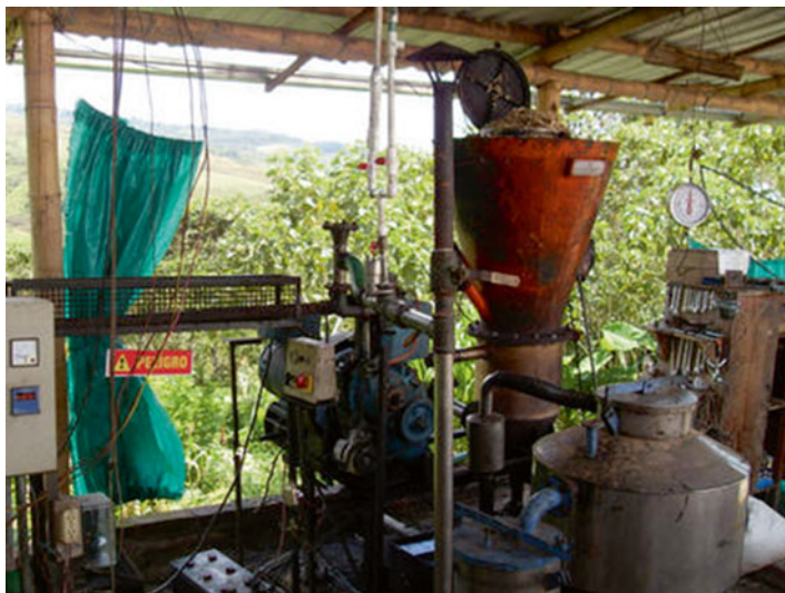
Photo 11 The down-draft gasifier for converting fibrous biomass to electricity
