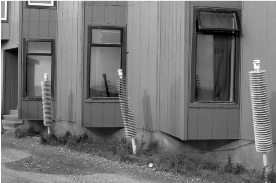
Fig. 10.11 Arctic buildings like the Nullagvik Hotel in Kotzebue, Alaska, must be isolated from permafrost to keep them from melting into the ground. Note the spring-like radiators designed to shed excess heat from beneath the raised foundation, which is separated from direct contact with the ground by pilings (Photo by the author)
